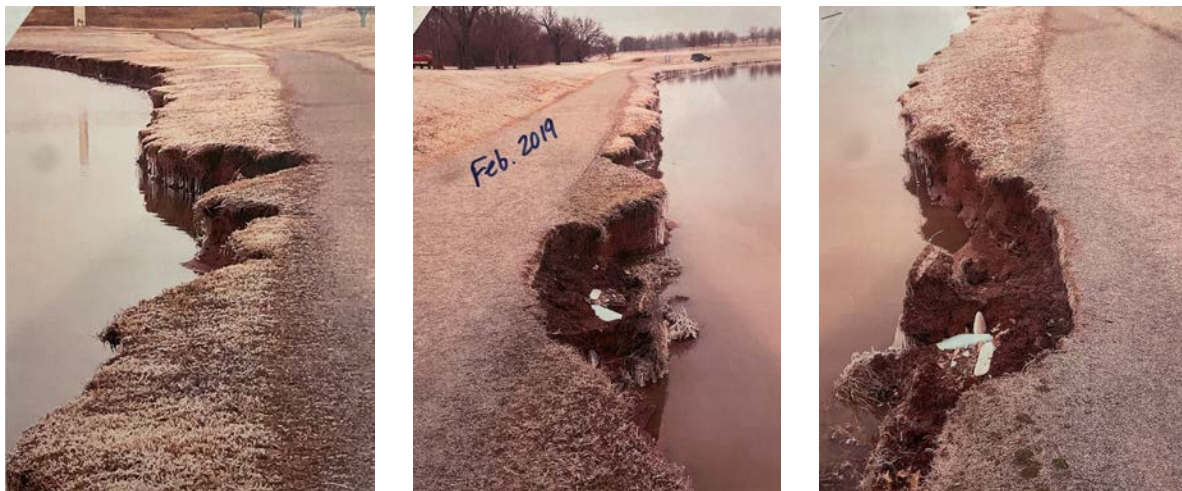
Figure 2: Erosion on pond prior to rip-rap placement. (C-Star, 2019)
