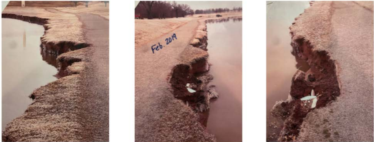
Figure 3. Pond Erosion Prior to Riprap
