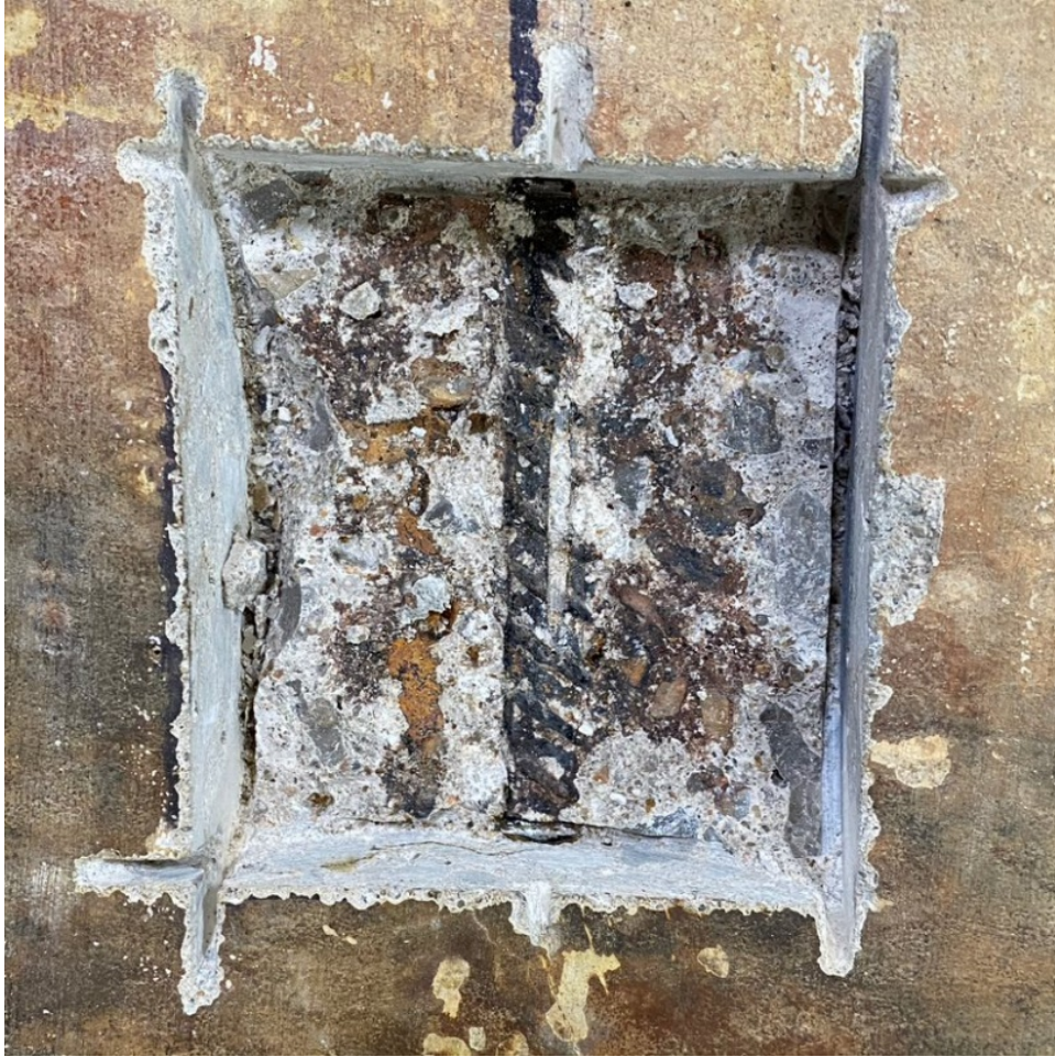
Figure 5-13: CAA-N observed rebar B, 37 days tested
