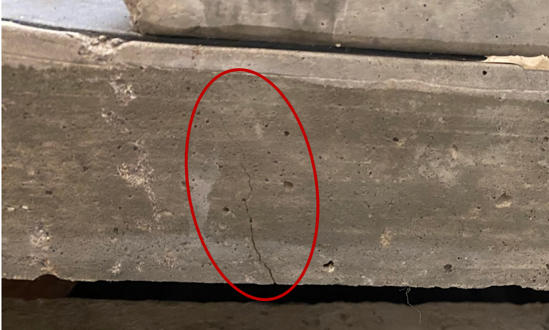
Figure 3-27: Cracking in AA-L during cyclic loading (annotated)
