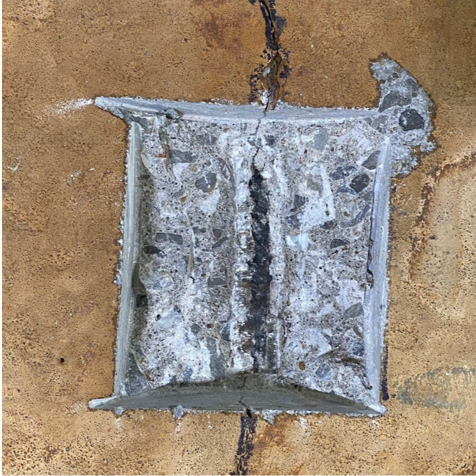
Figure 5-24: CAA-L observed rebar D, 65 days tested
