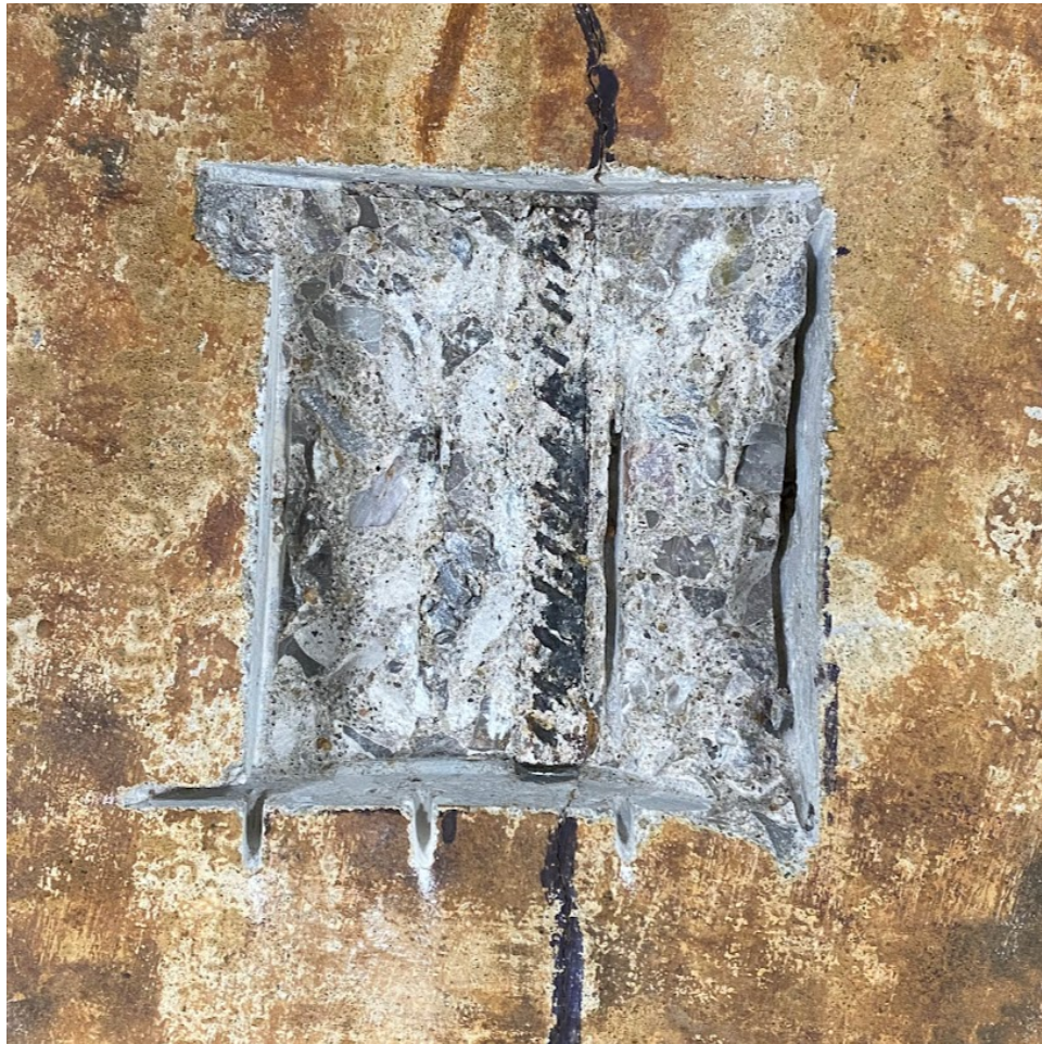
Figure 5-26: CAA-N observed rebar C, 65 days tested
