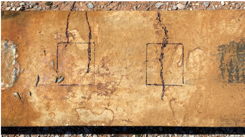
Figure 5-22: Surface of specimen CAA-L after 65 days of corrosion testing
