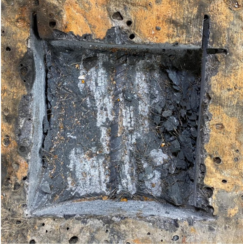
Figure 5-17: CU-L observed rebar B, 37 days tested
