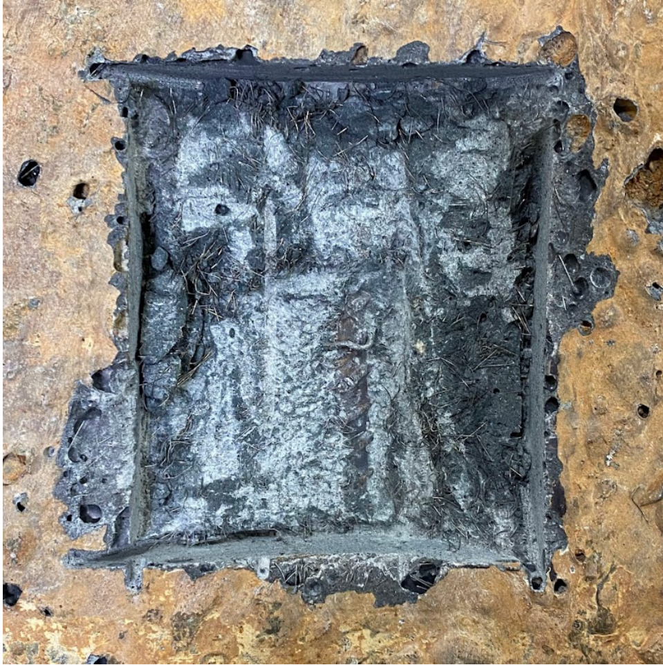
Figure 5-30: CU-L observed rebar D, 65 days tested
