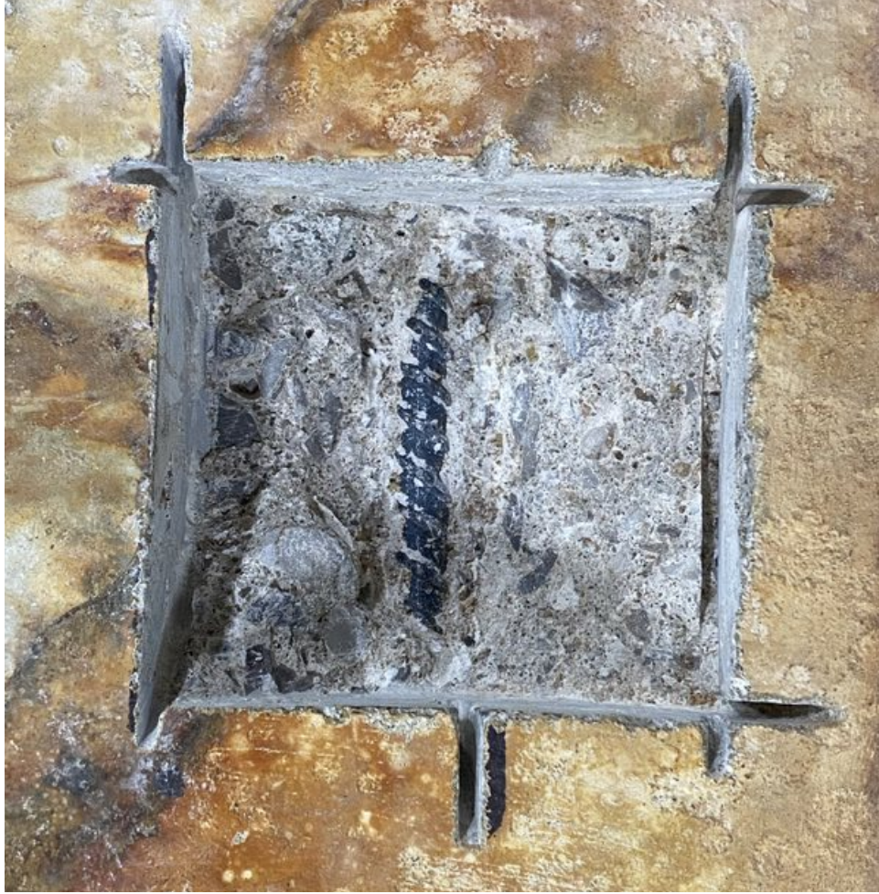
Figure 5-8: CAA-L observed rebar A, 37 days tested
