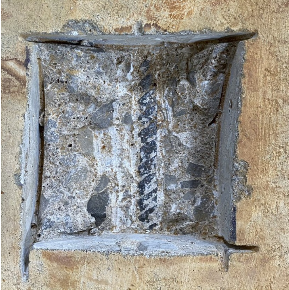
Figure 5-9: CAA-L observed rebar B, 37 days tested
