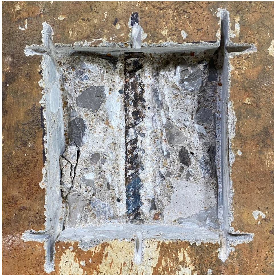
Figure 5-12: CAA-N observed rebar A, 37 days tested
