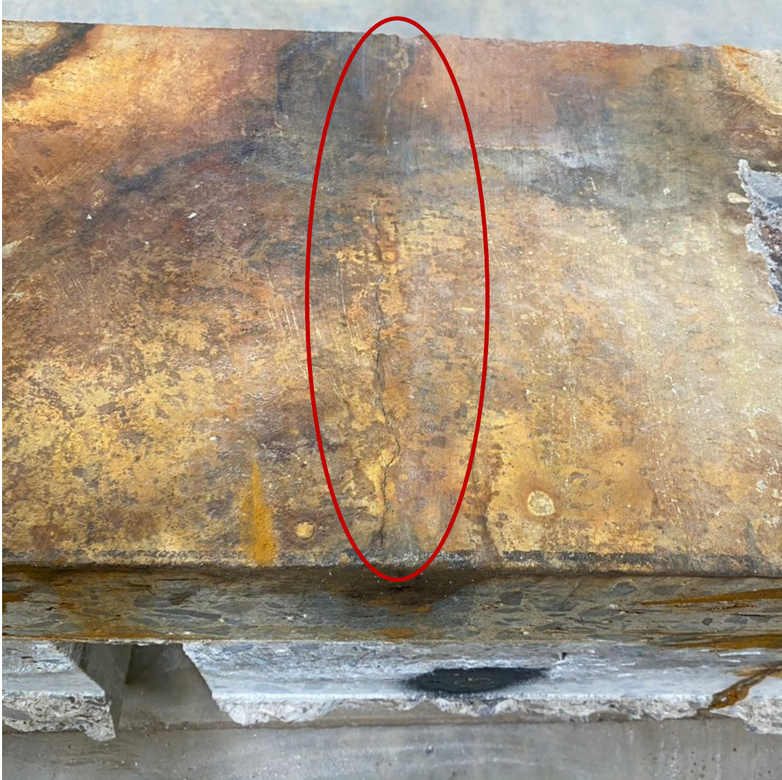
Figure 5-10: Cracking in specimen CAA-L (present prior to testing, annotated)
