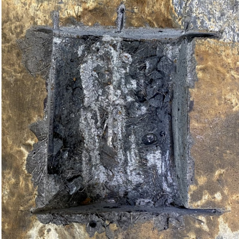
Figure 5-20: CU-N observed rebar B, 37 days tested
