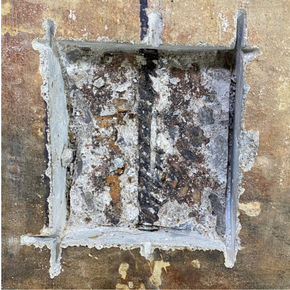
Figure 5-13: CAA-N observed rebar B, 37 days tested
