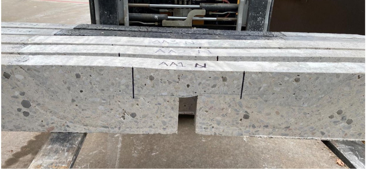
Figure 4-2: Specimen sections with freeze-thaw lengths indicated with marker
