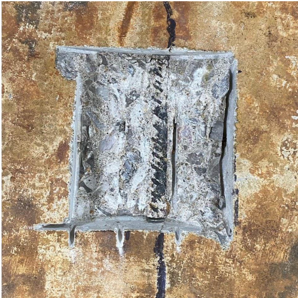
Figure 5-26: CAA-N observed rebar C, 65 days tested
