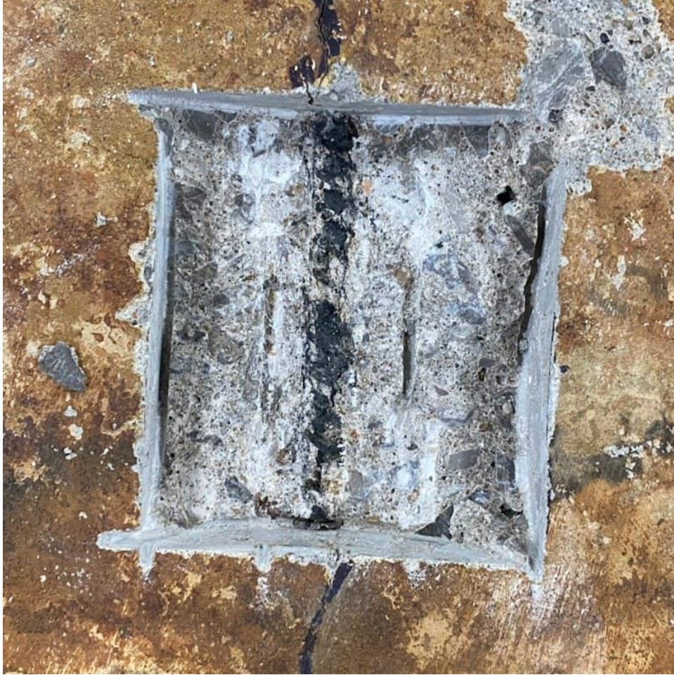
Figure 5-27: CAA-N observed rebar D, 65 days tested
