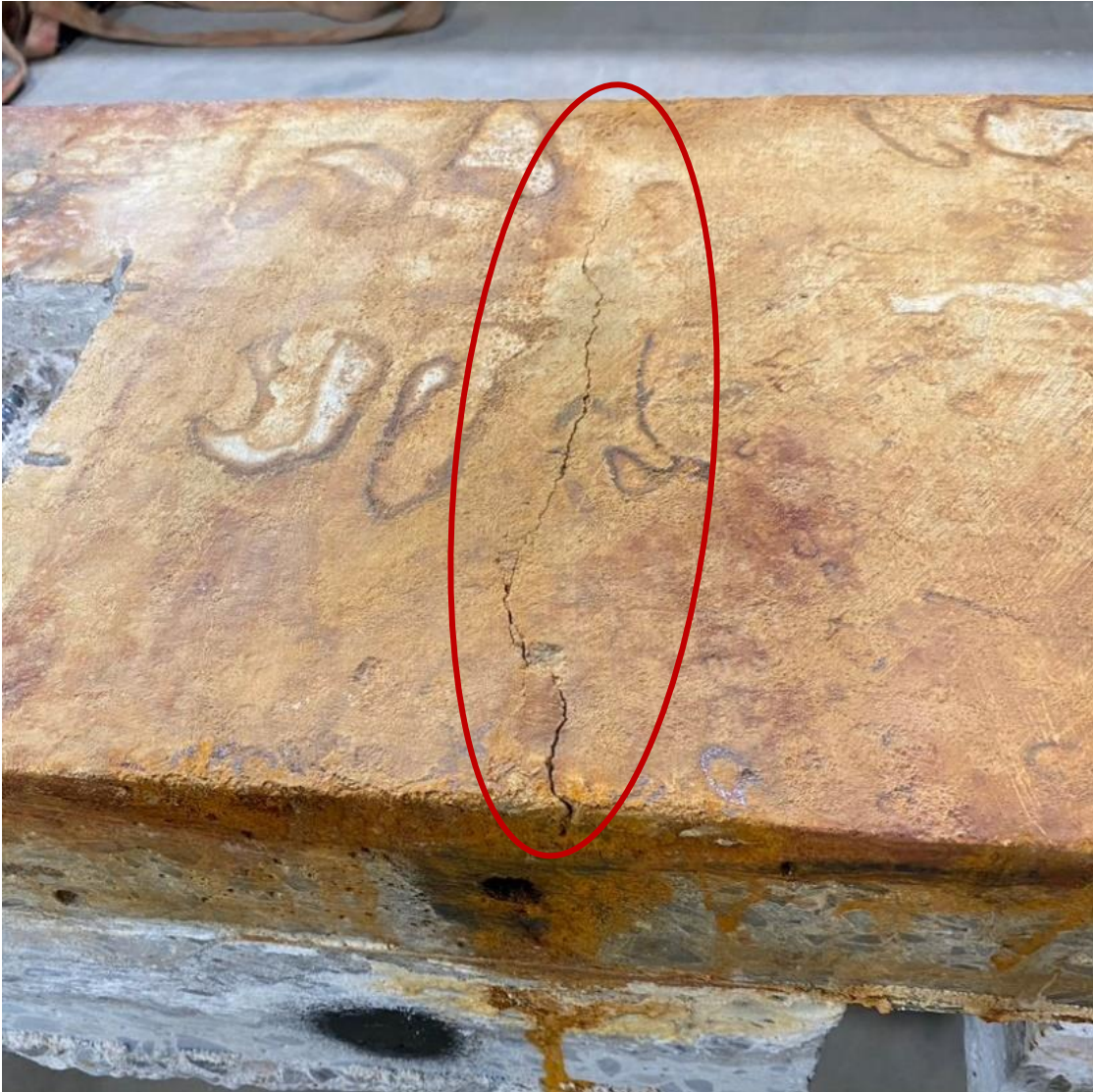
Figure 5-14: Cracking in specimen CAA-N (annotated)
