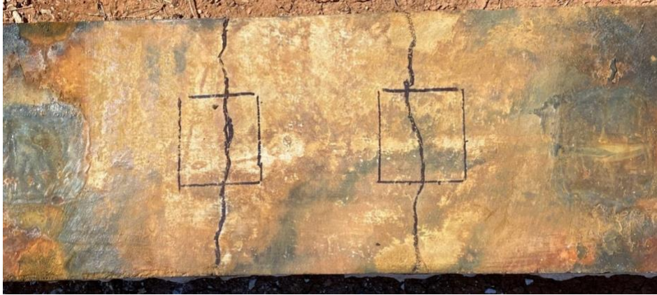
Figure 5-25: Surface of specimen CAA-N after 65 days of corrosion testing
