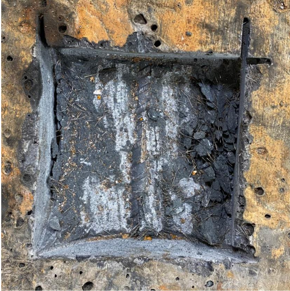
Figure 5-17: CU-L observed rebar B, 37 days tested
