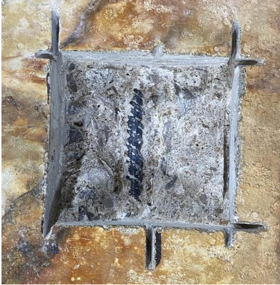
Figure 5-8: CAA-L observed rebar A, 37 days tested
