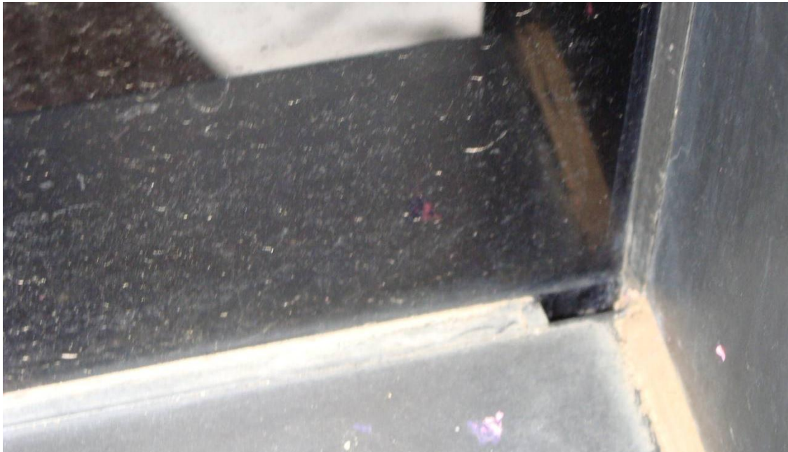
Figure 1: Gap in caulk
