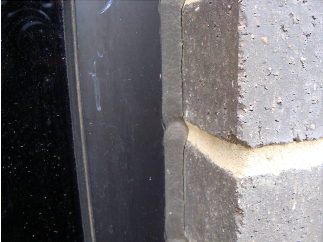
Figure 2: Caulk pulling away from the wall
