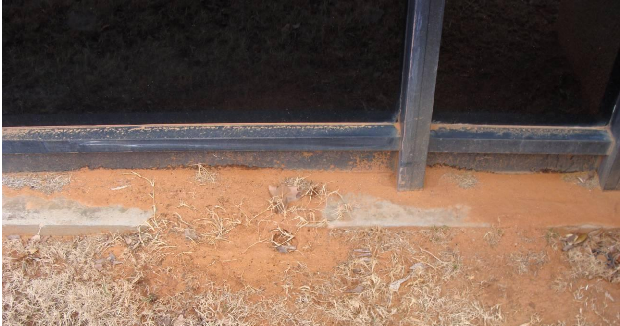
Figure 3: Dirt at the base of ground floor windows
