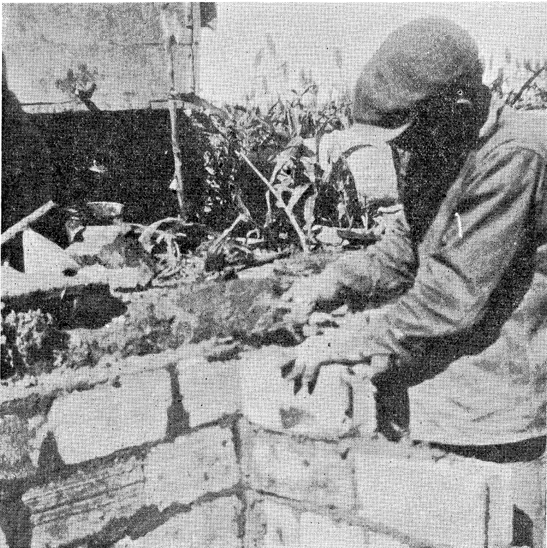
Fig. 6.—Shows a brace wall being laid after the main part of the baffle is completed.
