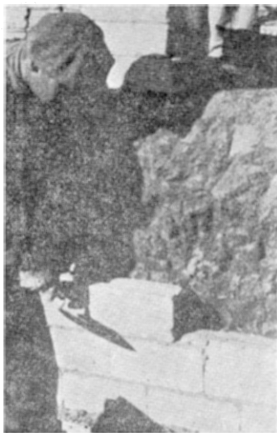
Fig. 5.—Shows the brick being laid in place following the spreading of the mortar. After pressing the brick in place the mortar is cut off with the trowel.
