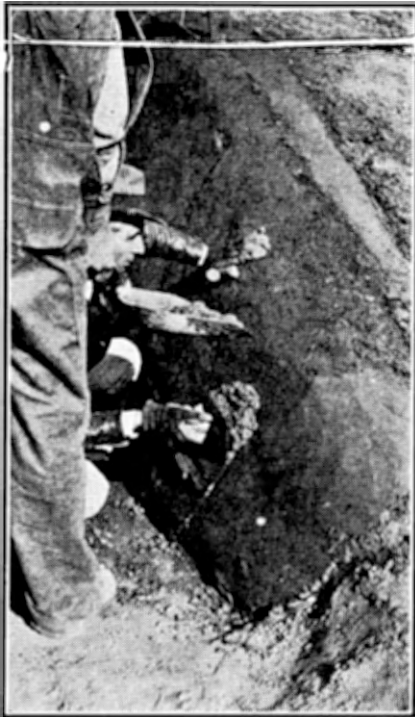
Fig. 4. —The wall is smoothly plastered after the three-inch reinforced wall is built.
