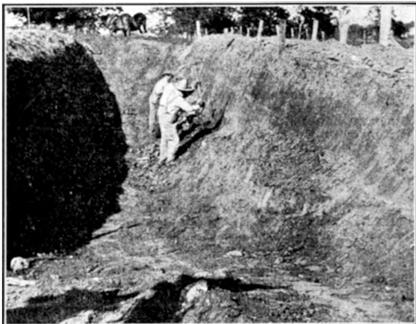
Fig. 2. —Plow and fresno or slip scraper are used to dig the trench; grubbing hoe and spade are used to true up and smooth the sides.
