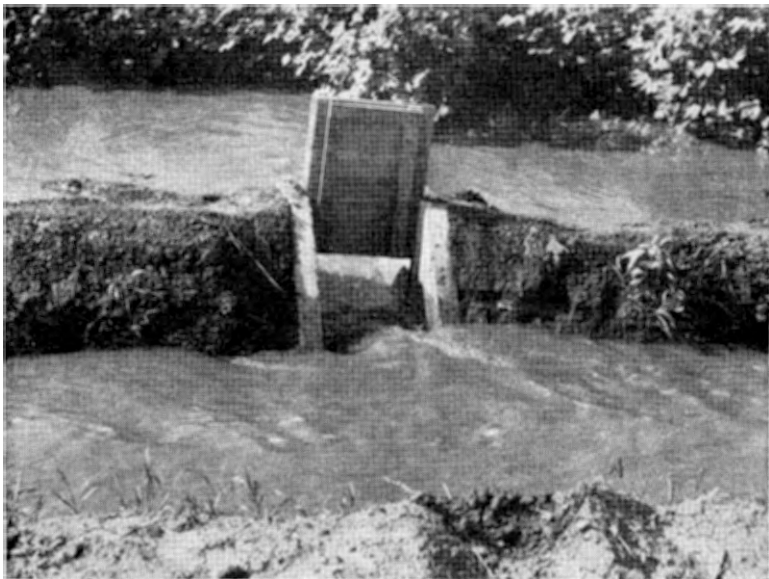
Figure 6. —A turn-out box used to divert water from ditch to field.
