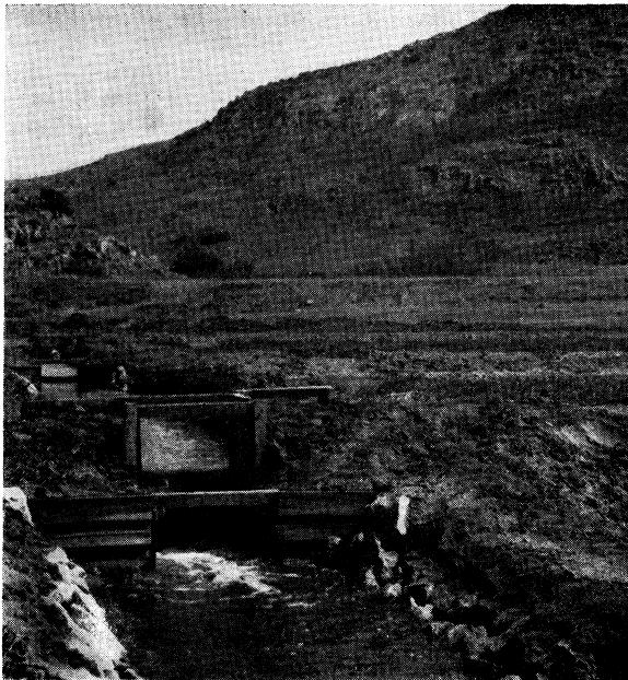
Figure 3.—Semi-permanent drop check structures are used to control the flow of water down a steep slope.
