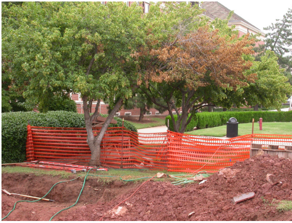
Figure 6.53. Damage to trees from construction and excavation of soil too close to the tree.
