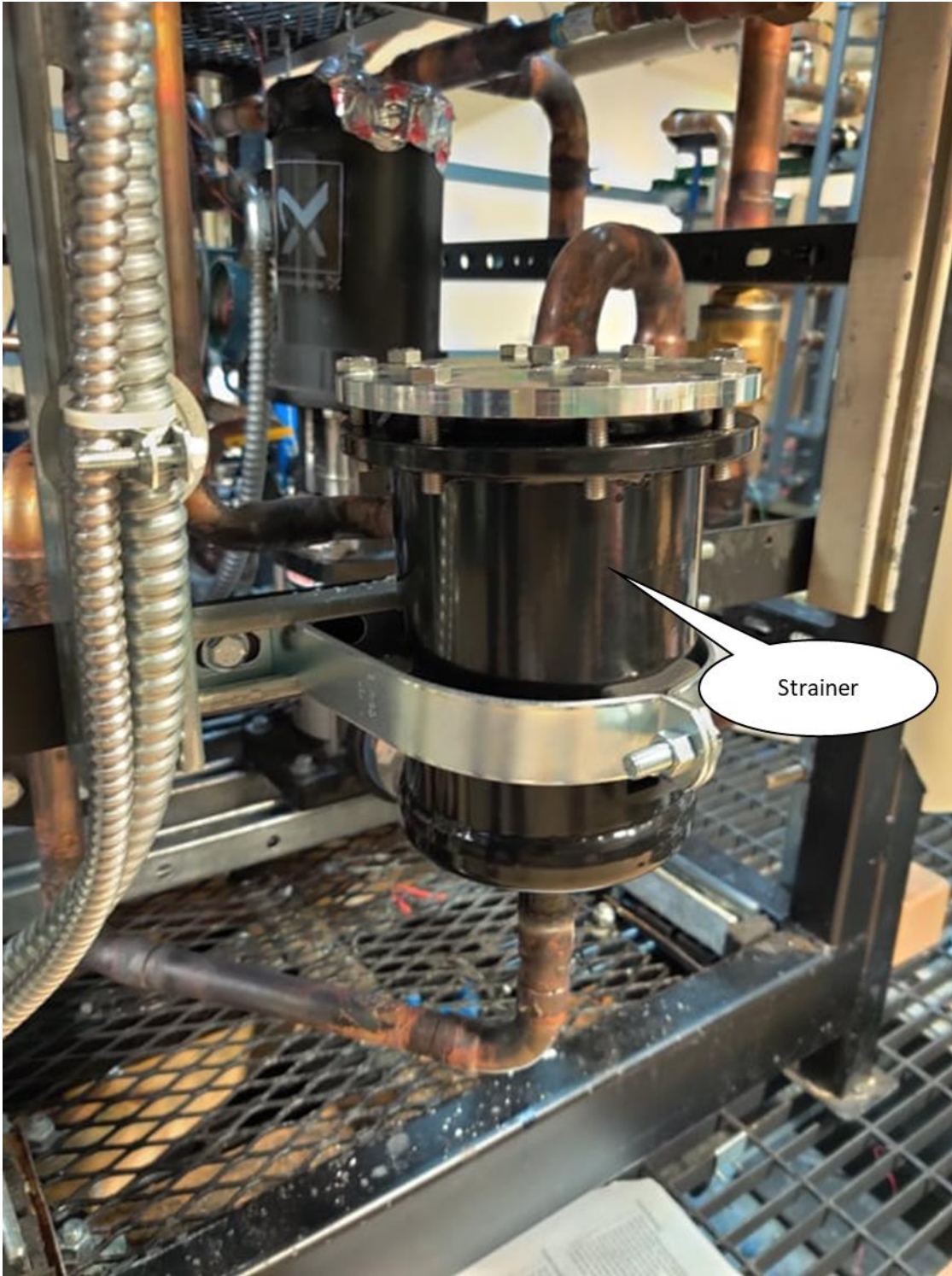
B.12: Refrigerant strainer mounted with clamp on a unistrut.
