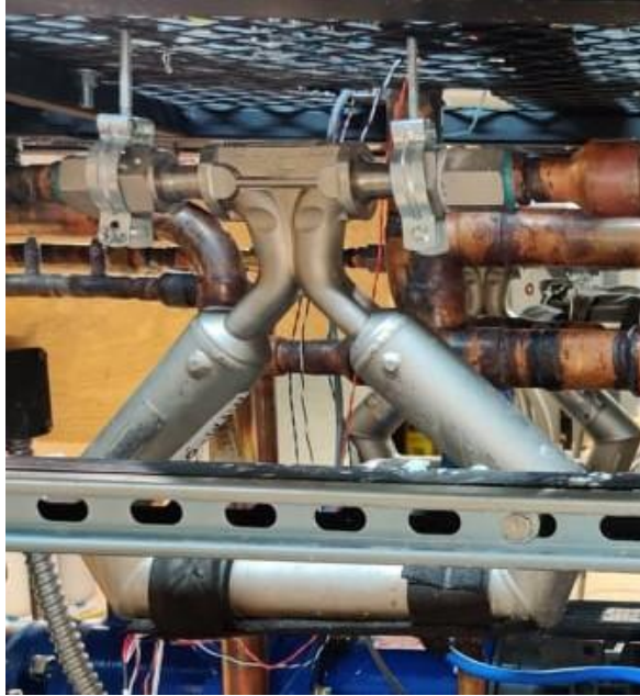
B.13: Refrigerant mass flow meter mounted with clamps.
