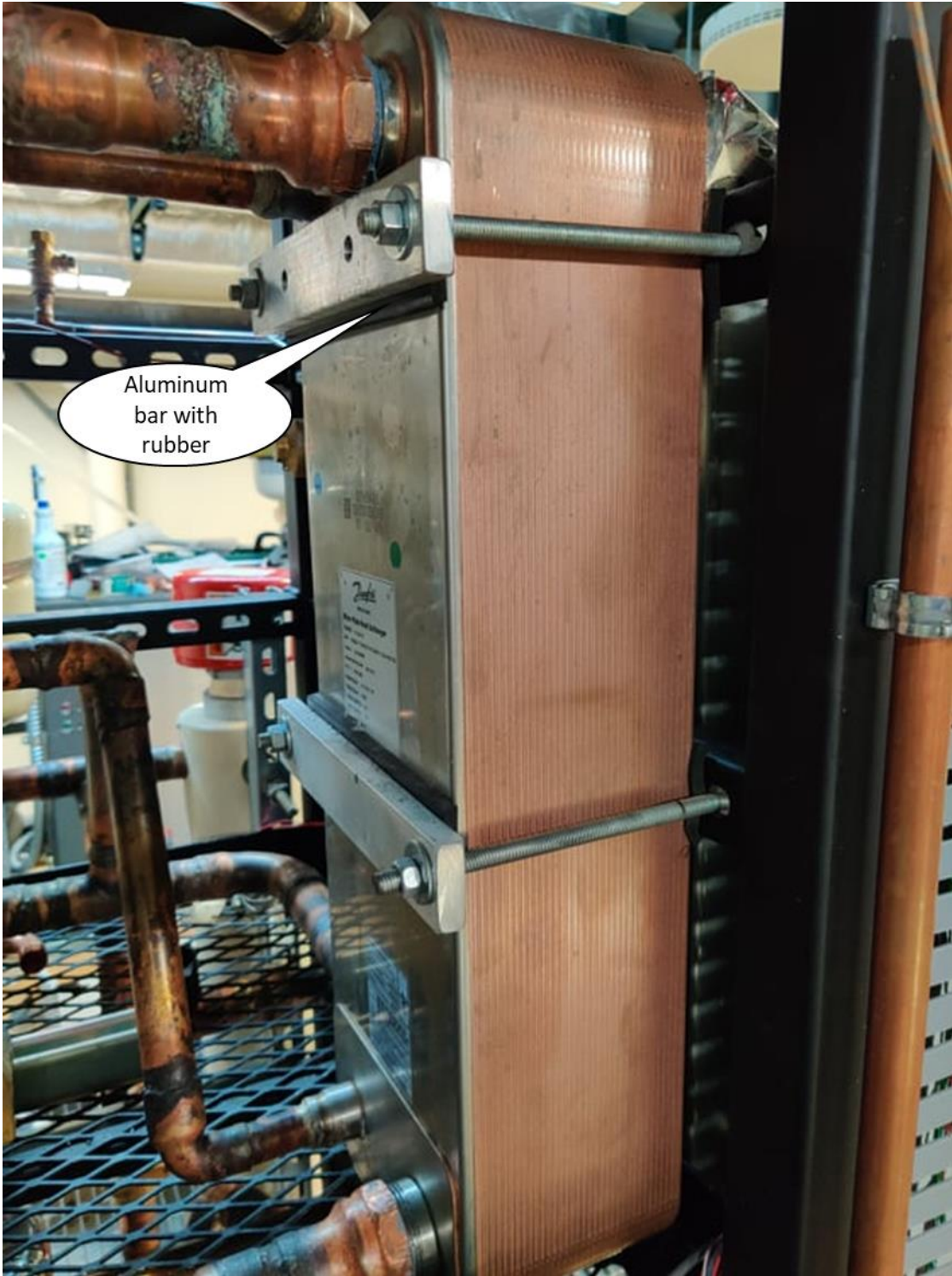
B.9: HX attached to the unistrut of the structure with aluminum bar and rubber on both sides.
