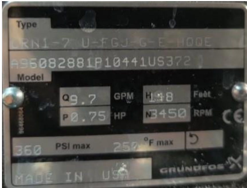
E.4: Glycols pump nameplate.
