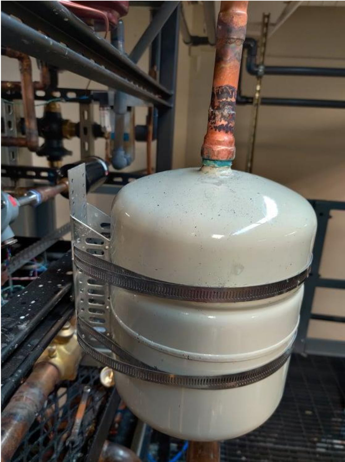
B.15: Glycol expansion tank mounted on the structure with bracket.
