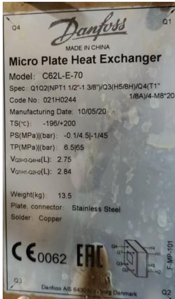
E.9: Pre-evaporator nameplate.
