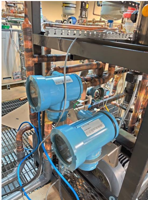
B.14: Transmitters of the mass flow meters mounted on the structure.
