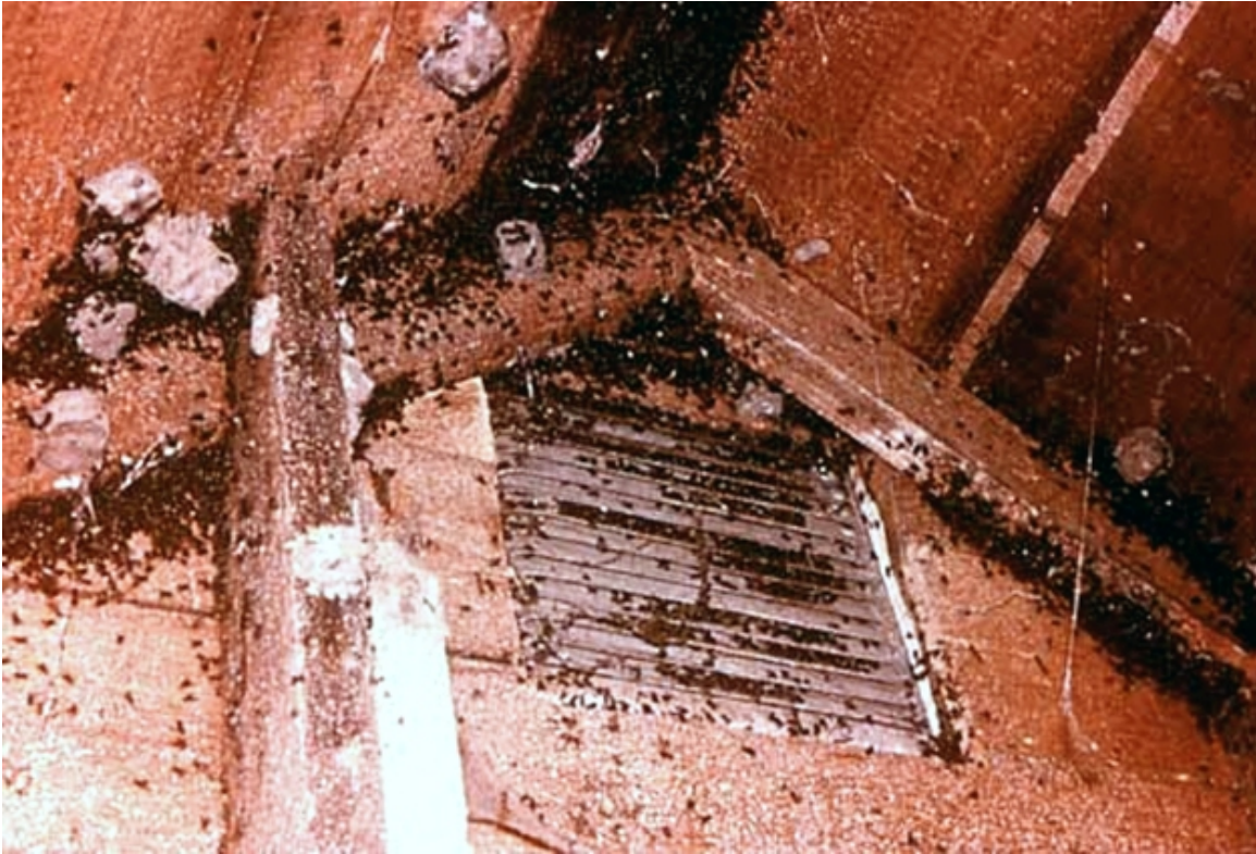
Fig 3. Face fly hibernaculum in an attic of a Nebraska farm house. Photo credit: C. Jones, USDA, ARS.
