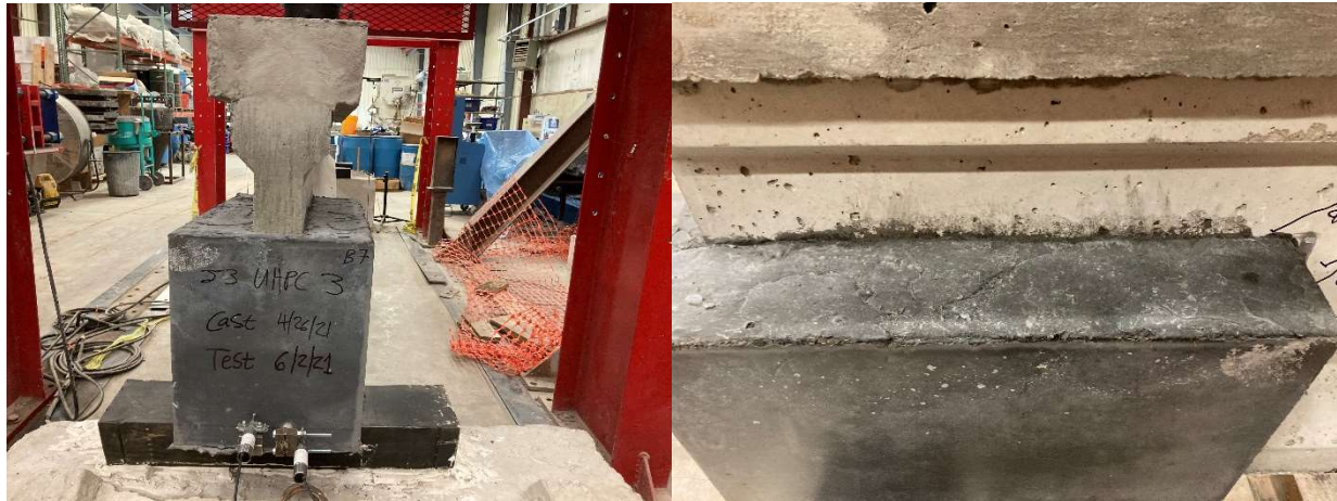
Figure 3.20: Finished UHPC Repaired Region at Front View (Left) and Side View (Right)
