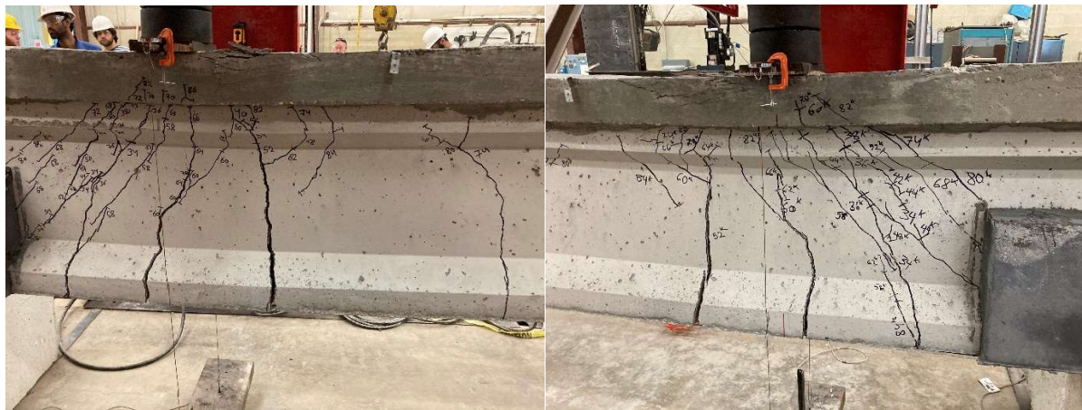
Figure 4.31: UHPC-3 Girder after Test with SE Side (Left) and SW Side (Right)
