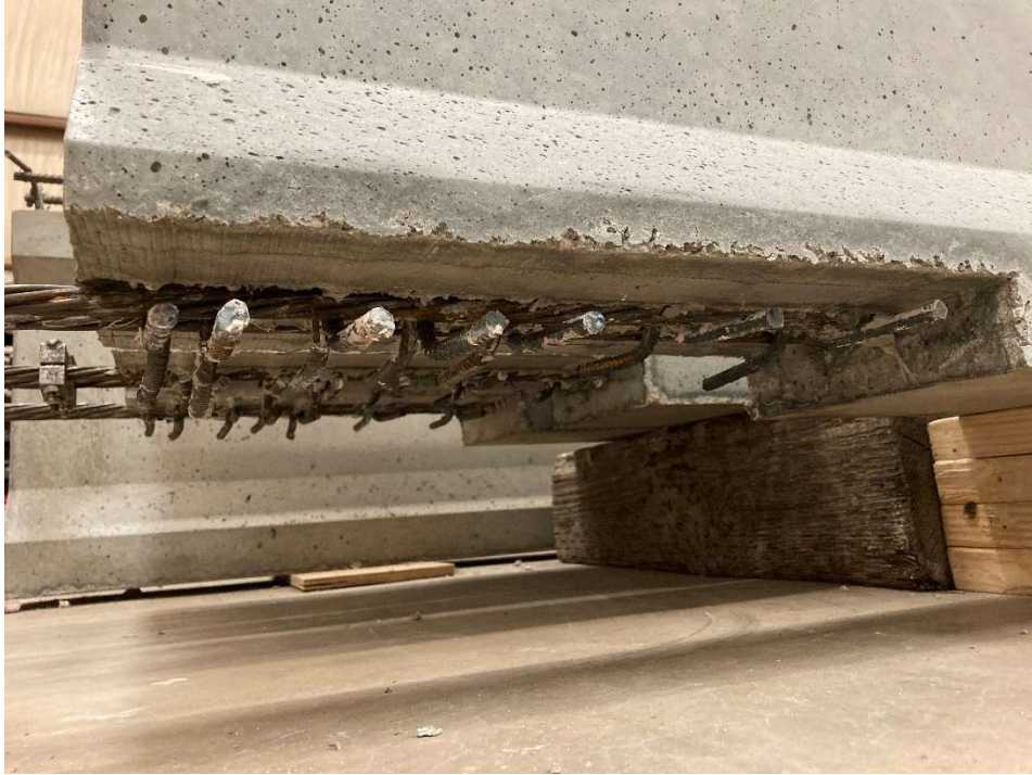
Figure 3.10: The Representative Corroded Region without the Foam
