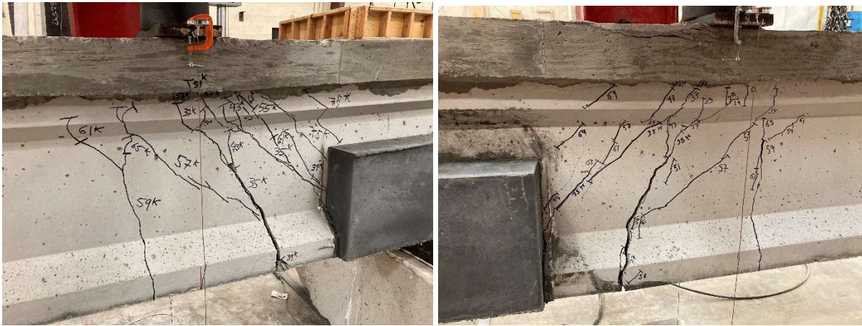
Figure 4.24: UHPC-1 Girder after Test with SW Side (Left) and SE Side (Right)
