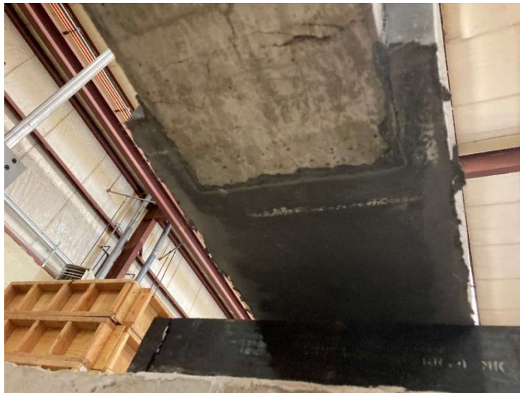
Figure 4.28: Cracks in Bottom Flange of UHPC-2 Girder after Test
