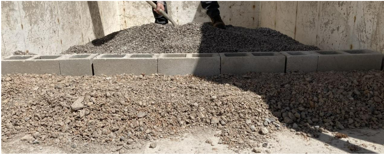
Figure 7 – Sand bed installation and protection; (Top) sand bed installation for GRS Abutment Model #7, (Bottom) aggregate placement for bed protection for GRS Abutment Model #8
