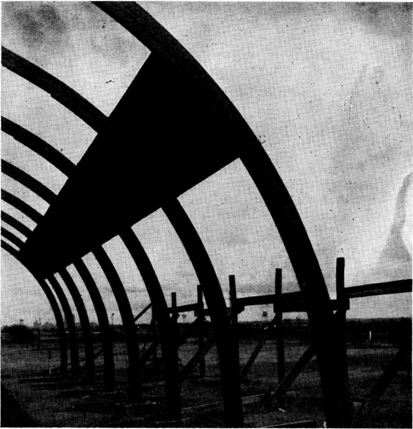
Figure 2. Self-indexing of stressed-skin panels with respect to main frame elements. Panel longitudinal ends fit between main frames.
