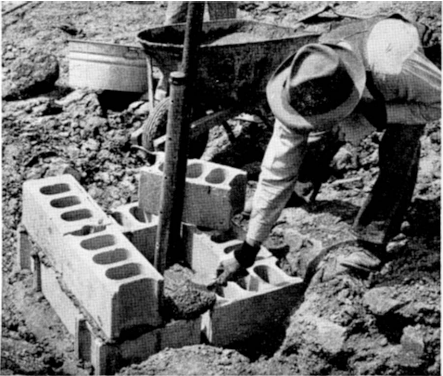
Figure 4.—Construction of intake at pond on dairy farm. The concrete blocks were built up to a level slightly above the top of the perforated and capped intake pipe. The other pipe is not connected; it merely extends above the water surface to aid in checking the level of water in the pond.
