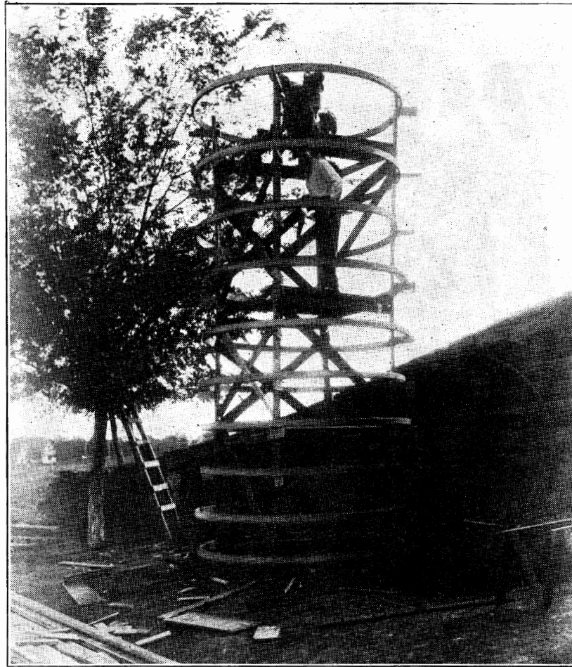
Figure 6—Model wooden-hoop Silo in process of construction. Scaffolding up and hoops in place
