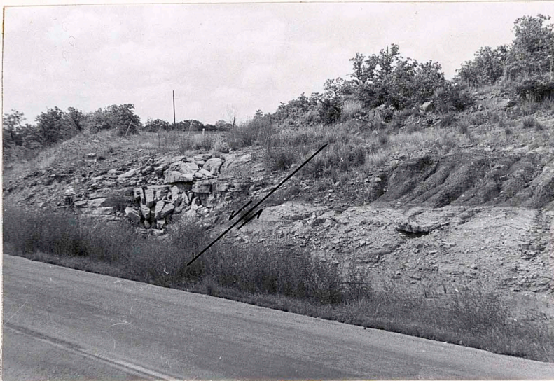
Figure 16. Kiheki sandstone (left and upper right of picture) displaced by small normal fault along Oklahoma State Highway 20, SE \frac{1}{4} sec. 14, T. 22 N., R. 9 E.
