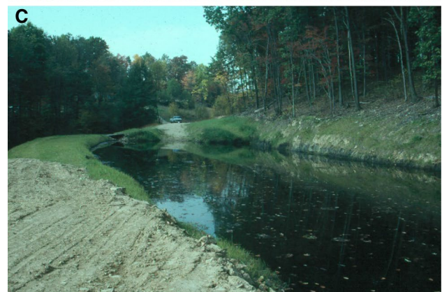
Fig. 6 Construction of an early SAPS in 1995, which has subsequently also been referred to as RAPS, vertical flow ponds, and vertical flow systems. A Initial placement of the limestone base layer with underdrain piping. B Compost layer being placed on top of the limestone. C The system filled with water
