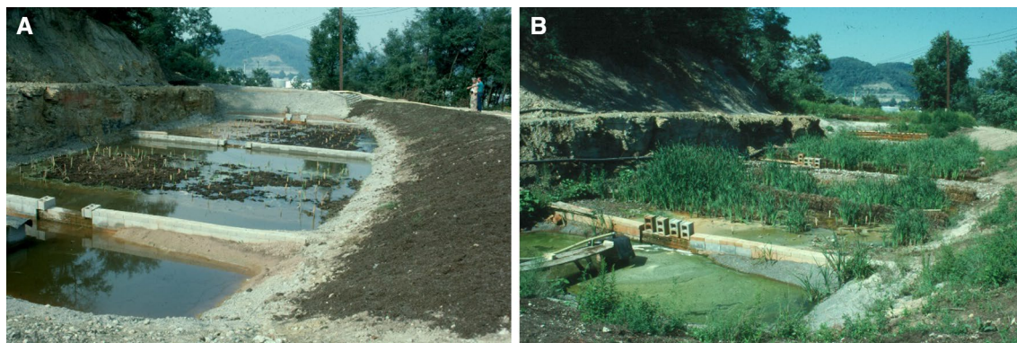
Fig. 3 A A Typha -based wetland immediately after construction in West Virginia. B the same site, two months later
