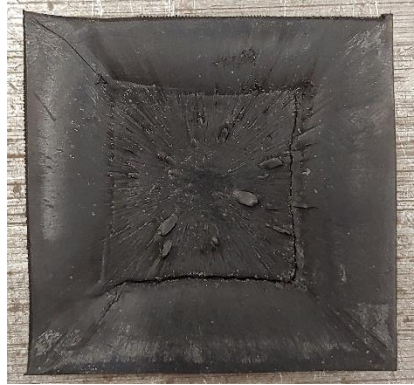
Figure 5.12 – Damaged neoprene pad after excessive expansion
