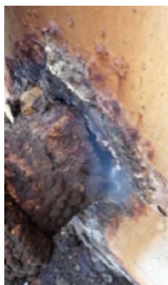
Figure 3 Evidence of Tampering with Monitoring Device
