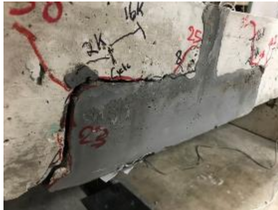
Figure 135. Cracks formed at the conventional concrete to UHPC interface on the north side of J3 slab joint 2
