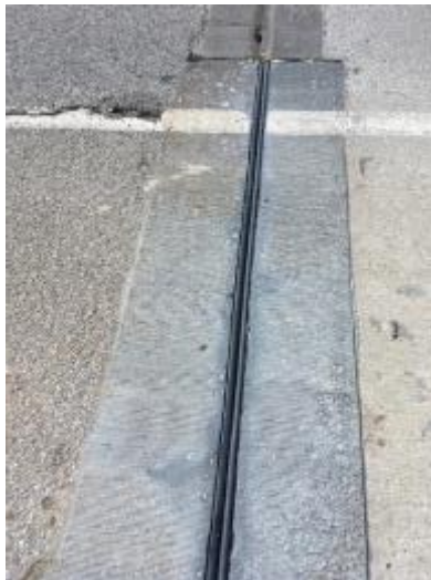
Figure 336. UHPC joint headers on SH-3E bridge immediately after joint sealant was placed
