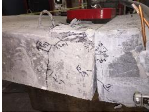
Figure 114. Ductal® slab joint 3 after completion of testing showing concrete crushing and separation at joint indicative of rebar failure
