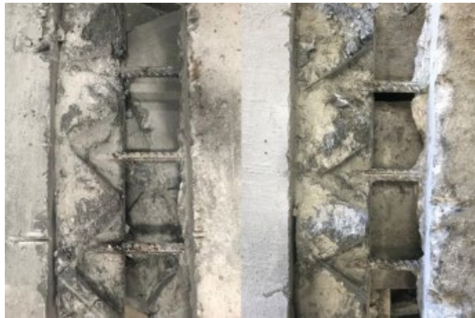
Figure 294. Corrosion state of rebar reinforcing at joint of Ductal® small-scale corrosion specimens with 4% NaCl (left) and 8% NaCl (right)
