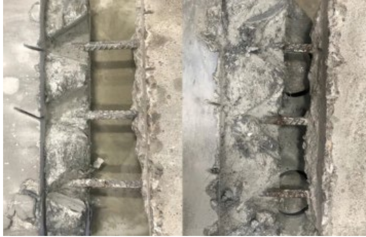
Figure 293. Corrosion state of rebar reinforcing at joint of J3 small-scale corrosion specimens with 4% NaCl (left) and 8% NaCl (right)
