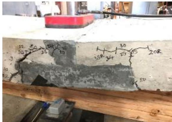
Figure 152. Cracks on the north side of Ductal® slab joint 2 after part 2 testing
