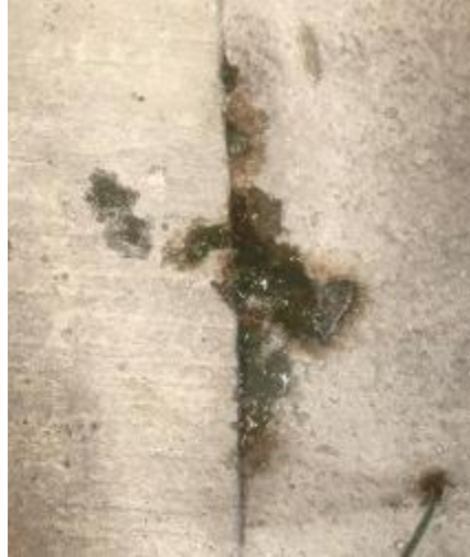
Figure 306. Green liquid in joint of Phoscrete large-scale corrosion specimen during week 7 of testing
