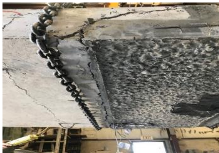
Figure 144. Cracks extending across the entire width of the slab at the joint and in the conventional concrete
