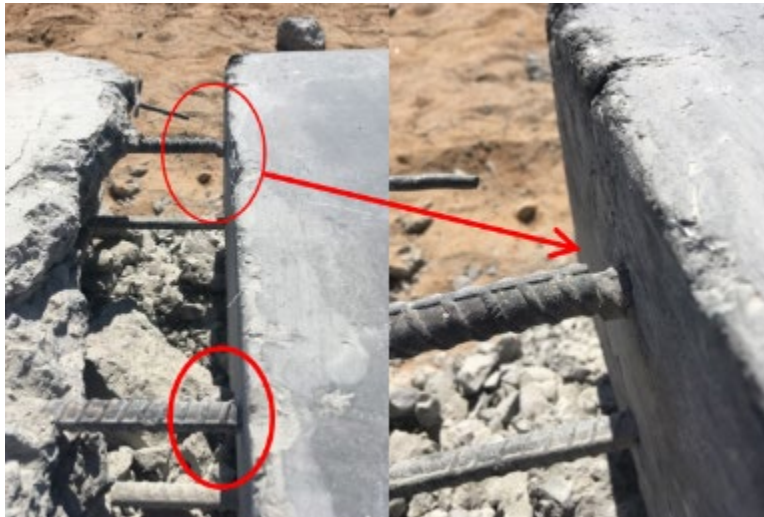
Figure 118. Fractured tension reinforcing bars after fatigue failure of slab joint (note that the slab has been flipped relative to the testing orientation)
