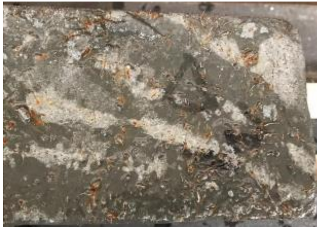
Figure 281. Surface corrosion of Ductal ® freeze-thaw specimen - Cycle 350
