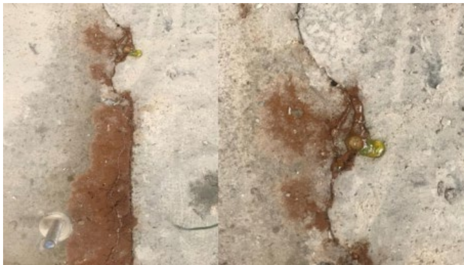
Figure 307. Green liquid in joint of Ductal ® large-scale corrosion specimen during week 8 of testing
