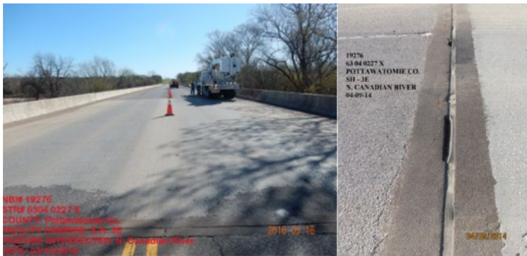
Figure 326. SH-3 bridge over N. Canadian River (left) and expansion joint to be replaced (right)
