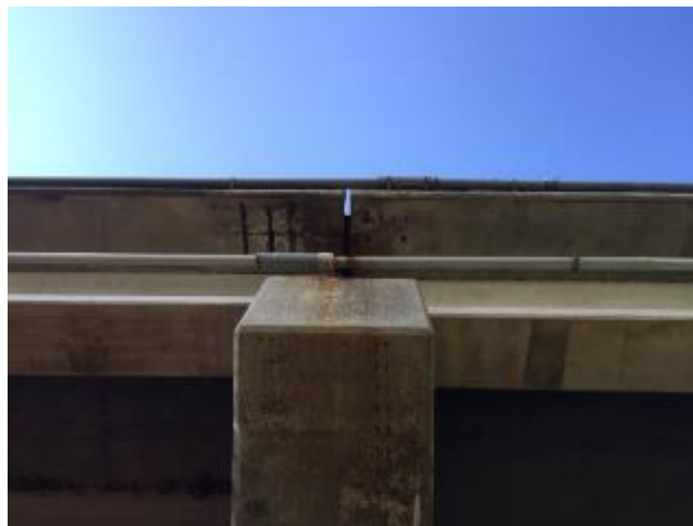
Figure 327. Underside of the SH-3 bridge over N. Canadian River at the candidate joint showing concrete deterioration
