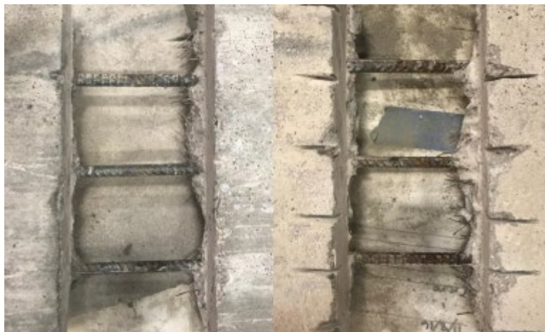
Figure 295. Corrosion state of rebar reinforcing at joint of Phoscrete small-scale corrosion specimens with 4% NaCl (left) and 8% NaCl (right)
