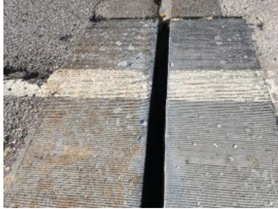
Figure 338. UHPC joint headers on SH-3E bridge before joint sealant was placed and showing surface rusting of the exposed steel fibers
