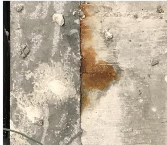
Figure 6.17. Joint corrosion in Ductal ® large-scale corrosion testing specimen during week 2 of testing (Ductal ® on left side of image)
