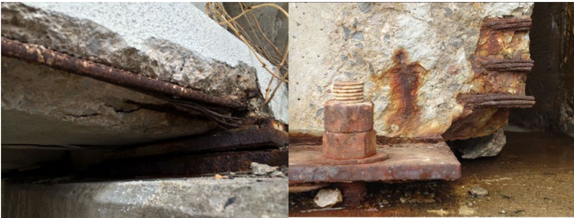
Figure 2.3. Corrosion damage to a precast, prestressed concrete girder end region
