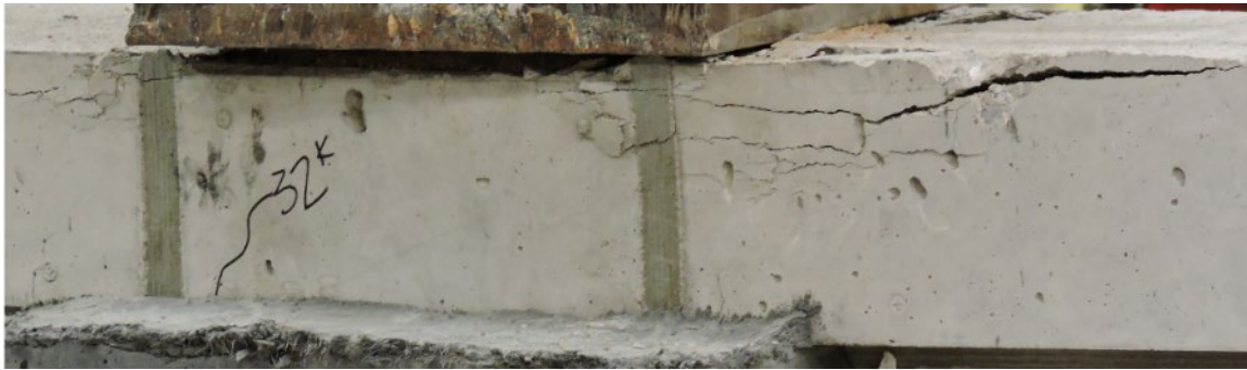
Figure 4.91. Specimen R1-J3 deck crushing at failure
