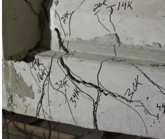
Figure 4.123. Specimen R3-FRSCC deck cracking
