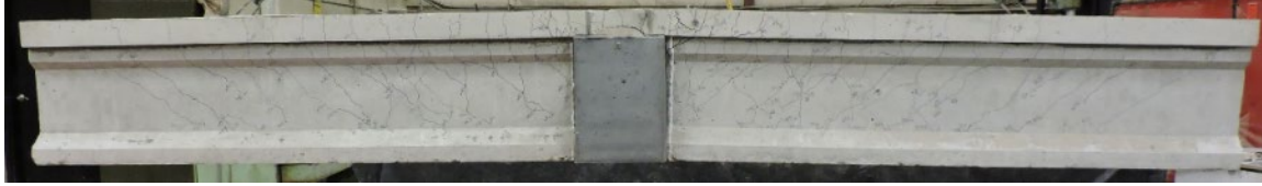
Figure 4.99. Deflected shape of specimen R2-J3 after testing
