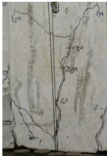
Figure 4.55. Specimen C3 flexural cracking in the continuity joint
