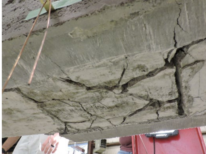
Figure 4.129. Specimen R1-PHOS girder-joint separation
