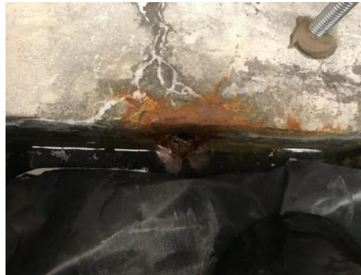
Figure 6.23. Visible confirmation of reinforcing bar corrosion during week 1
