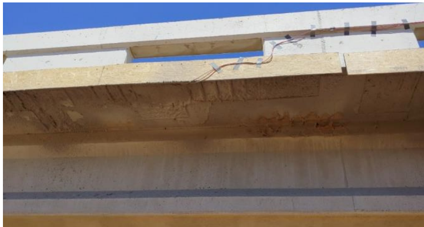
Figure 7.7. Repaired section at the location of the westernmost strain gages (Figure 7.4) after the first layer of MALP was placed
