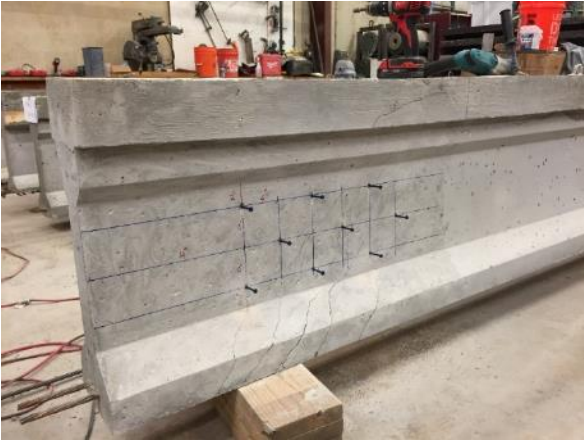
Figure 5.10. Concrete anchors used for shear studs in the web of a girder specimen ready for repair
