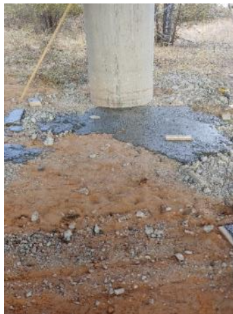
Figure 7.28. UHPC from failed formwork
