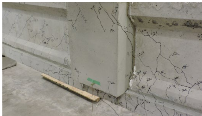
Figure 4.114. Specimen R2-FRSCC shear and flexural cracking
