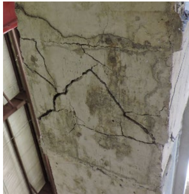
Figure 4.75. Initial cracking of specimen R1-PHOS on the bottom joint face
