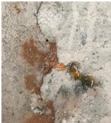
Figure 6.22. Green liquid in joint of Ductal® large-scale corrosion specimen during week 10 of testing
