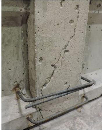
Figure 4.85. Roughened surface of continuity joint to be repaired
