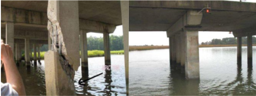
Figure 2.29. Damaged (left) and SCC repaired bridge pier (right) (Ozyildirim 2013)
