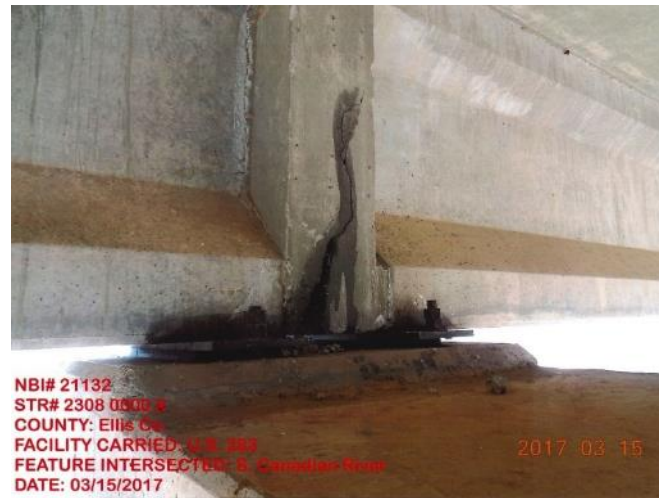
Figure 2.2. Cracking in continuity linkage block (photo courtesy of Walt Peters)
