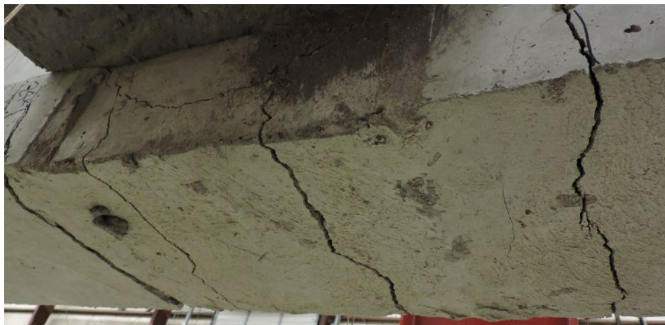
Figure 4.143. Specimen R3-PHOS deck cracking
