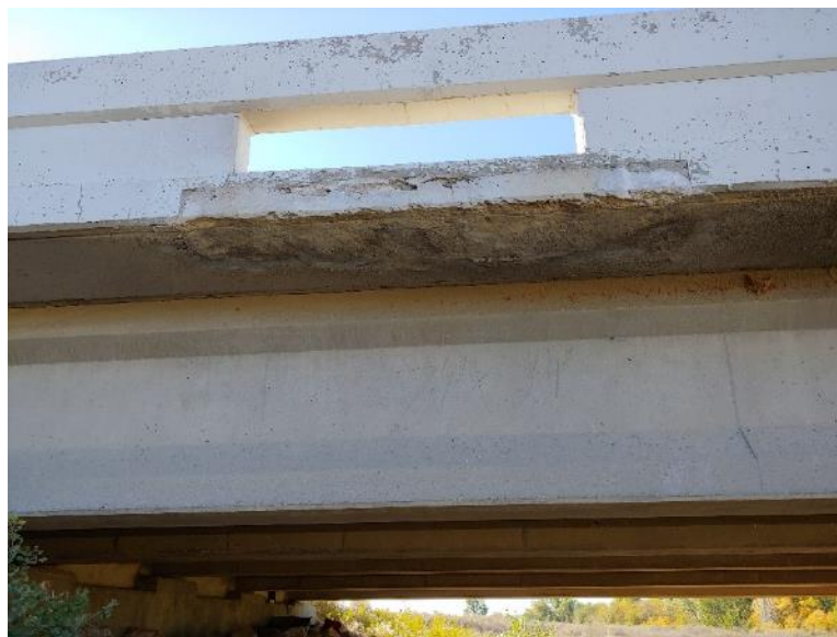
Figure 7.11. Repair spalling on the northeast side of the bridge 18 months after repair
