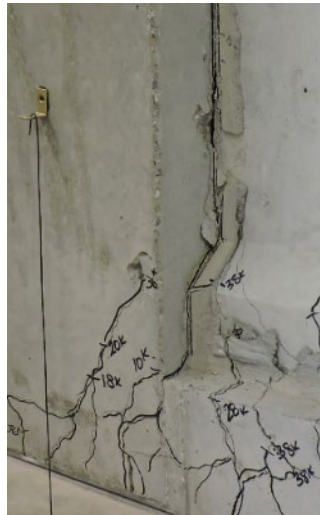
Figure 4.49. Specimen C2 cracking at girder-joint interface (right side)
