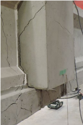
Figure 4.122. Specimen R3-FRSCC joint cracking on the longitudinal and transverse faces from the back left
