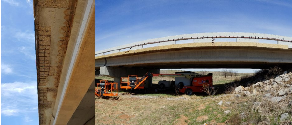
Figure 7.4. Slab cantilever section after removal of loose material (left) and forms in place for the repair (right)
