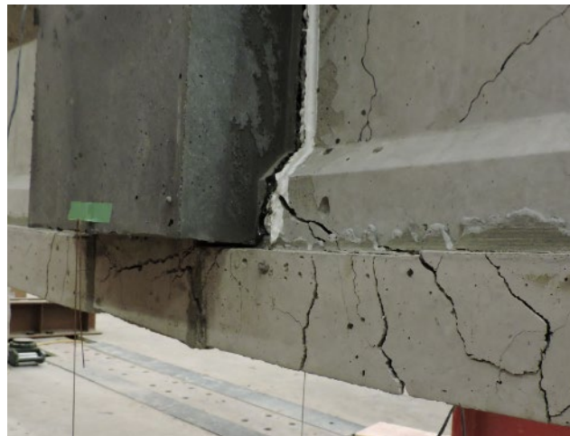
Figure 4.98. Specimen R2-J3 girder-joint interface cracking on the back right
