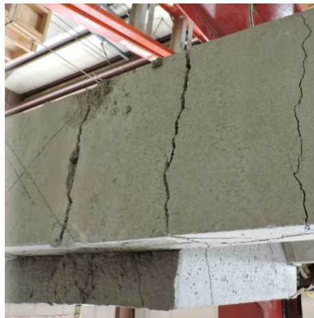
Figure 4.136. Specimen R2-PHOS deck cracking
