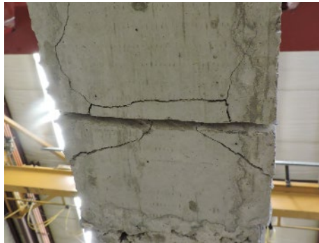
Figure 4.65. Initial cracking of specimen R2-J3 on the bottom joint face
