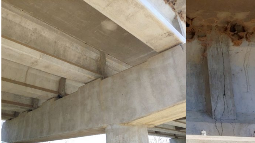
Figure 7.19. Joints at pier 3 prior to repair (left) and typical damage (right)
