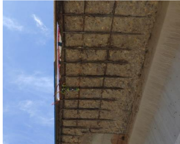
Figure 7.5. Strain gauge placement within the area to be repaired on the south side of span 3 of the S.H. 3 bridge over Fulton Creek in Beaver County
