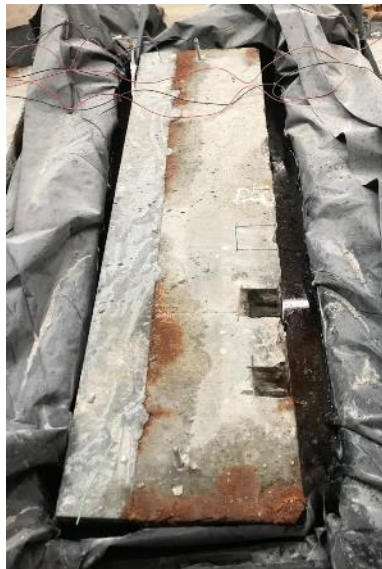
Figure 6.18. Joint corrosion in Ductal ® large-scale corrosion specimen during week 5 of testing
