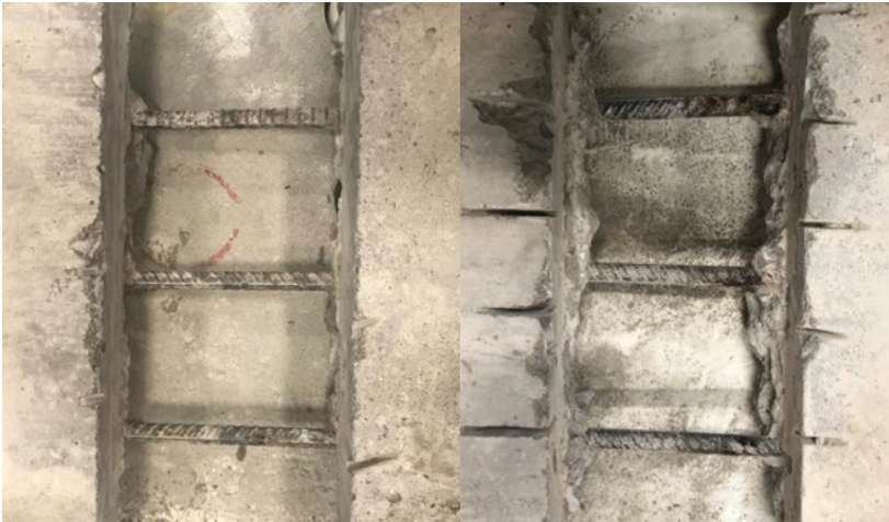
Figure 6.5. Corrosion state of rebar reinforcing at joint of ODOT Class AA small-scale corrosion specimens with 4% NaCl (left) and 8% NaCl (right)
