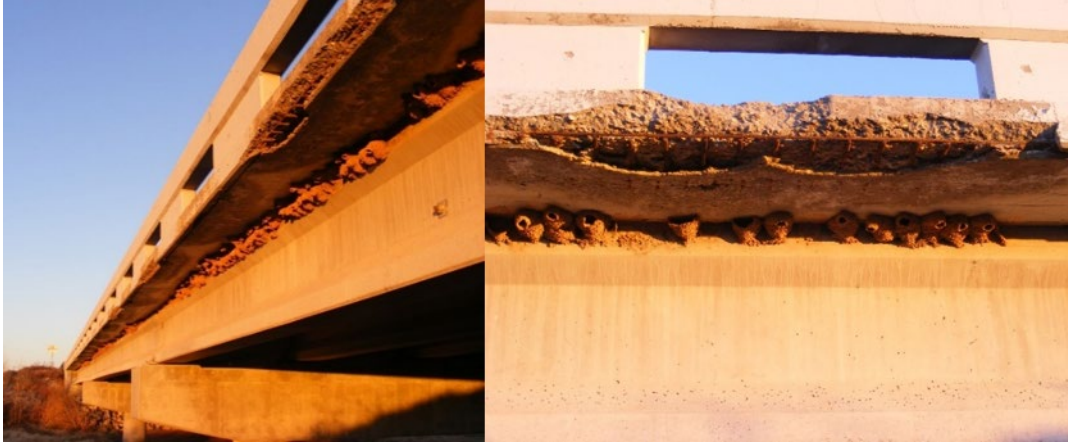
Figure 7.2. Typical spalling on slab cantilever of Fulton Creek bridge
