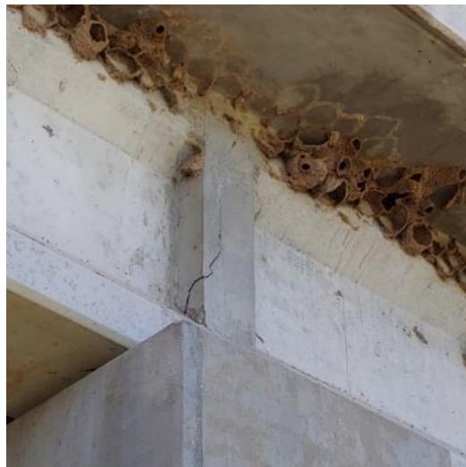
Figure 7.16. Example of positive moment cracking in a continuity joint of the U.S. 183/412 bridge over Wolf Creek
