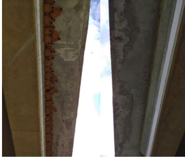
Figure 7.9. Close-up initial MALP placement on the southeast side (left) and later MALP placement on the northeast side (right) showing difference in surface finish of repair
