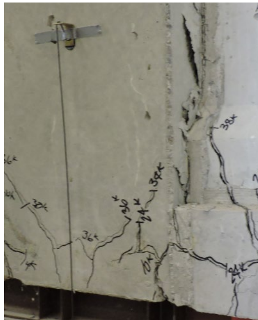
Figure 4.41. Specimen C1 cracking at girder-joint interface (right side)
