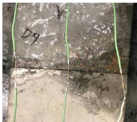
Figure 6.4. Initial joint corrosion in Ductal® small-scale corrosion testing specimen - corrosion spotting
