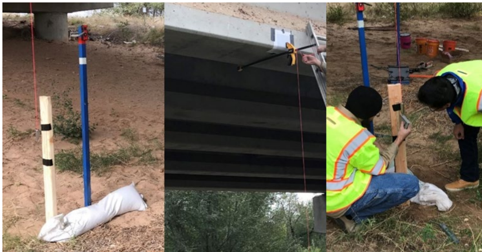
Figure 7.21. Laser measurer and plumb bob setup (left), clamp on the girder bottom (middle), and method used for measurement with the plumb bob (right)
