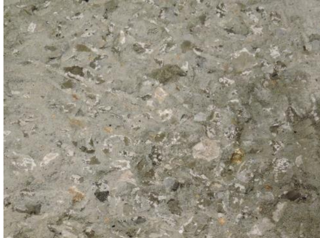
Figure 3.11 Chipped top surface of substrate (ODOT AA pull-off slabs)
