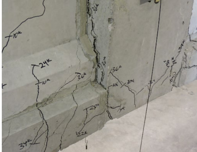
Figure 4.40 Specimen C1 cracking at girder-joint interface (left side)
