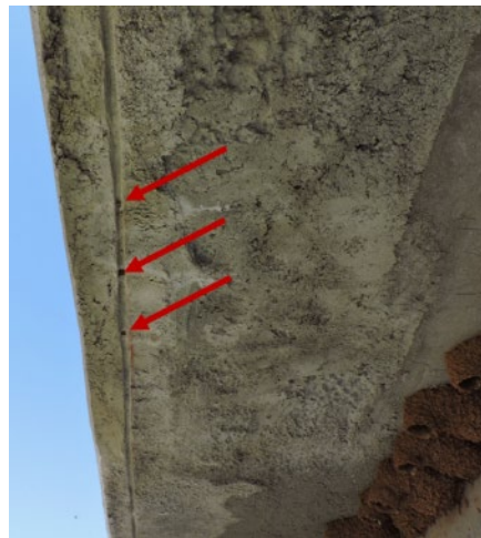
Figure 7.10. Rust spot in this section of MALP repair where drip edge was cut on the south side of the bridge
