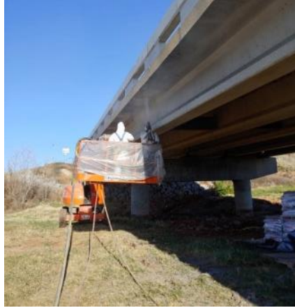
Figure 7.6. Placement of MALP mortar on the S.H. 3 bridge over Fulton Creek in Beaver County
