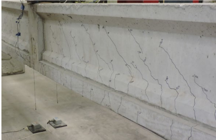
Figure 4.54. Specimen C3 shear cracking
