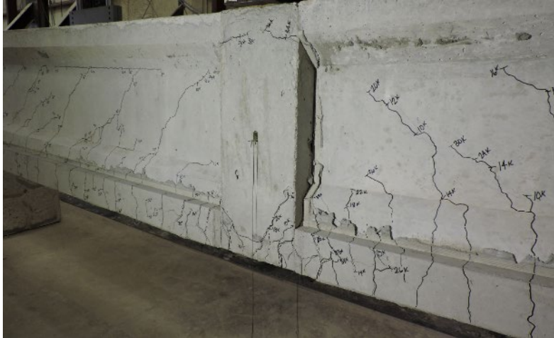
Figure 4.46. Specimen C2 shear cracking
