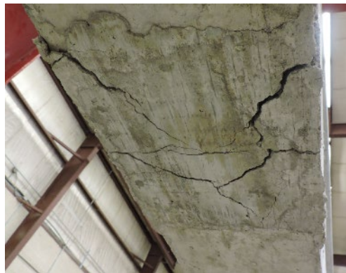
Figure 4.73. Initial cracking of specimen R3-FRSCC on the bottom joint face
