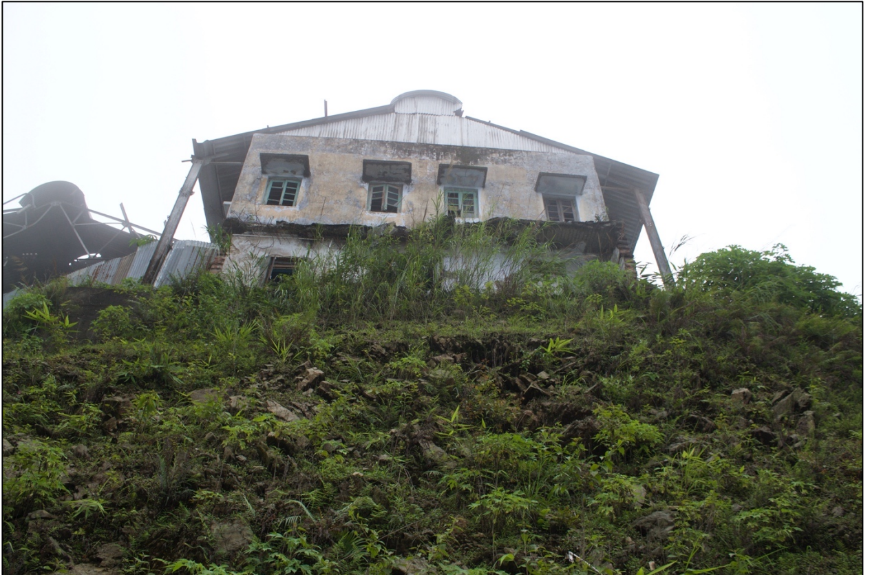
Fig. 4.1. Railway Workshop Structure vandalized and bombed between 1986 and 1988 in Tindharia, Kurseong. (Picture taken during fieldwork, 2016)
