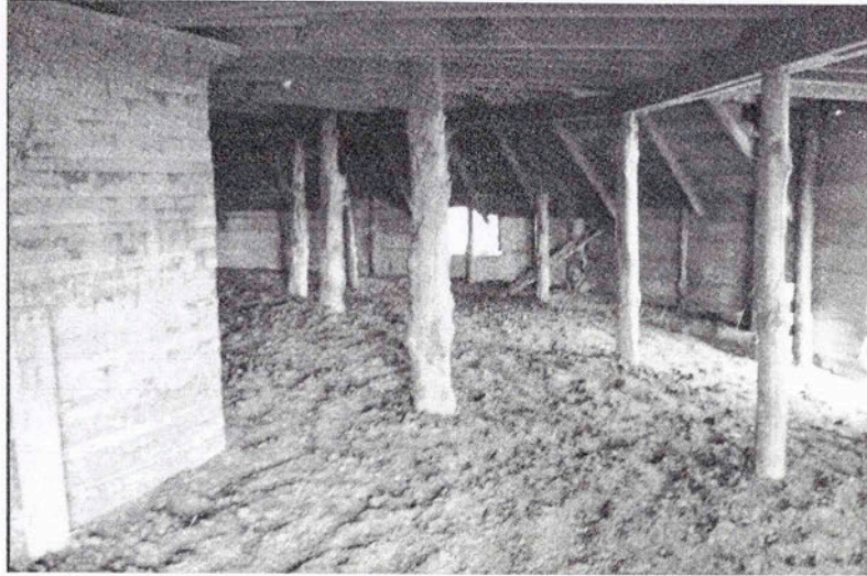
Fig. 5.64 Posts of bois d'arc placed throughout the structure to support loft floor joists. (Photo by Lynda Ramsey)
