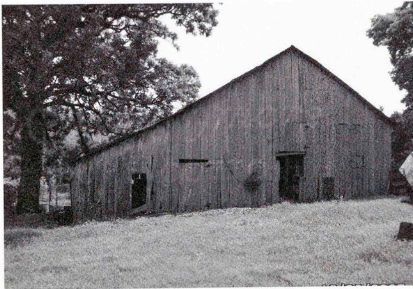
North gable end of Sober's barn and calf shed on the east added later.
