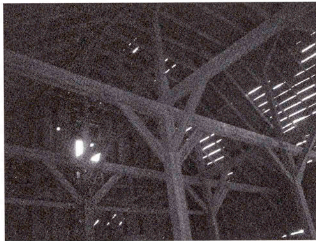
Post and beam construction inside the hay loft of the Hinger-Smith barn.
