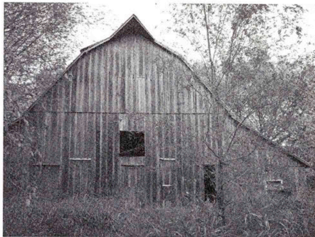
South view of the spread gambrel roof, triangular hay hood, and hinged doors with metal pentice.
