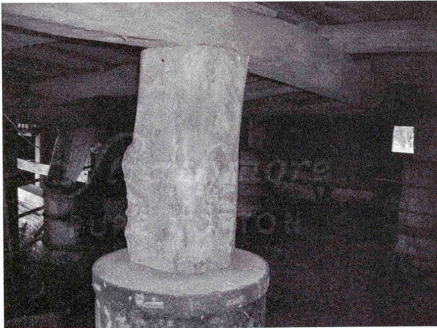
Cottonwood post positioned on top of a concrete cylinder covered in metal and iron reinforcement belts. The rough hewn post is supporting a hayloft floor joist post.
