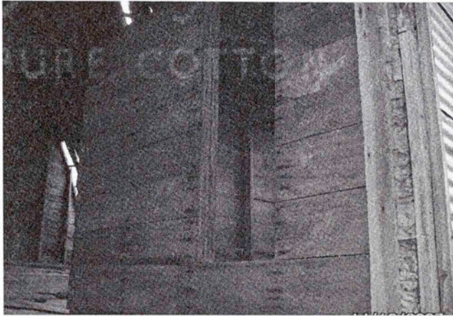
Granary located just west of the sliding wagon door on the north.
