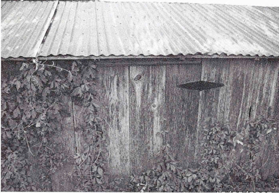
Fig. 5.37 One of three entries into the haymow on the upper ground level of Martin Stadler and Tom and Edna Beck's hillside barn. (Photo by Lynda Ramsey)
