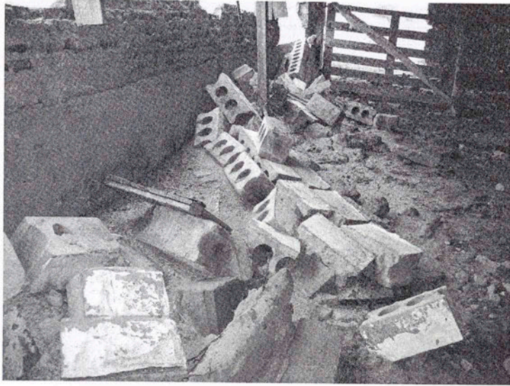
Fig. 5.49 Concrete blocks have fallen away from the outside wall, exposing the inside of the barn. (Photo by Lynda Ramsey)
