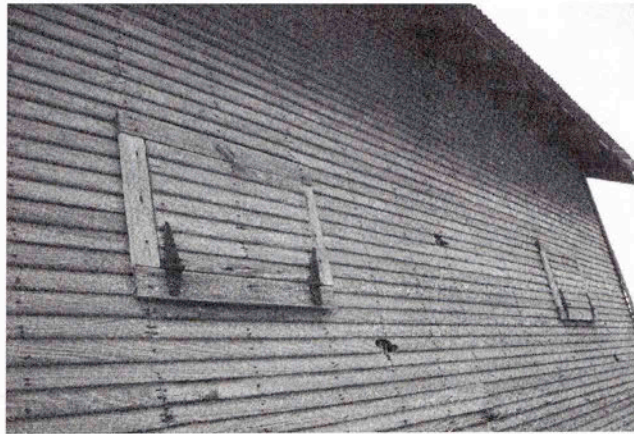
Shutter windows that access the granaries on the north side of the Upright's barn.
