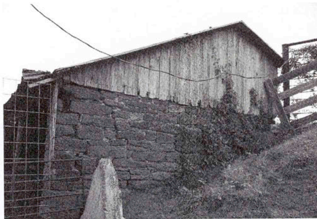
The east side of the barn has a red sandstone foundation/wall with vertical wood siding on the upper gable.
