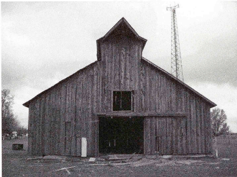
West end of Jones’ horse barn with monitor roof and triangular hay hood.
