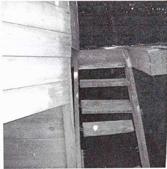
Fig. 5.60 Stairway located on the west side of the Rohwer barn leads into the hayloft from the ground floor. All entrances into the loft are on the west side of the barn. (Photo by Lynda Ramsey)
