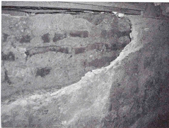
Fig. 5.50 Portland cement plaster veneer on the interior brick wall. (Photo by Lynda Ramsey)
