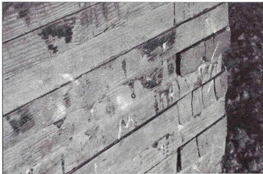
Fig. 5.70 The silo was built using laminated layers of lumber sealed with tar. (Photo by Lynda Ramsey)
