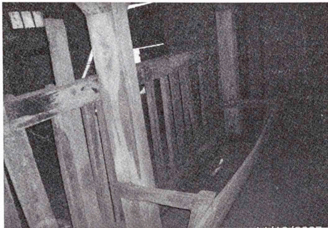
Wood dairy stanchions and feed troughs in the basement of F.A. Hall and Mach's barn.
