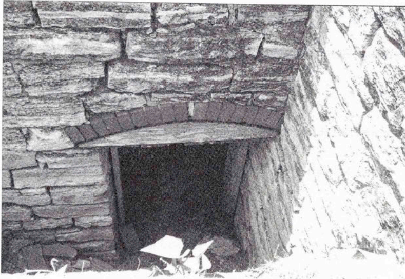
Fig. 5.19 A red brick jack arch over the root cellar door. (Photo by Lynda Ramsey)
