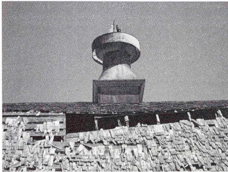
Fig. 5.56 The metal ventilator on the top of the Rohwer's Dutch gambrel roof was very popular on dairy barns before World War II.
