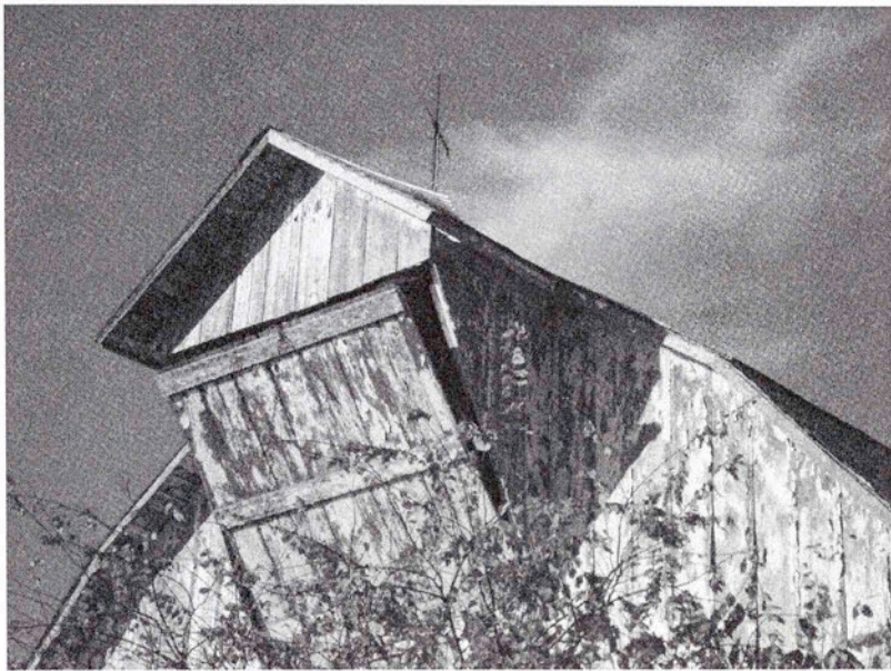
Boxed hay hood and hinged hayloft door. Wind vane and lightning rod on ridge of the roof.
