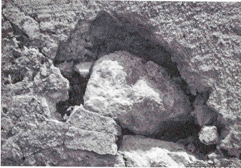
Figure 5.23 Field stone used in the concrete mixture of John W. Carter's barn. (Photo by Lynda Ramsey)
