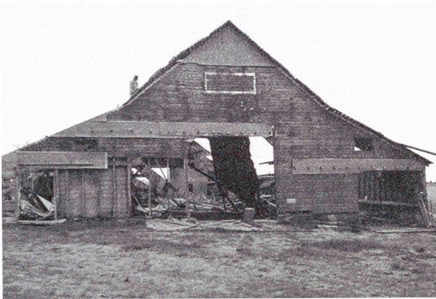
Vaclav Dobry barn in 2007 during demolition, to prepare land for housing development.
