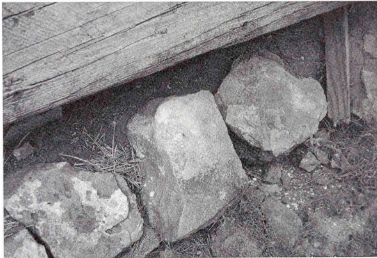
Figure 5.72 Fieldstone foundation in Don Elemnhorst and Frank Blaha's barn. (Photo by Lynda Ramsey)
