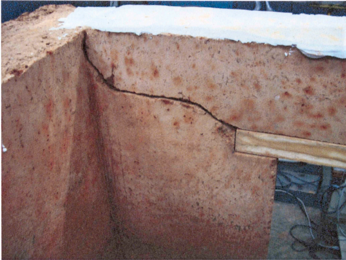
Figure 3.3: Test 1 interior view of crack above lintel in NE corner
