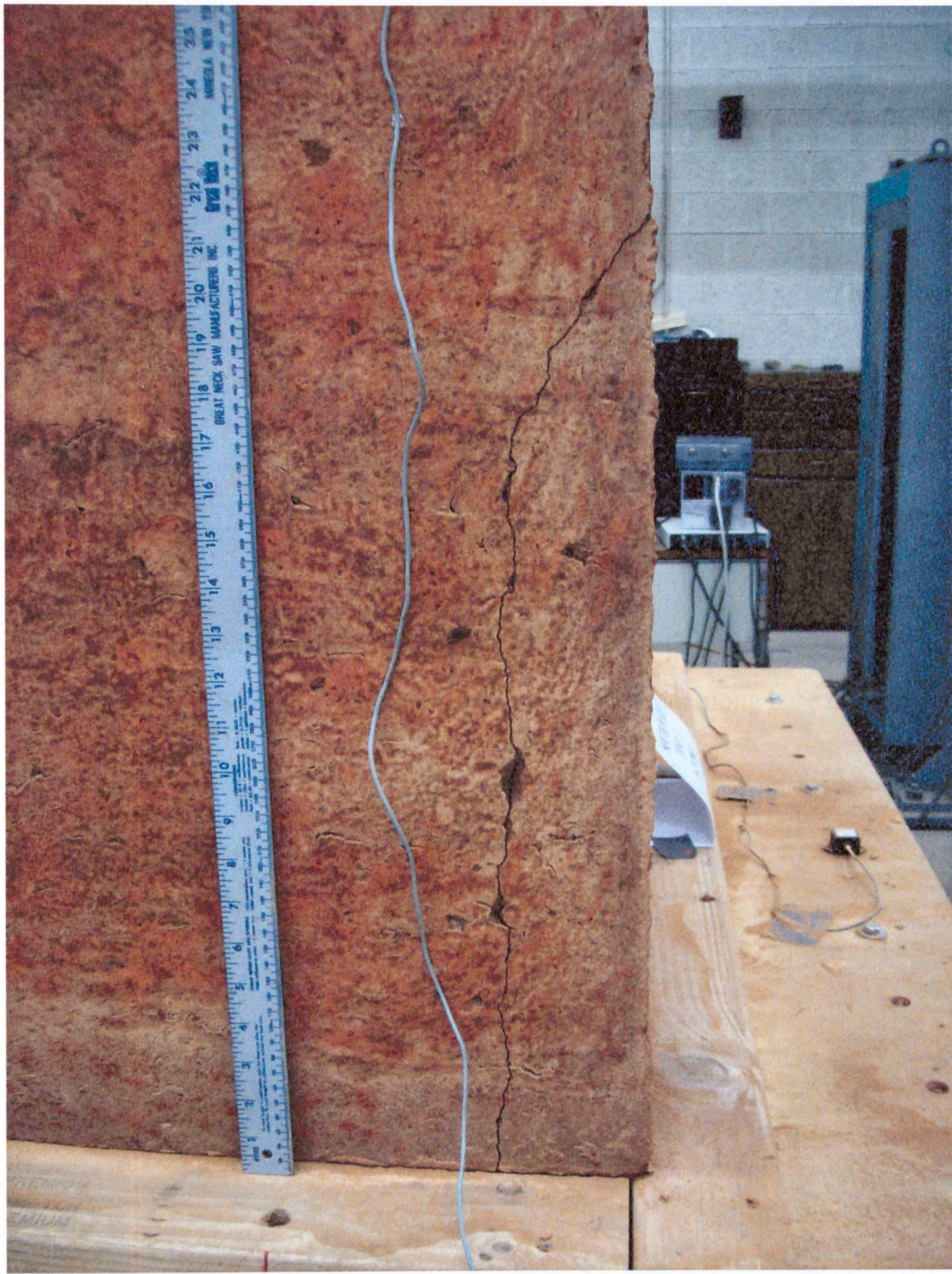
Figure 3.33: Test 3 view of crack near base of west wall at SW corner
