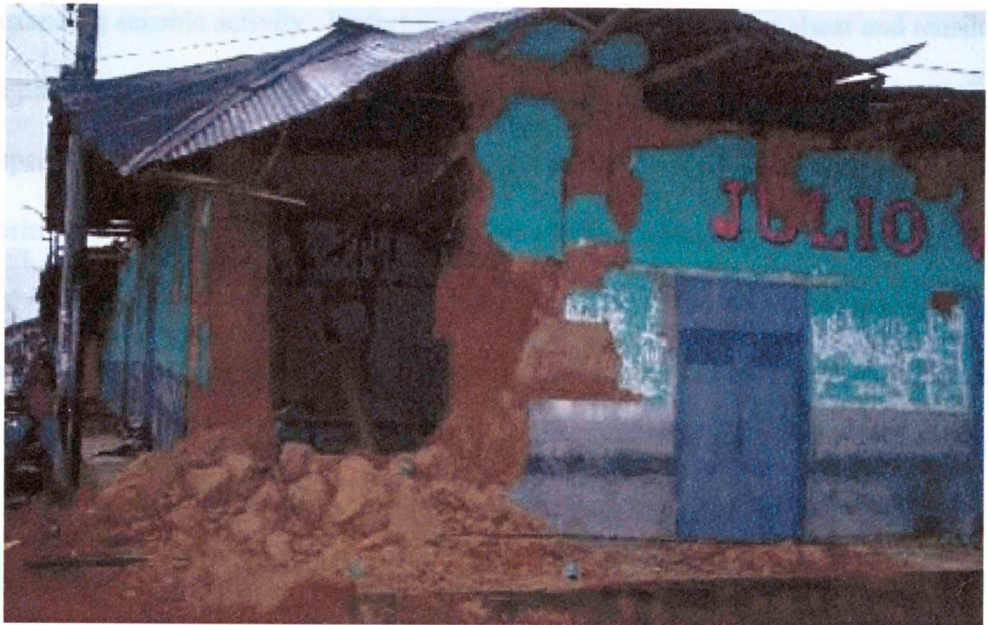
Figure 1.1: Earthquake damage to rammed earth in Peru ( www.lamasperu.com )
