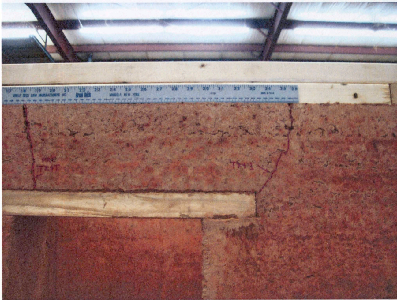
Figure 3.29: Test 3 cracks above lintel near NE corner of east wall
