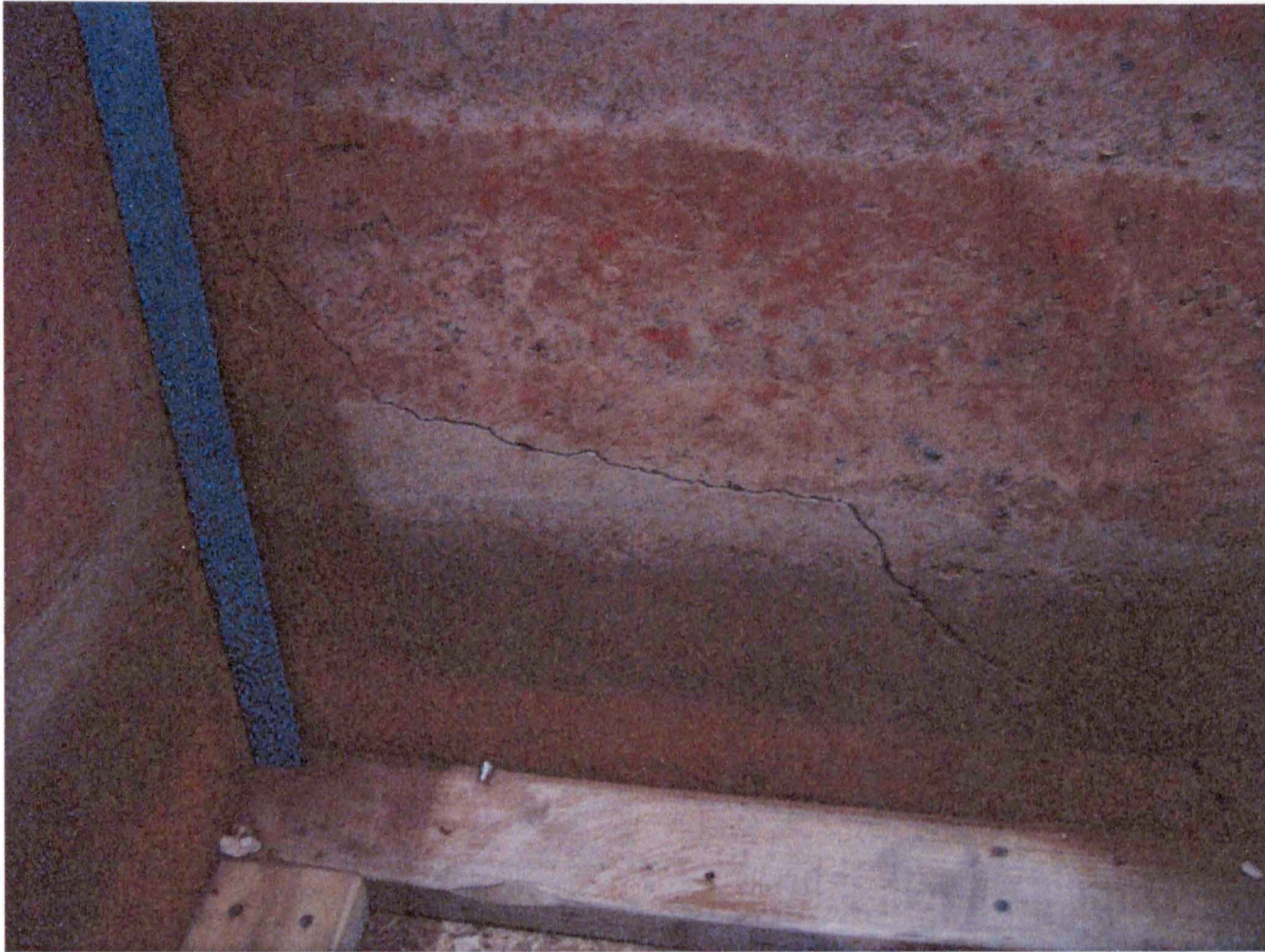
Figure 3.11: Test 1 interior of crack along north wall
