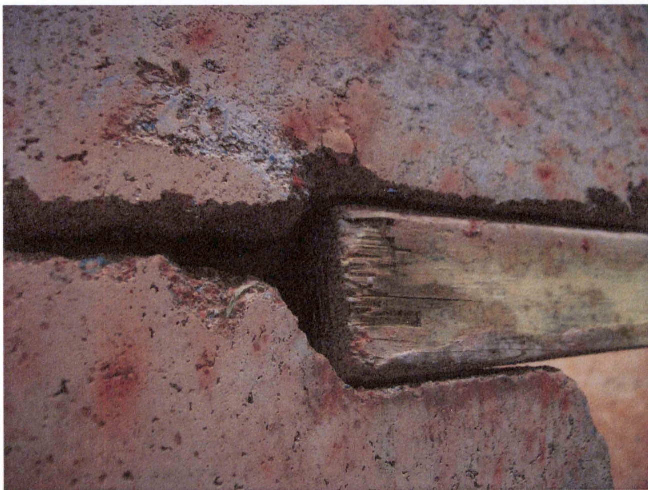
Figure 3.4: Test 1 closeup view of exterior crack near lintel
