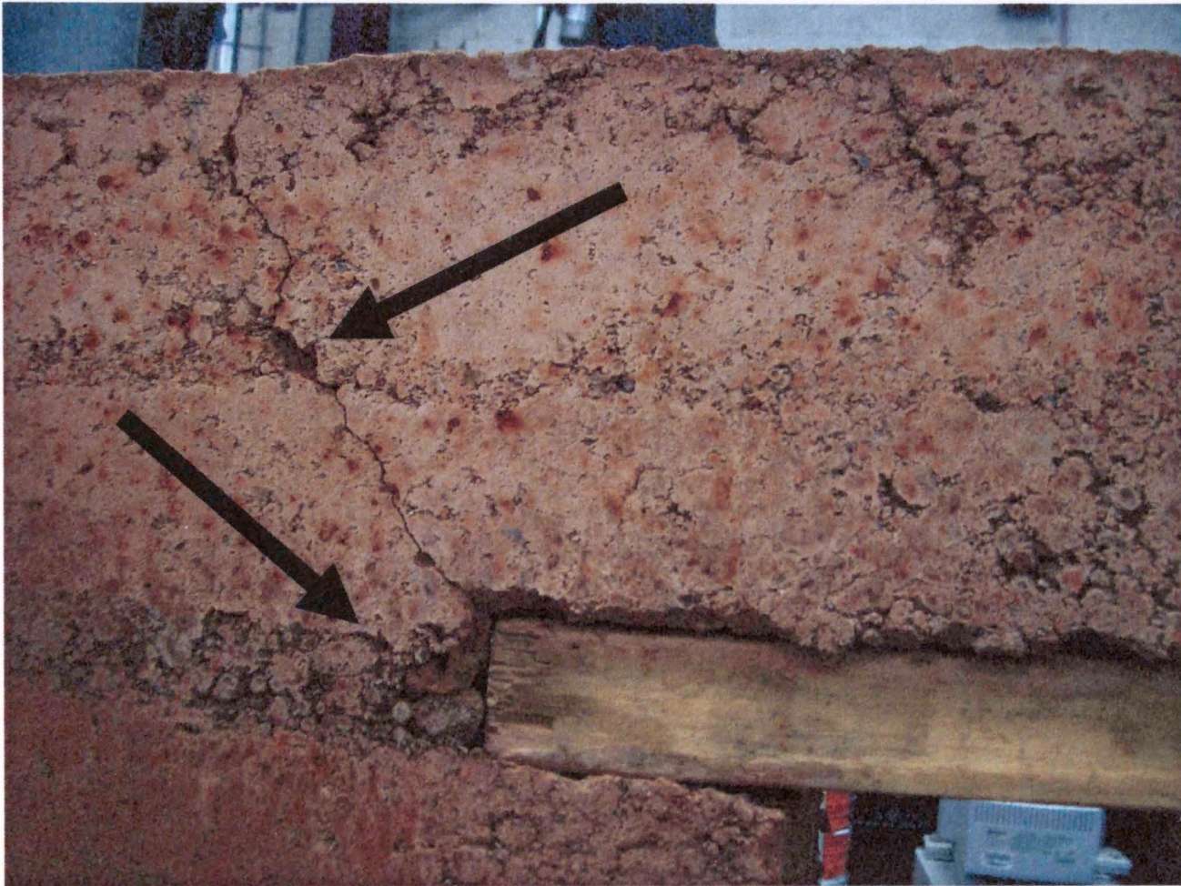
Figure 3.17: Test 2 close up view of crack in NE corner above lintel after test, note less compacted soil adjacent to edge of lintel
