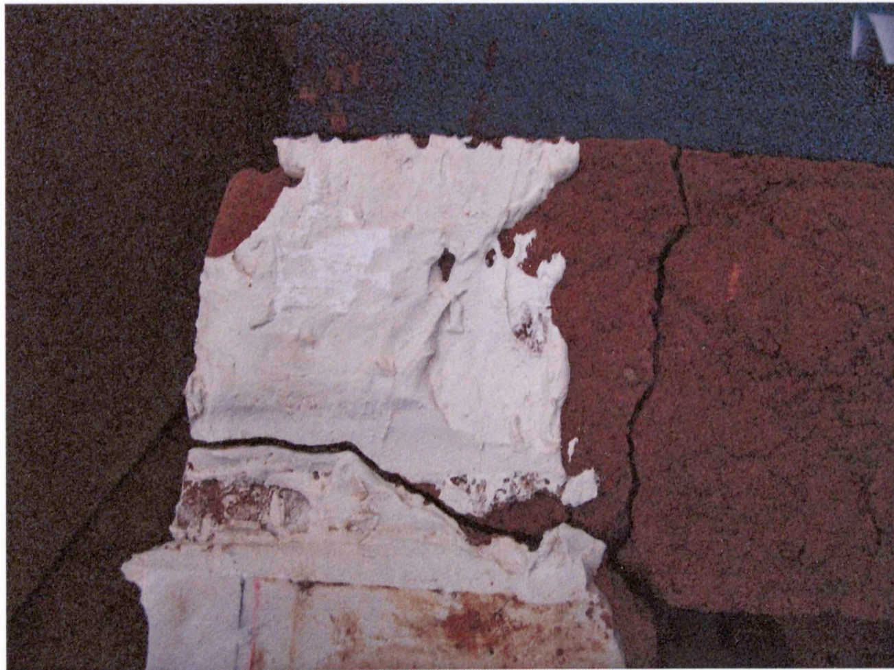
Figure 3.8: Test 1 plan view above cracked northwest corner of north wall
