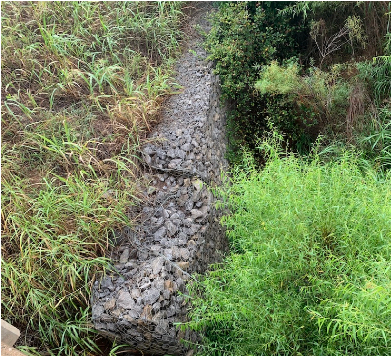
Figure 65: Gabion baskets at site 31
