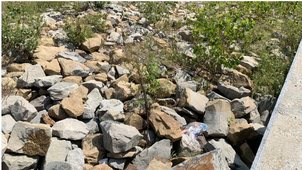
Figure 4: Rip rap along bridge abutment in good condition, taken near Laverne, Oklahoma, in 2020.
