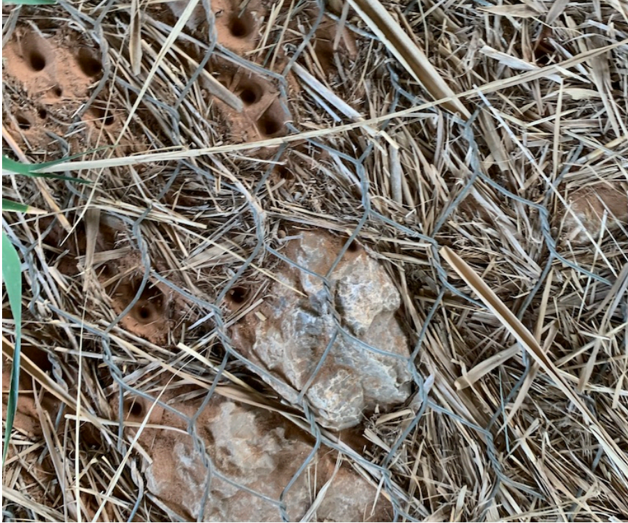
Figure 66: Sunken gabion baskets at site 26
