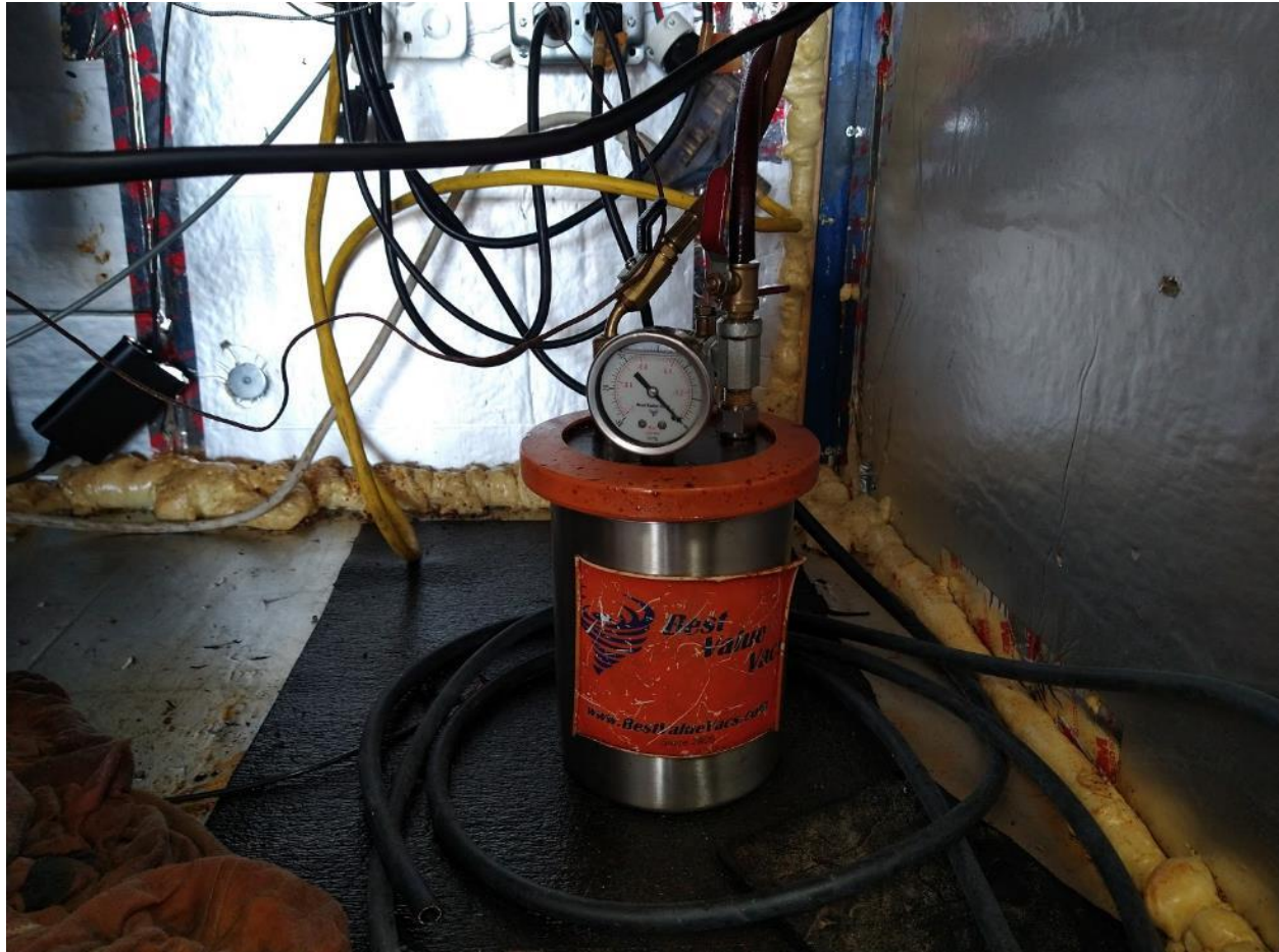
Figure 4.8: Vacuum tank as installed in the system. The vacuum tank prevents the ingress of oil into the vacuum pump and the generation of oil mist.
