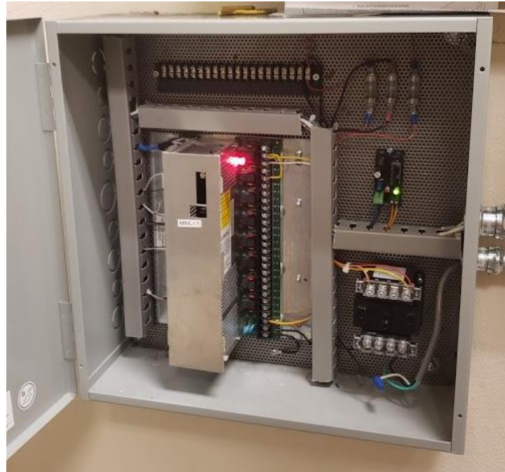
Figure 3-8: Additional Building Automation System MNL800 Controller
