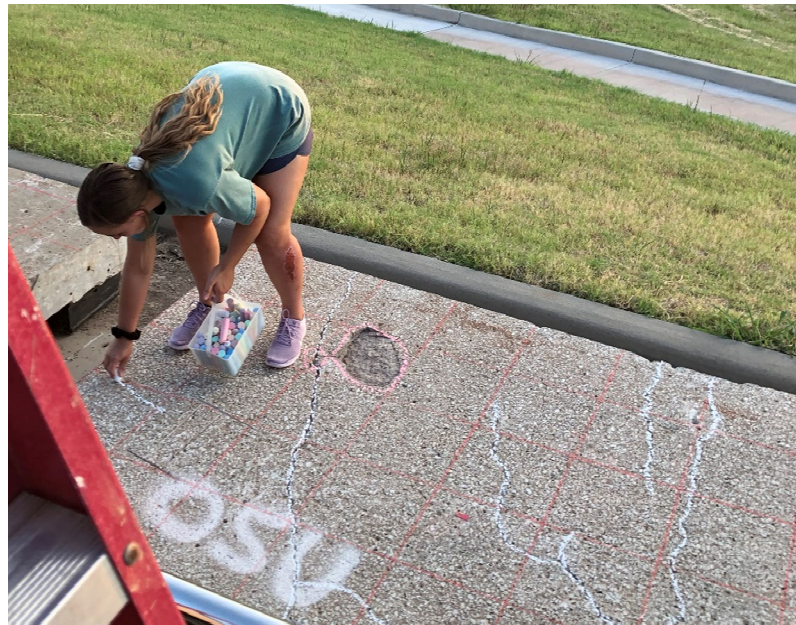
Figure 4.2: Crack Mapping for Visual Condition Survey
