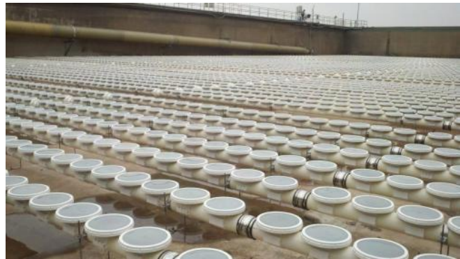
Figure 2: Aeration Basin Diffusers
