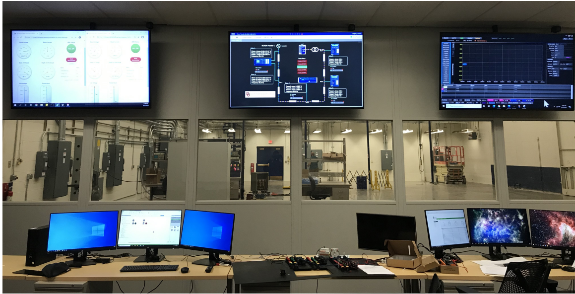
Fig. 3.13: Control Room Visual Display System
