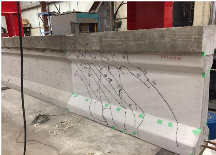
Figure 3.11: Tracing paper on one side of the cracked girder to copy the cracks' location
