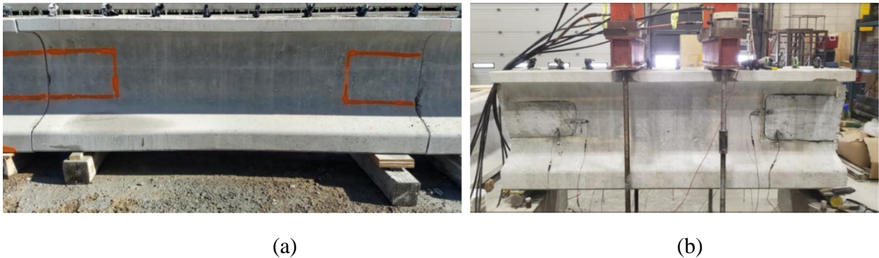
Figure 2.10: (a) Cut beam segment marked for controlled damage and (b) loading setup for testing repaired beam segment (Shafei, 2020)
