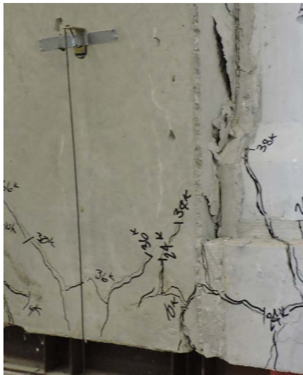
Figure 4-8: CI Cracking at Girder-Joint Interface (Right Side)
