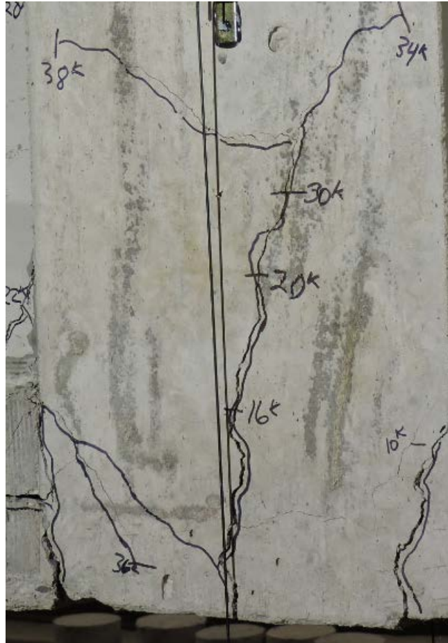
Figure 4-22: C3 Cracking in Continuity Joint
