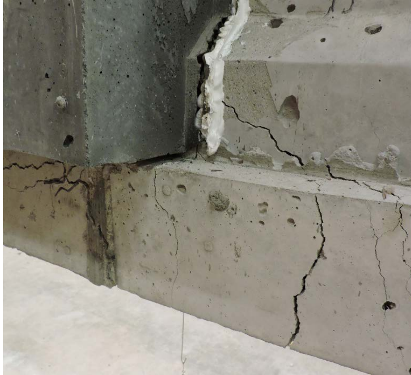
Figure 6-10:R2-J3 Girder-Joint Interface Cracking (Front Right)
