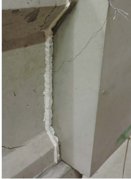
Figure 6-34:R2-FRSCC Joint Cracking, Longitudinal & Transverse Faces (Back Left)
