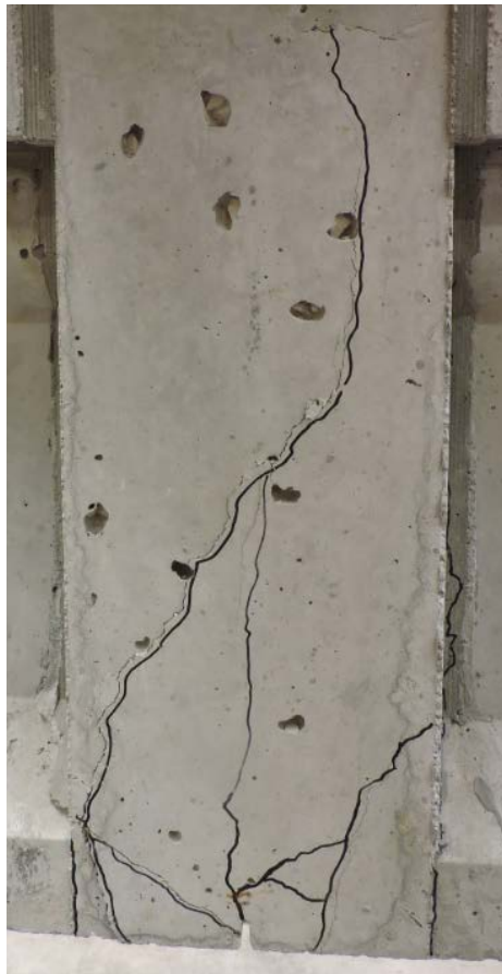
Figure 4-29:R1-J3 Rear Joint Face Initial Cracking
