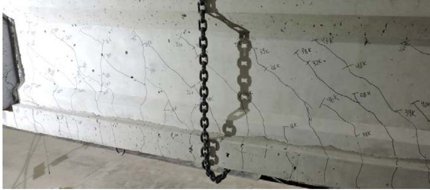
Figure 6-64:R3-PHOS Shear & Flexural Cracking (Front Right)
