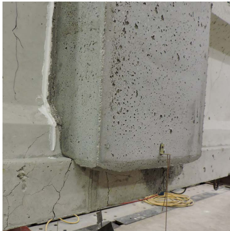
Figure 6-67:R3-PHOS Joint Transverse Face Cracking (Back Left)
