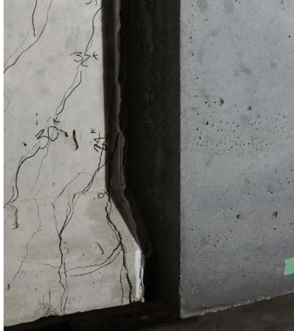
Figure 6-3:R1-J3 Girder-Joint Interface Crack (Left)
