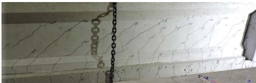
Figure 6-63:R3-PHOS Shear & Flexural Cracking (Front Left)
