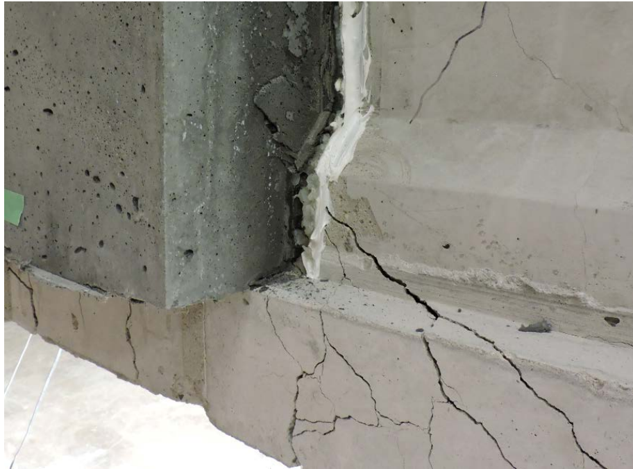
Figure 6-17:R3-J3 Girder-Joint Interface Cracking (Right)
