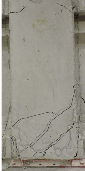
Figure 4-44:R3-FRSCC Front Joint Face Initial Cracking
