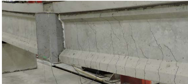
Figure 6-46: R1-PHOS Shear & Flexural Cracking
