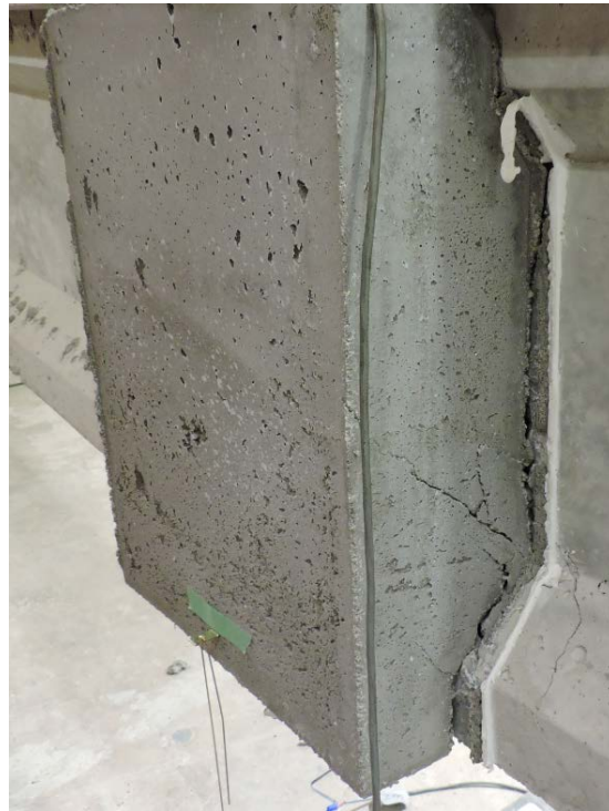
Figure 6-50:R1-PHOS Girder-Joint Interface & Joint Transverse Face Cracking (Back Right)
