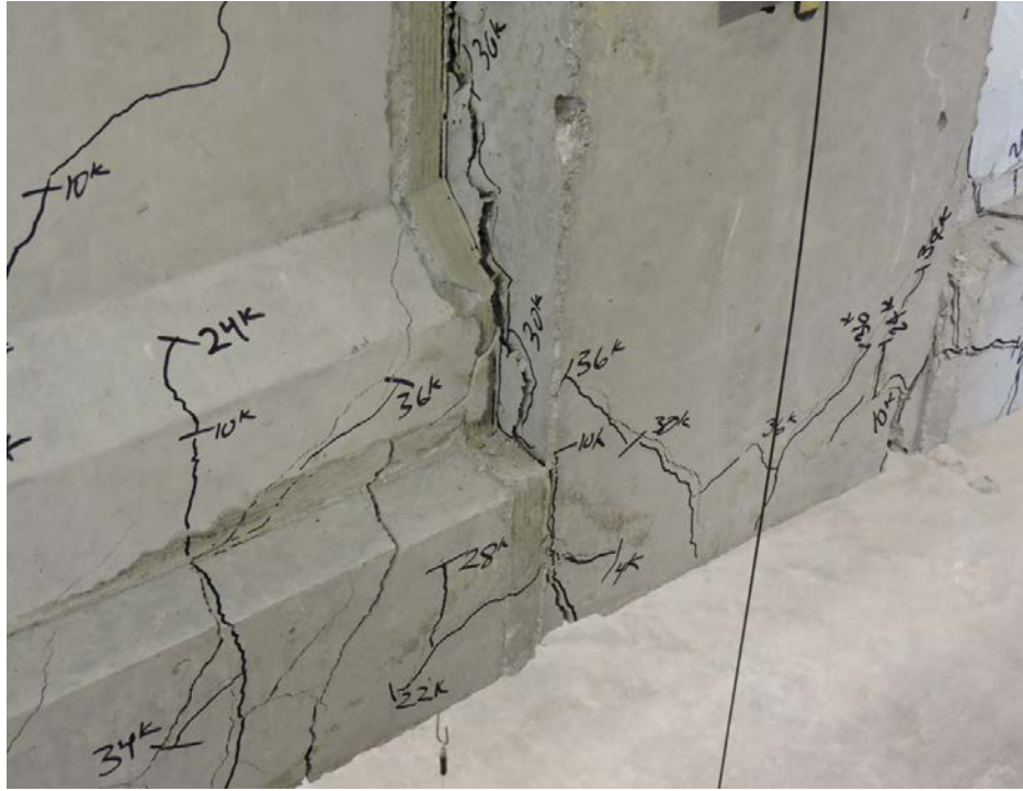
Figure 4-7: CI Cracking at Girder-Joint Interface (Left Side)
