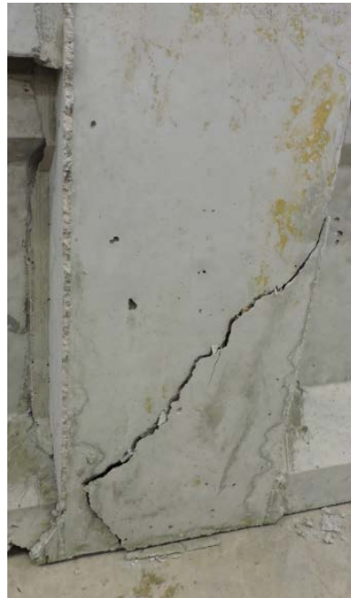
Figure 4-52:R2-PHOS Rear Joint Face Initial Cracking
