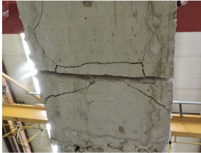
Figure 4-33:R2-J3 Bottom Joint Face Initial Cracking
