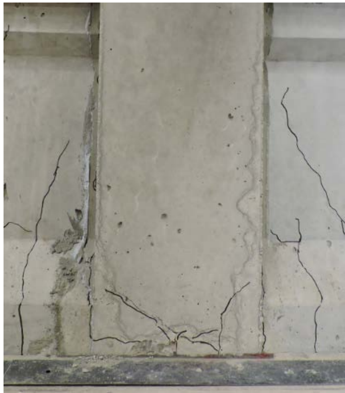
Figure 4-31:R1-J3 Front Joint Face Initial Cracking
