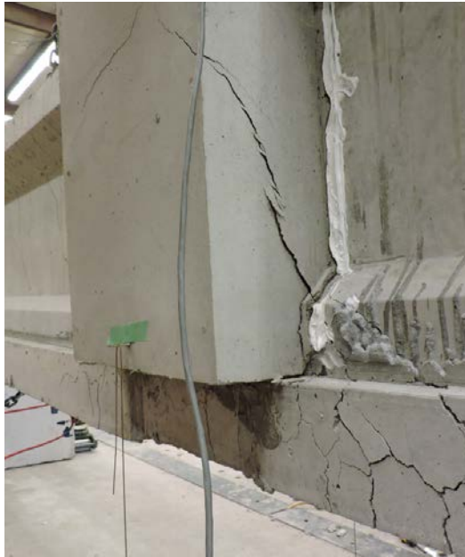
Figure 6-35:R2-FRSCC Joint Cracking, Longitudinal & Transverse Faces (Back Right)
