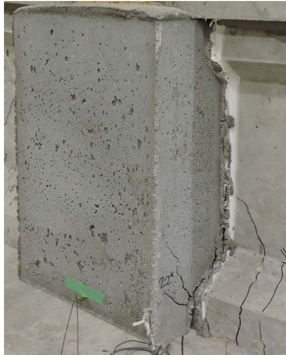
Figure 6-48:R1-PHOS Girder-Joint Interface & Joint Transverse Face Cracking (Front Right)
