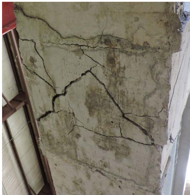
Figure 4-48:R1-PHOS Bottom Joint Face Initial Cracking
