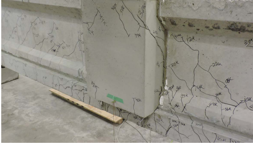
Figure 6-31: R2-FRSCC Shear & Flexural Cracking
