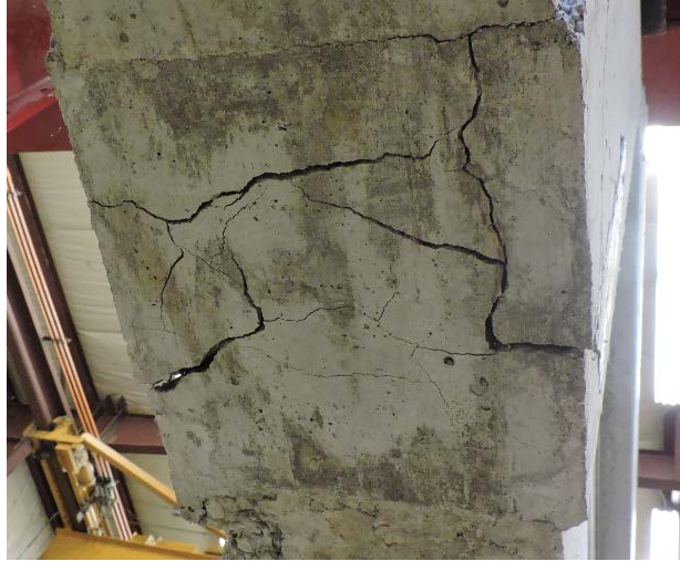
Figure 4-51:R2-PHOS Bottom Joint Face Initial Cracking
