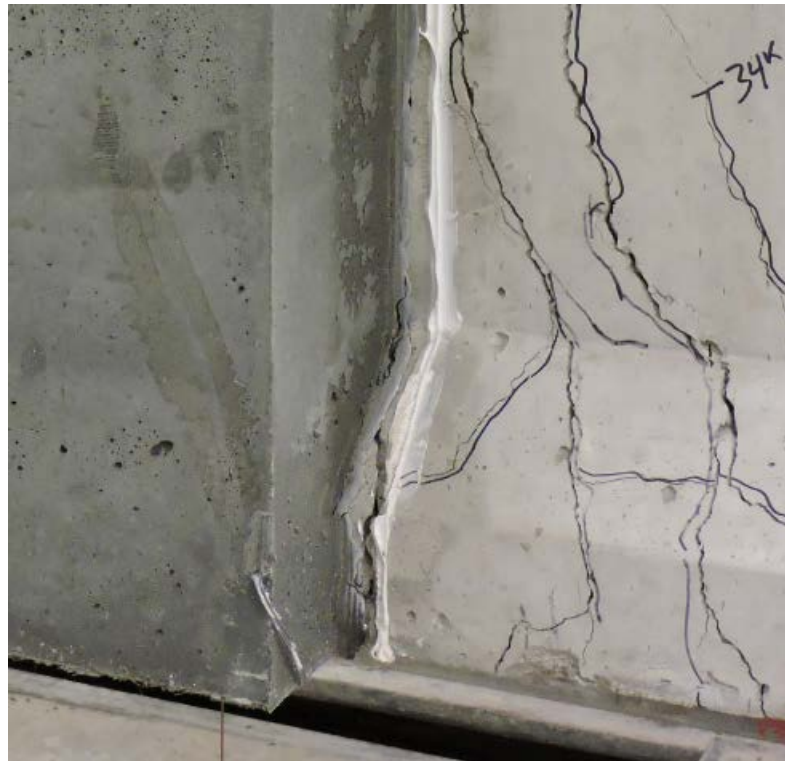
Figure 6-2:R1-J3 Girder-Joint Interface Crack (Right)
