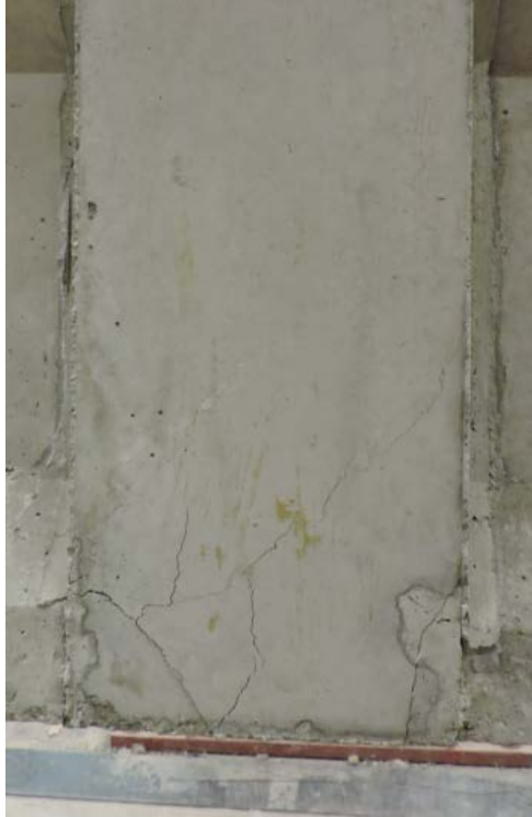
Figure 4-43:R2-FRSCC Rear Joint Face Initial Cracking
