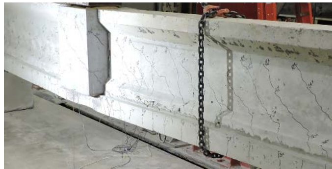
Figure 6-55: R2-PHOS Shear & Flexural Cracking
