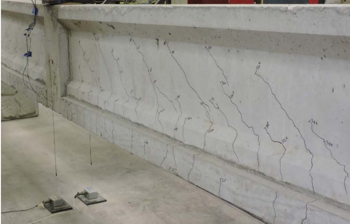
Figure 4-21: C3 Shear Cracking
