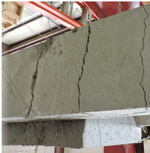
Figure 6-59:R2-PHOS Deck Cracking
