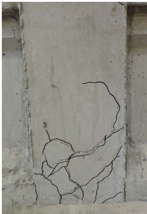
Figure 4-37:R3-J3 Rear Joint Face Initial Cracking
