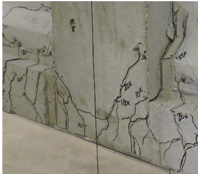
Figure 4-14:C2 Initial Cracking in Continuity Joint
