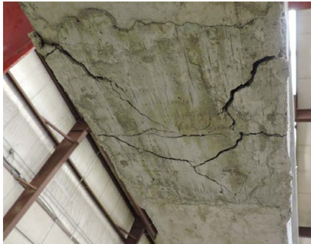
Figure 4-45:R3-FRSCC Bottom Joint Face Initial Cracking
