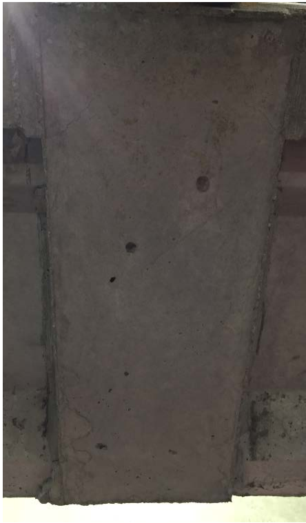
Figure 4-40:R1-FRSCC Rear Joint Face Initial Cracking
