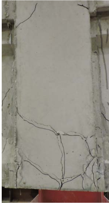
Figure 4-41:R2-FRSCC Front Joint Face Initial Cracking
