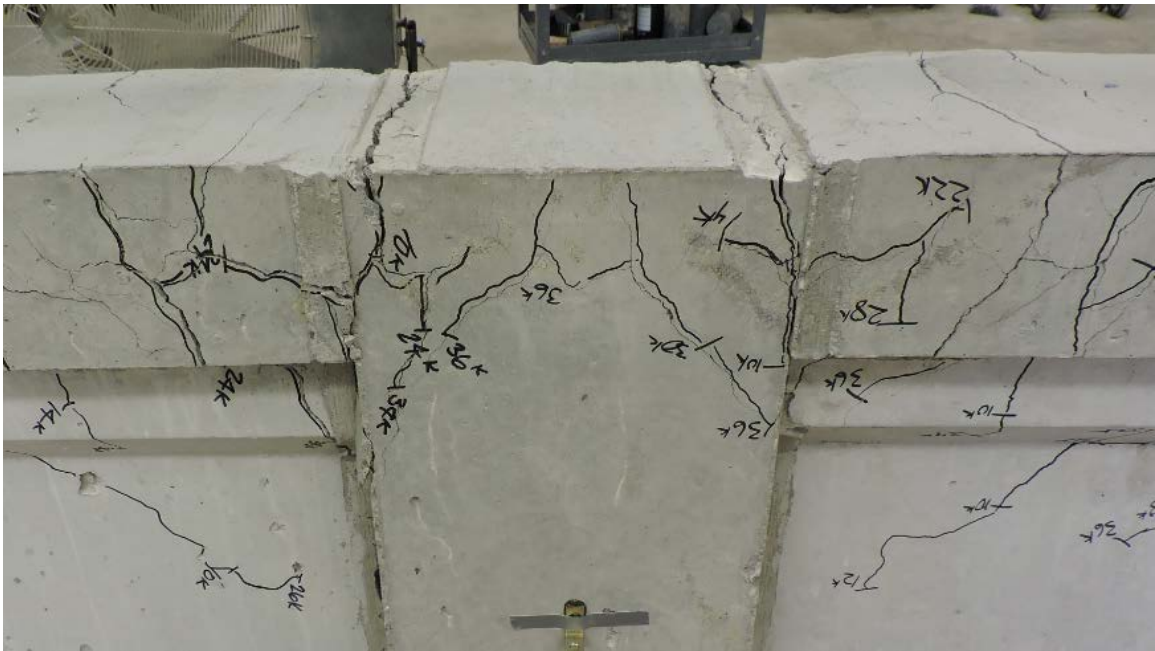
Figure 4-9: C1 Girder-Joint Interface Cracking across the Deck
