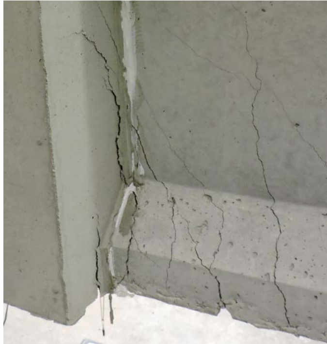
Figure 6-24:R1-FRSCC Joint Transverse Face Cracking (Back Right)
