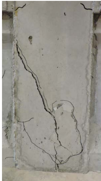
Figure 4-50:R2-PHOS Front Joint Face Initial Cracking
