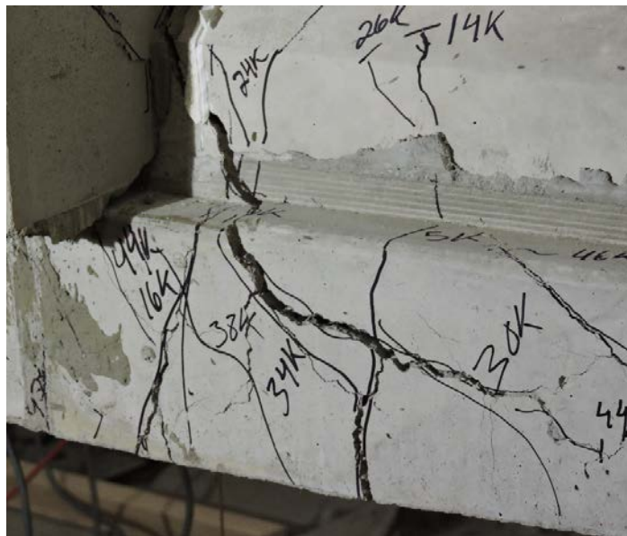
Figure 6-43:R3-FRSCC Deck Cracking
