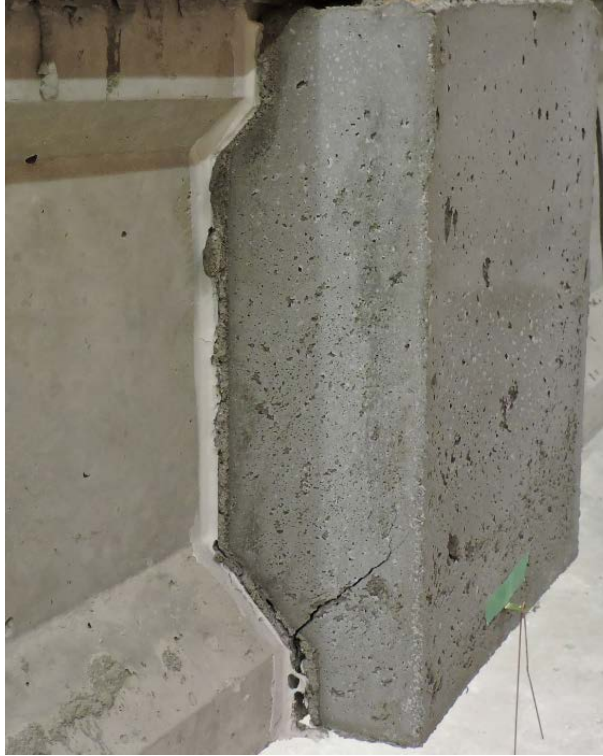
Figure 6-49:R1-PHOS Girder-Joint Interface & Joint Transverse Face Cracking (Back Left)
