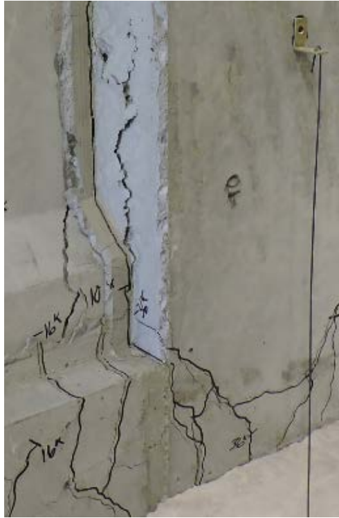
Figure 4-15: C2 Cracking at Girder-Joint Interface (Left Side)
