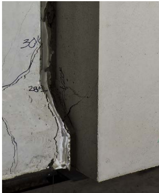
Figure 6-26: R1-FRSCC Girder-Joint Interface Cracking (Front Left)
