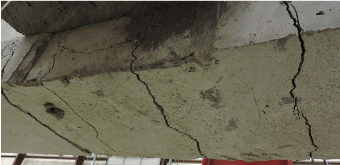
Figure 6-69:R3-PHOS Deck Cracking
