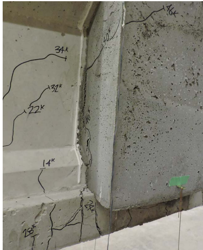
Figure 6-65:R3-PHOS Girder-Joint Interface Cracking (Front Left)
