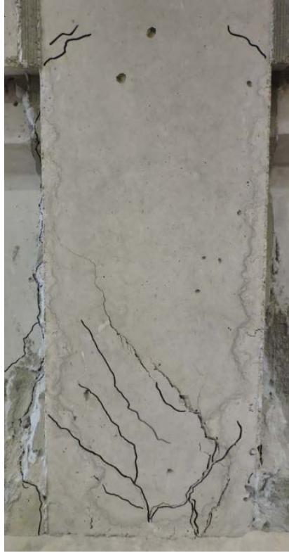
Figure 4-32:R2-J3 Front Joint Face Initial Cracking
