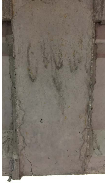
Figure 4-55:R3-PHOS Rear Joint Face Initial Cracking
