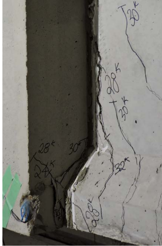
Figure 6-25: R1-FRSCC Girder-Joint Interface Cracking (Front Right)
