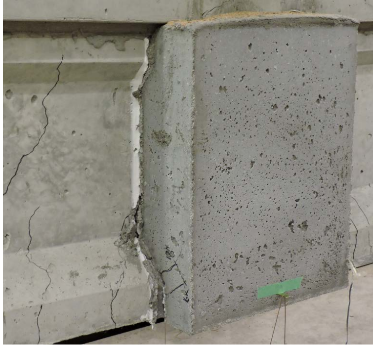
Figure 6-47:R1-PHOS Girder-Joint Interface & Joint Transverse Face Cracking (Front Left)
