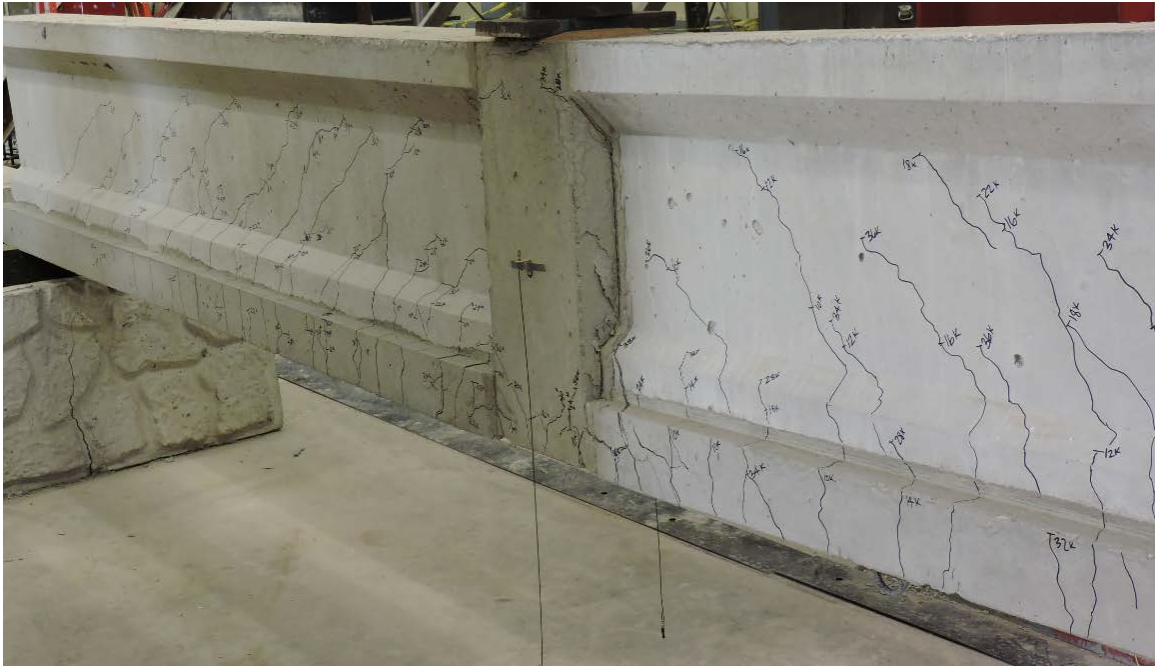
Figure 4-5: C1 Shear Cracking
