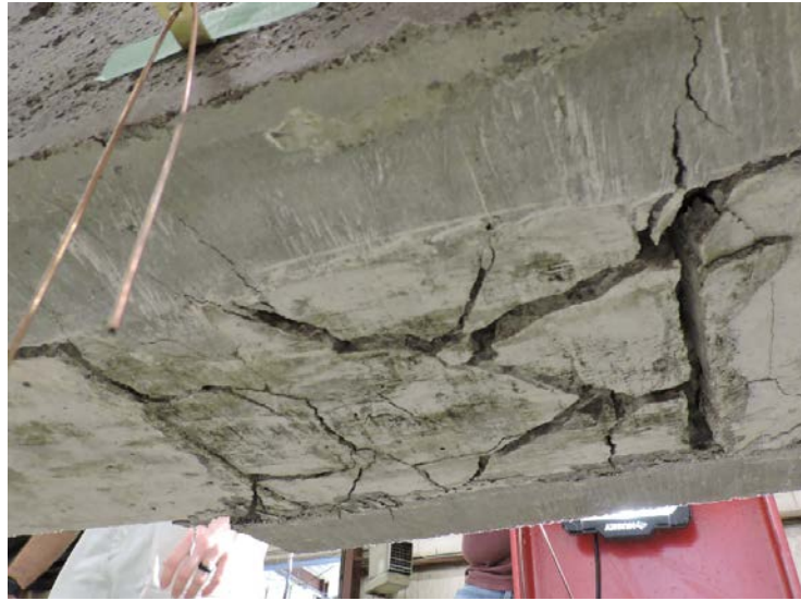
Figure 6-51:R1-PHOS Girder-Joint Separation
