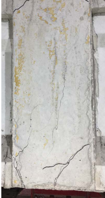
Figure 4-53:R3-PHOS Front Joint Face Initial Cracking
