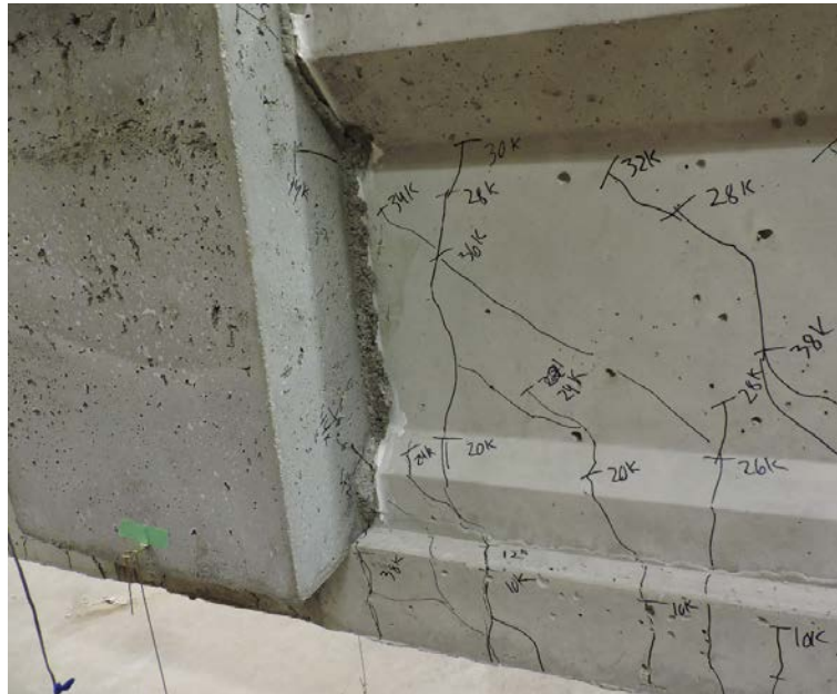
Figure 6-66:R3-PHOS Joint Transverse Face Cracking (Front Right)
