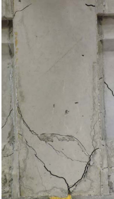
Figure 4-47:R1-PHOS Front Joint Face Initial Cracking
