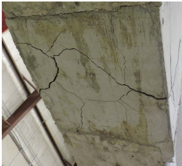
Figure 4-42:R2-FRSCC Bottom Joint Face Initial Cracking
