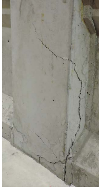
Figure 4-46:R3-FRSCC Rear Joint Face Initial Cracking
