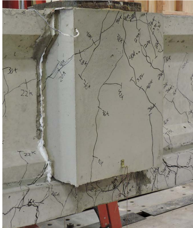
Figure 6-40:R3-FRSCC Joint Cracking, Longitudinal & Transverse Faces (Front Left)
