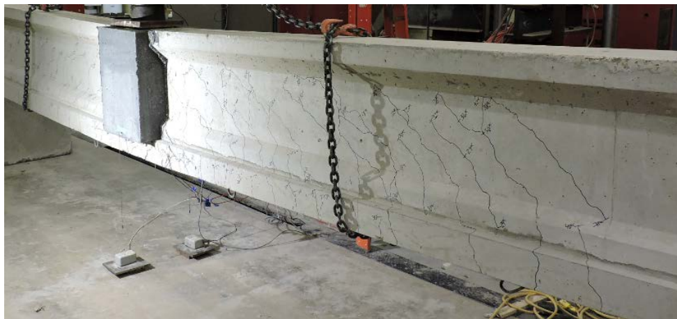
Figure 6-16:R3-J3 Shear & Flexural Cracking
