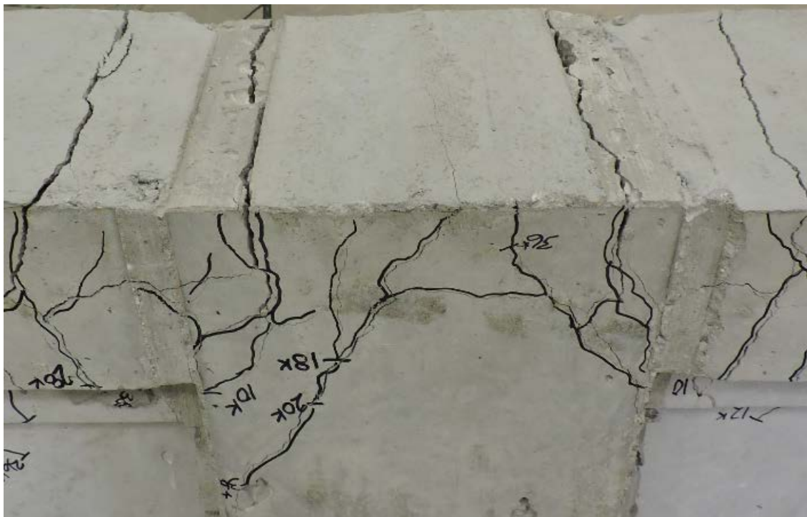
Figure 4-17: C2 Girder-Joint Interface Cracking Across the Deck
