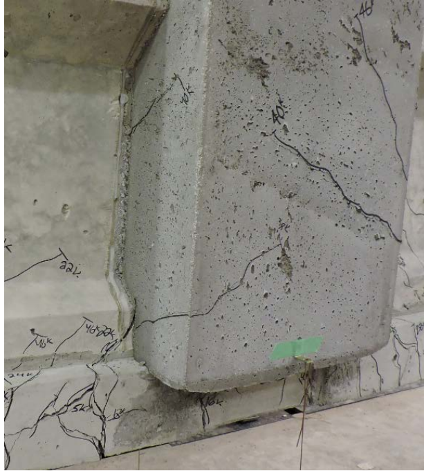
Figure 6-56: R2-PHOS Joint Cracking, Longitudinal and Transverse Faces (Front Left)
