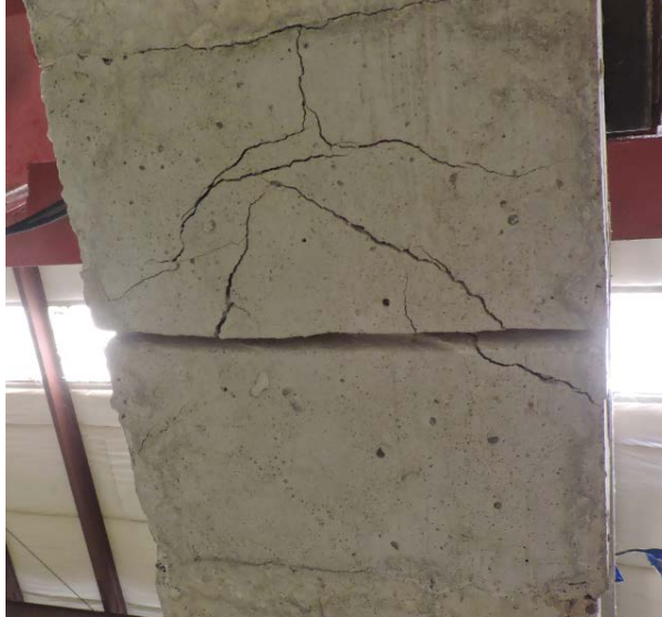
Figure 4-36:R3-J3 Bottom Joint Face Initial Cracking
