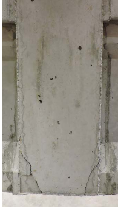
Figure 4-49:R1-PHOS Rear Joint Face Initial Cracking
