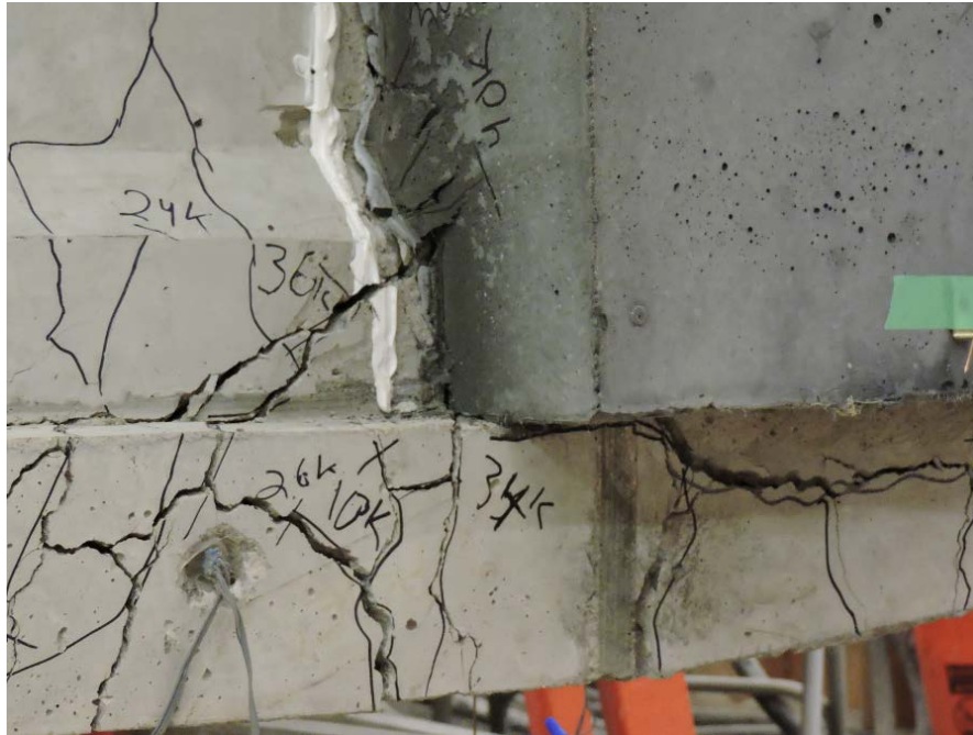
Figure 6-9:R2-J3 Girder-Joint Interface Cracking (Front Left)
