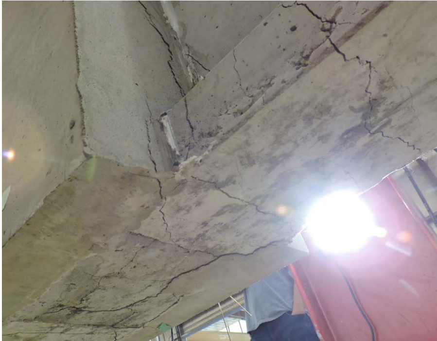
Figure 6-27:R1-FRSCC Flexural Cracking Through Entire Specimen
