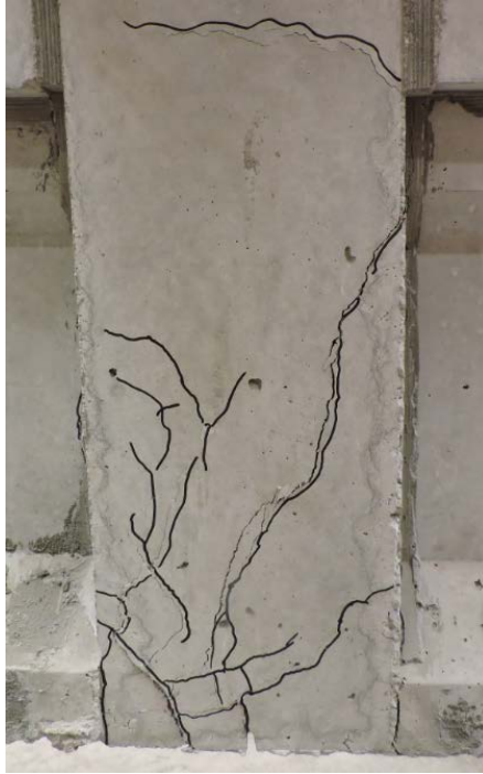
Figure 4-34:R2-J3 Rear Joint Face Initial Cracking
