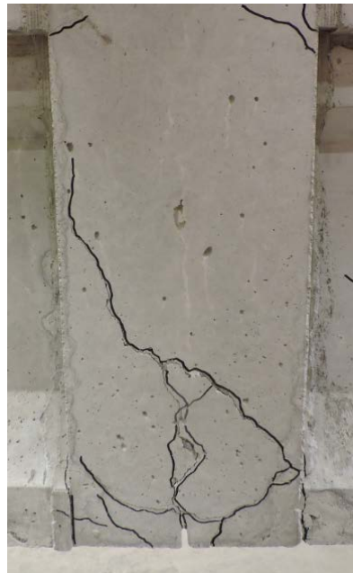
Figure 4-35:R3-J3 Front Joint Face Initial Cracking
