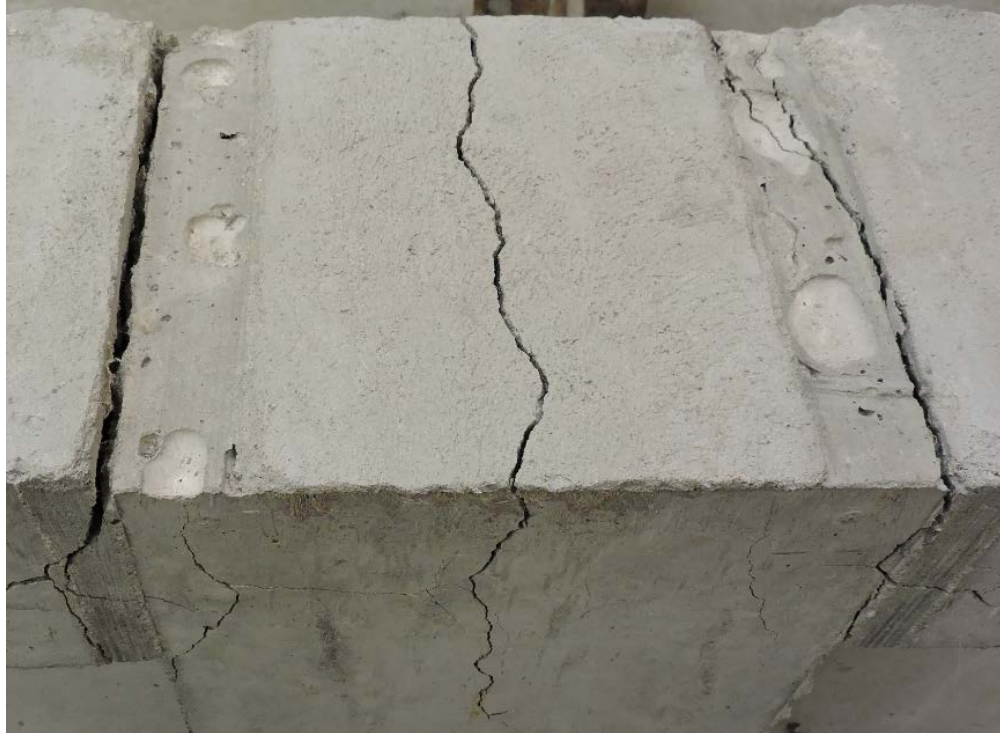
Figure 4-23: C3 Girder-Joint Interface and Centerline Cracking Across the Deck
