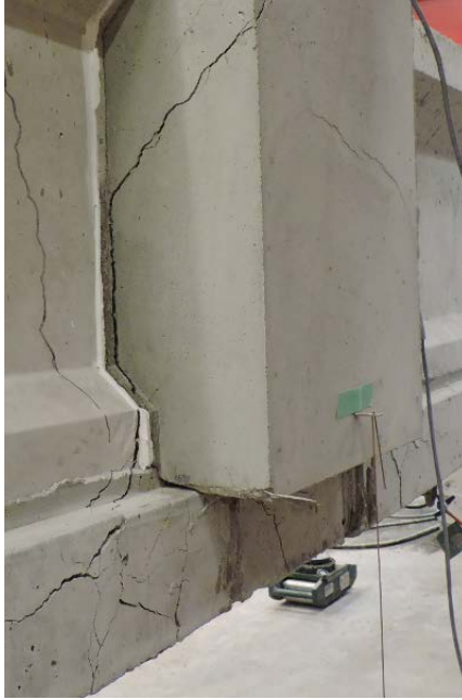
Figure 6-42:R3-FRSCC Joint Cracking, Longitudinal & Transverse Faces (Back Left)
