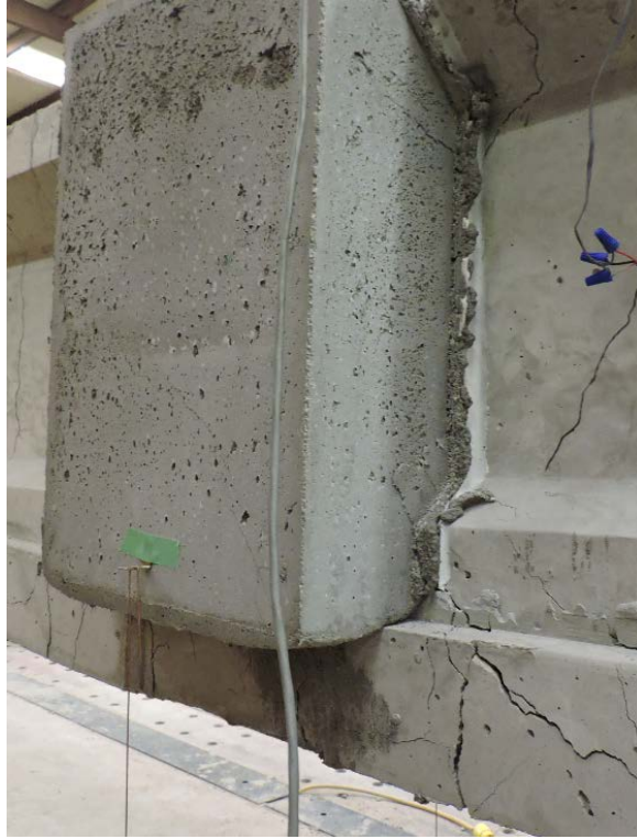
Figure 6-58:R2-PHOS Joint Cracking, Longitudinal and Transverse Faces (Back Right)
