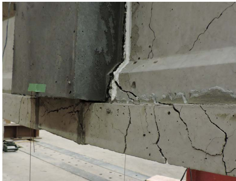
Figure 6-11:R2-J3 Girder-Joint Interface Cracking (Back Right)
