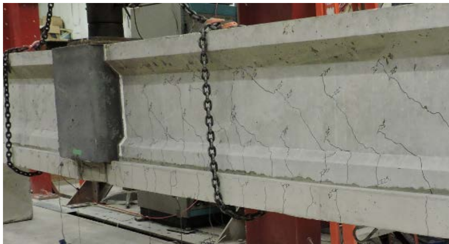
Figure 6-8: R2-J3 Shear & Flexural Cracking
