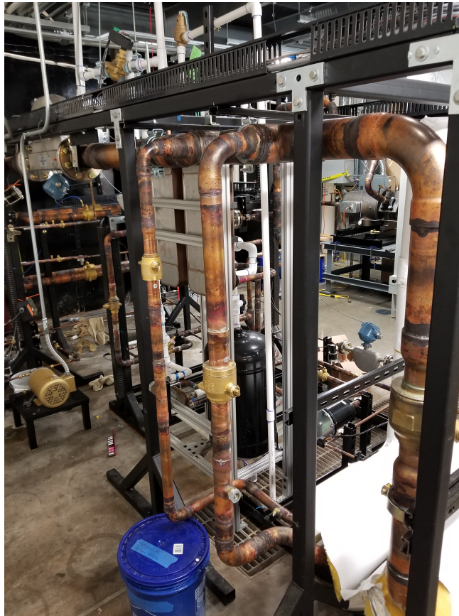
Figure 5.4: Original load stand mixing section
