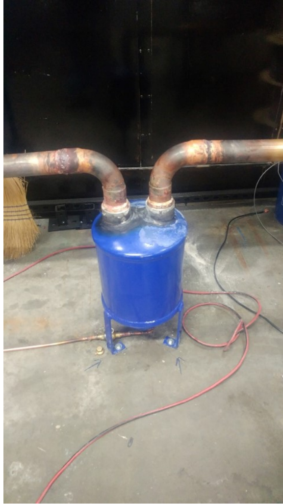
Figure 5.1: Image of the secondary oil separator used with the 30-ton spool compressor conventional separator, while the coalescing separator would catch the rest of the oil that is carried over.
