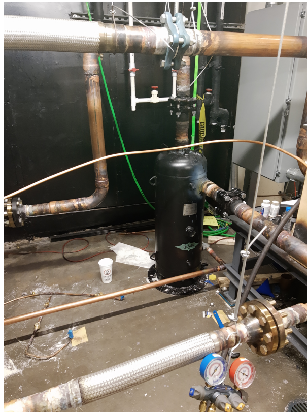
Figure 6.3: Bitzer OA4188US centrifugal separator installed upstream of the coalescing separator.
