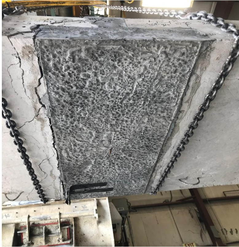
Figure 58: Cracks on the as-tested underside of Ductal® slab 2 after testing
