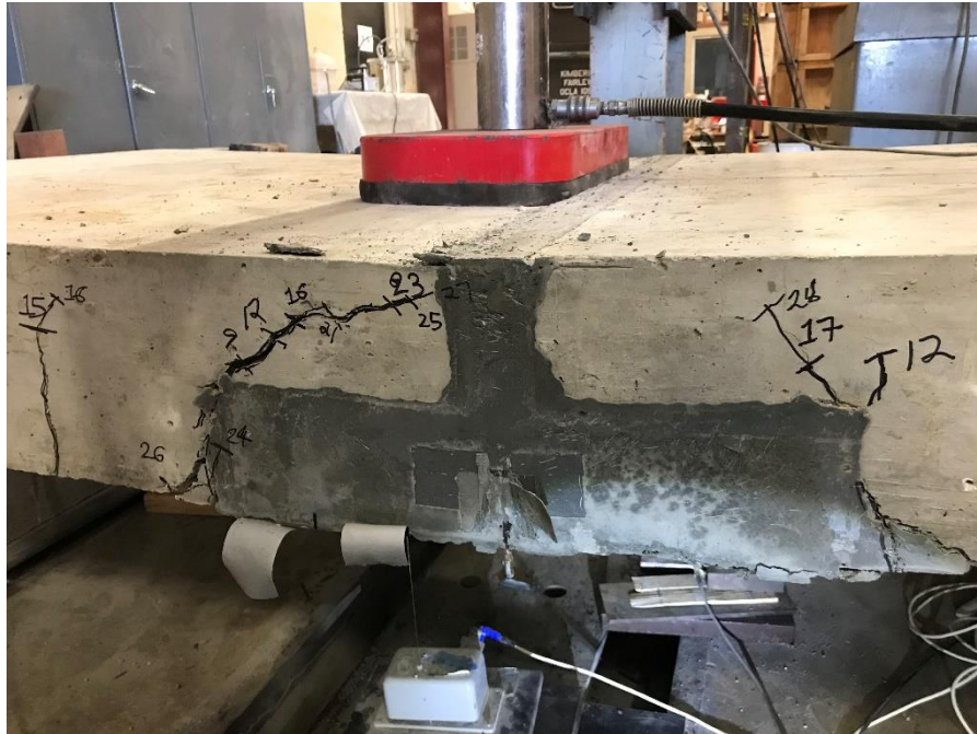
Figure 45: Large cracks at the conventional concrete to UHPC interface after part 1 of testing
