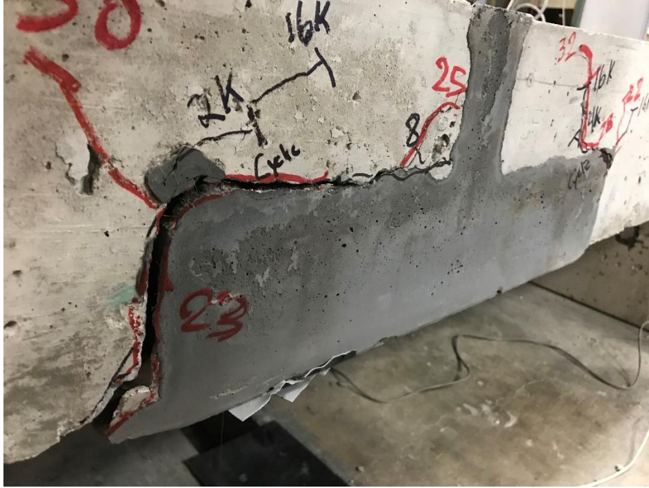
Figure 39: Cracks formed at the conventional concrete to UHPC interface on the north side of J3 slab 2
