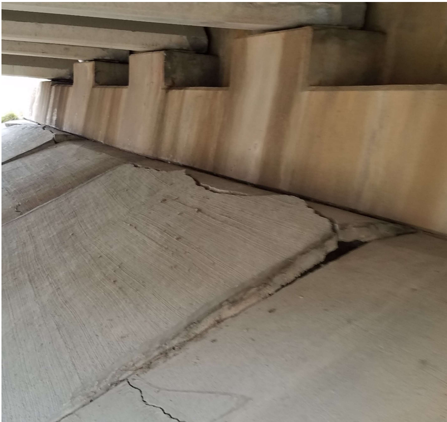
Figure 47. SH-3 Ada, OK - Buckled Slope Wall
