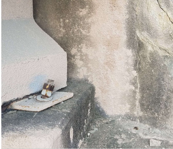
Figure 46. SH-3 Ada, OK - Rotated Anchor Bolt
