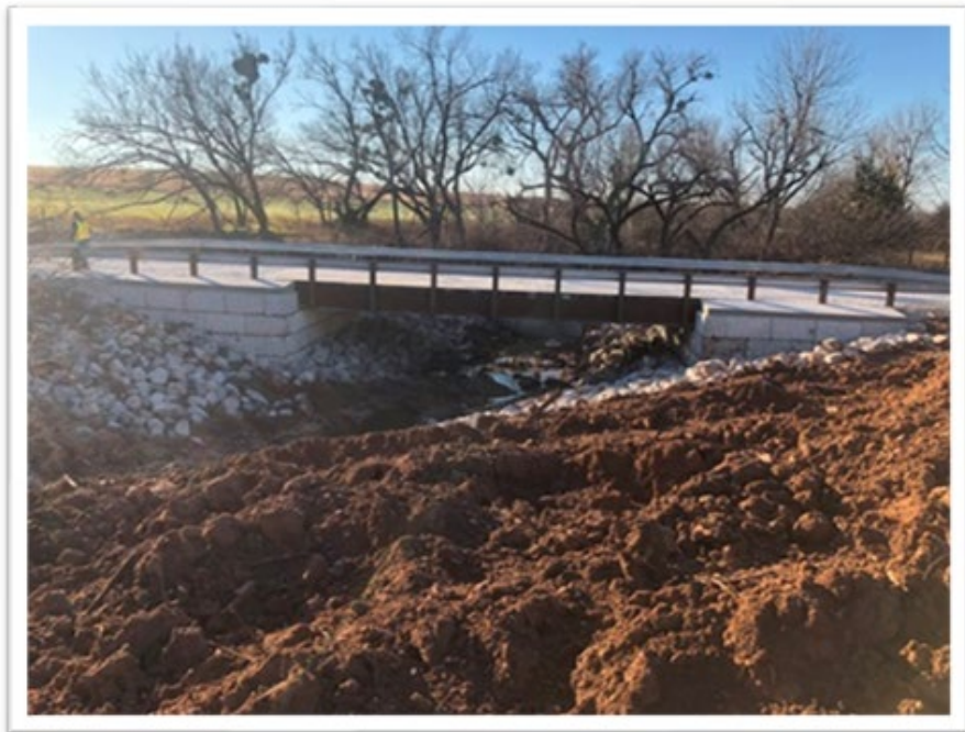
Figure 22. Recently constructed Little Washita River (Large block facing) GRS-IBS in Caddo County, OK
