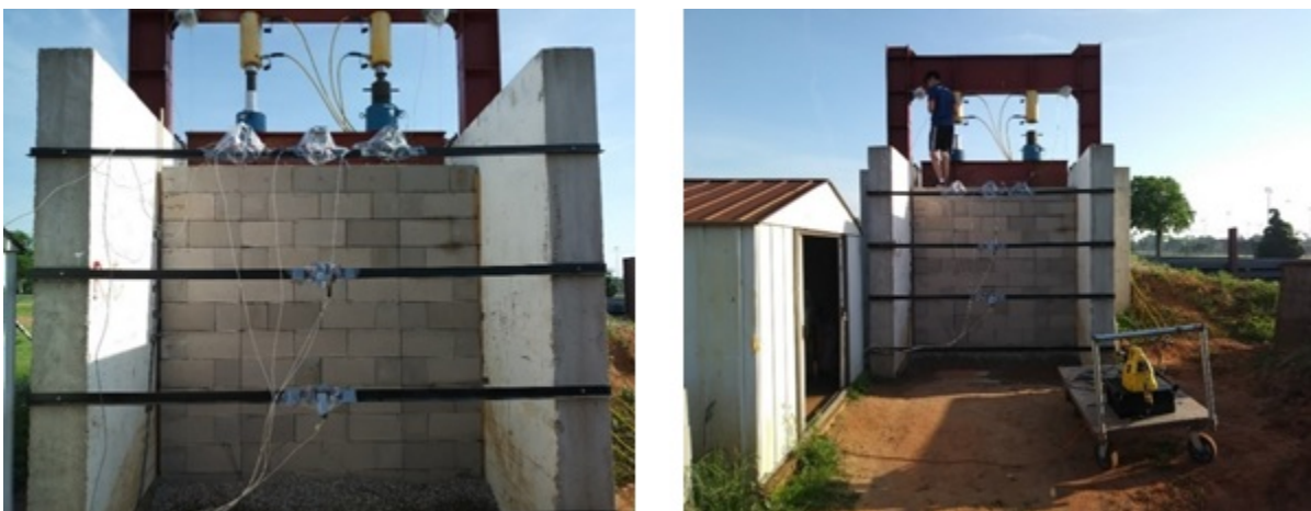
Figure 8. (Left) Wire extensometers are attached to the facing of GRS Abutment Model #1 to measure its deformation at three different levels; (Right) Electric-hydraulic pump is attached to the loading assembly before the start of loading test
