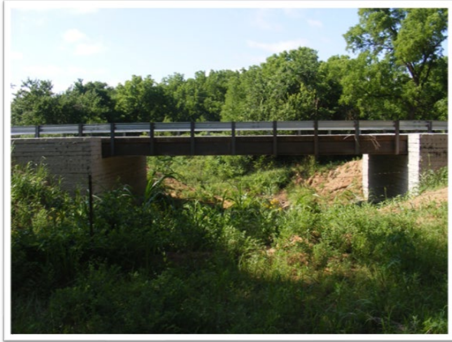
Figure 21. Recently constructed Two Hatchet Creek (CMU block facing) GRS-IBS in Caddo County, OK
