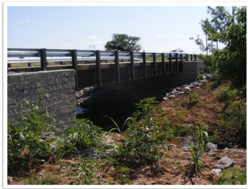
Figure 20. Recently constructed East Cache Creek (CMU block facing) GRS-IBS in Caddo County, OK
