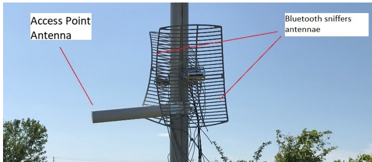
Figure 46. Access point antenna on the pole.
