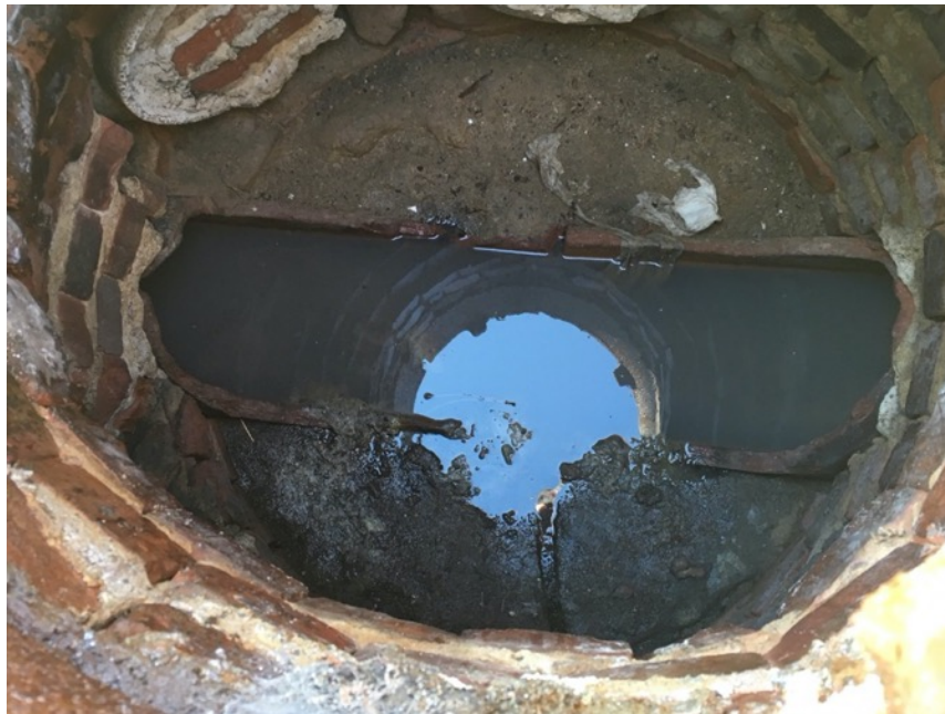
Figure 10. Shallow manhole used to obtain grab sample SC 73. The manhole was located one-half block upstream from the location where SC 57-69 were collected.
