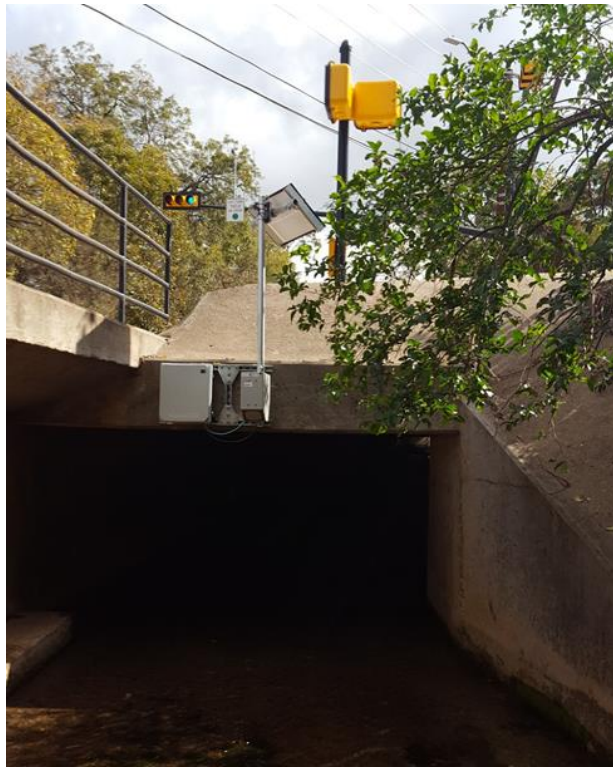
Figure 13: Stream radar mounted on culvert at Sessom Creek
