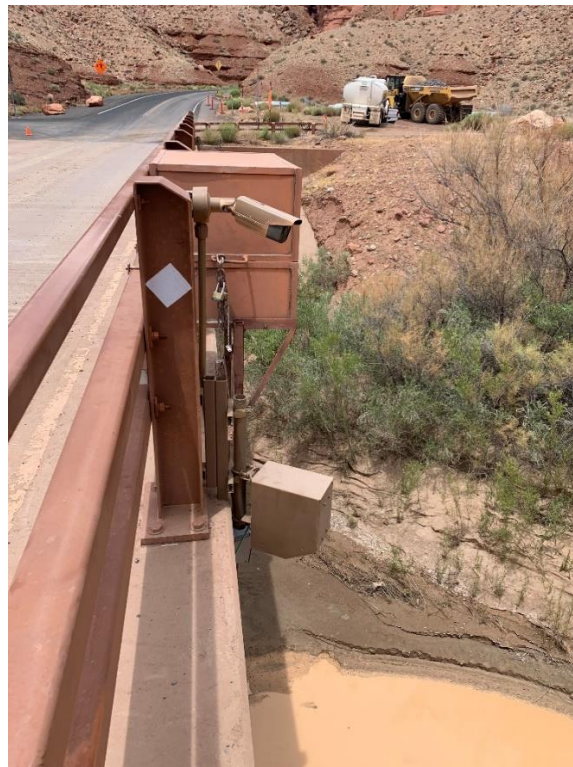
Figure 9: Stream radar mounted on bridge at Paria River
