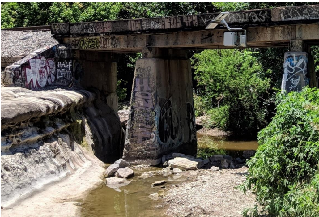
Figure 17: Stream radar mounted on bridge at Austin South
