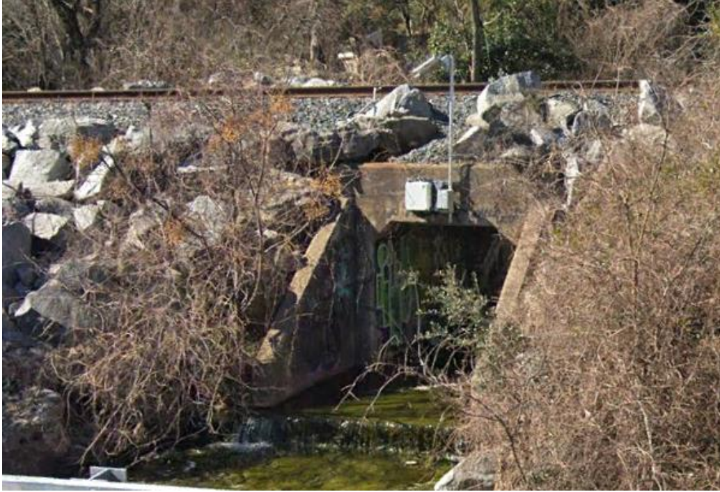
Figure 15: Stream radar mounted on culvert at Austin North (source: Google Earth Pro)
