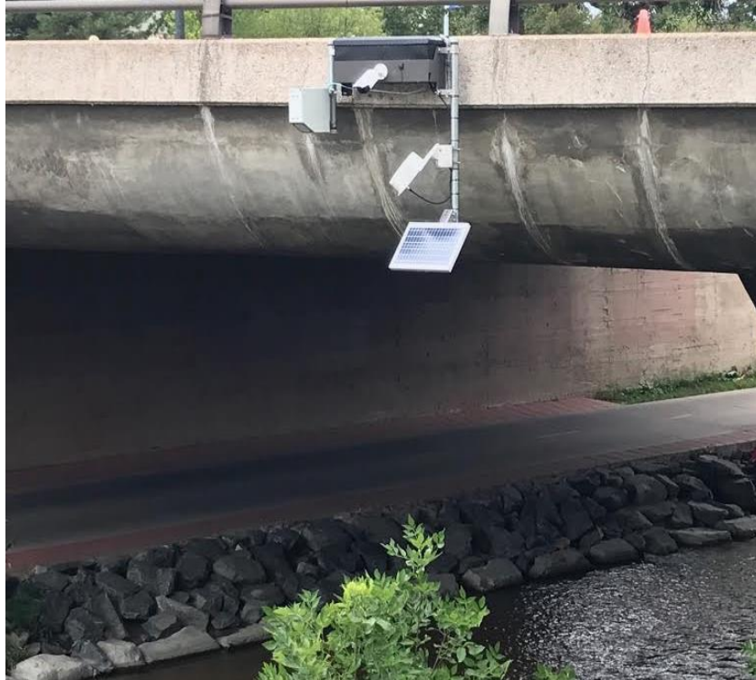
Figure 3: Stream radar mounted on bridge at Cherry creek
