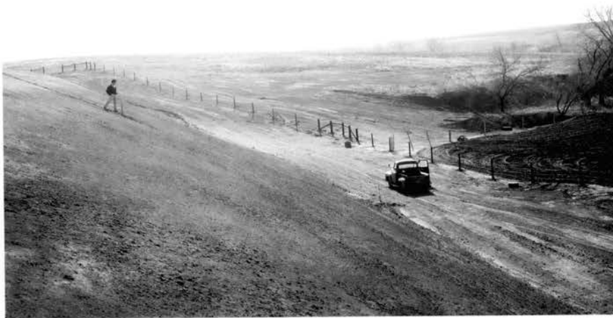
Figure 22. Back (2:1) slope of Site 34 after completion of the embankment showing the relative location of Gages Nos. 4 and 5 and Relief Wells Nos. 1 and 2.
