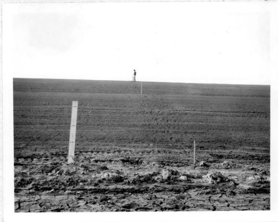
Figure 20. Gages Nos. 1, 2 and 3 on Site 3 4 shown after the completion of the embankment.
