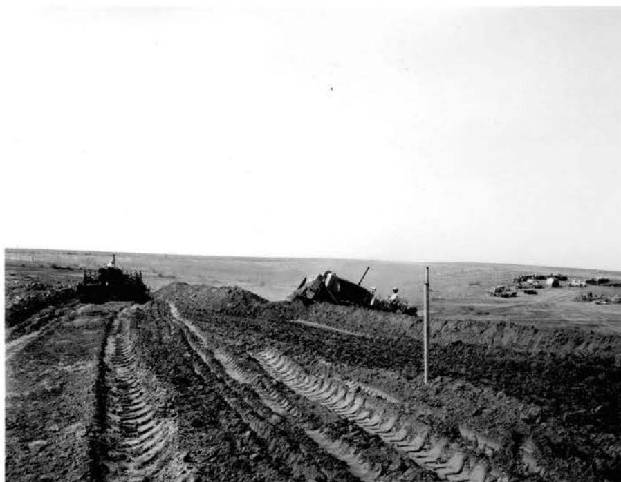
Figure 12. Gage pipes 3 and 6 on Site 34 shown two days before the embankment was completed.
