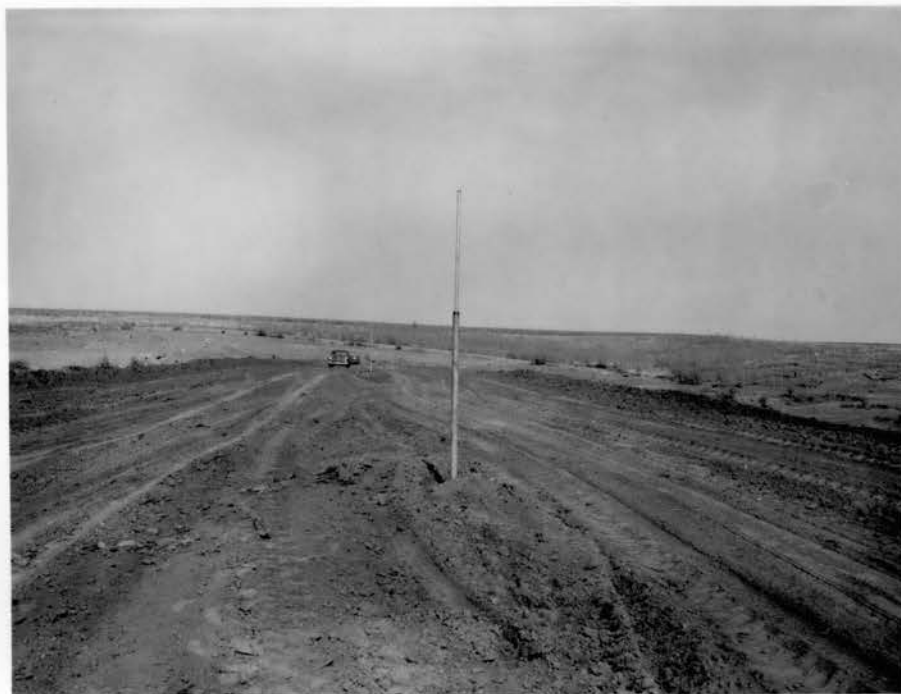
Figure 11. Gage pipes on Site 34 showing relative location of Gages Nos. 3 and 6. (No. 6 is by the open door of the car.)
