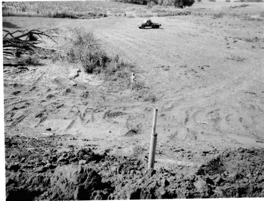
Figure 21. Site 34. View showing Gages Nos. 4 and 5 during construction of dam. The man is standing by Relief Well No. 1.
