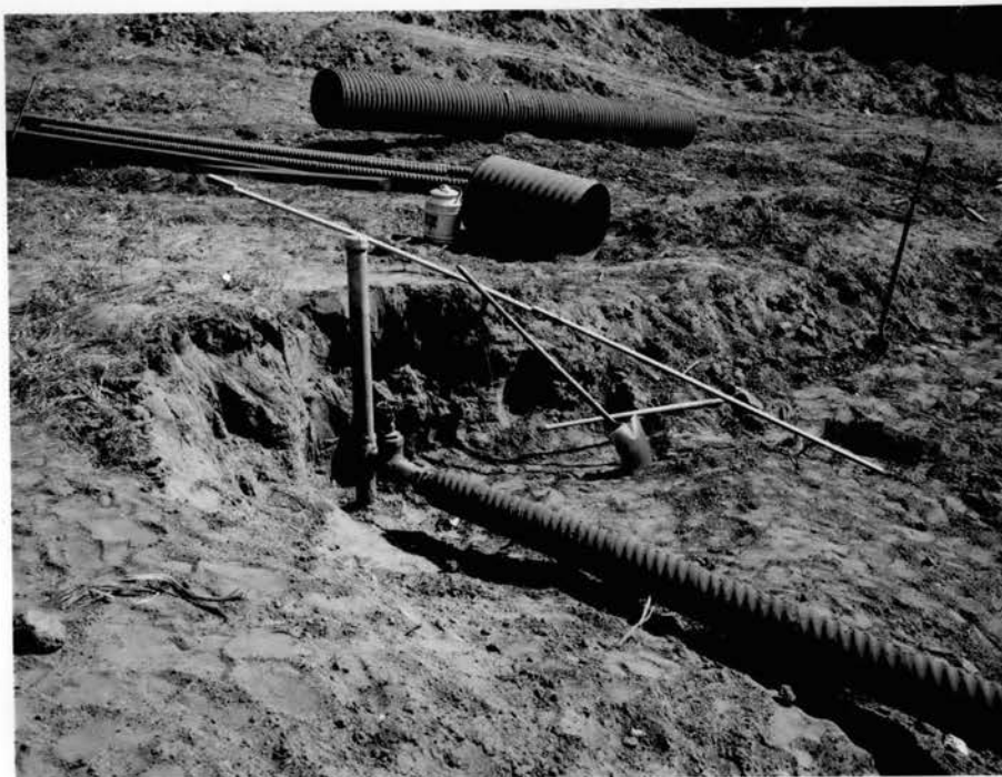
Figure 7. Relief Well No. 1 - Site 34. Remaining steps: Installing well cover and covering collector line with earth.
