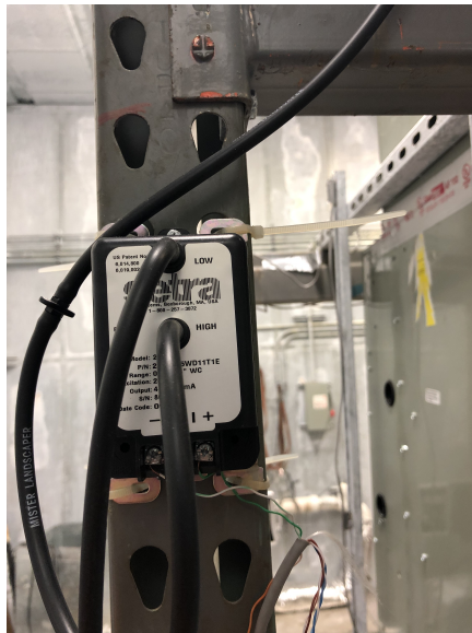
Figure A.15: Setra differential pressure transducer (unit side)
