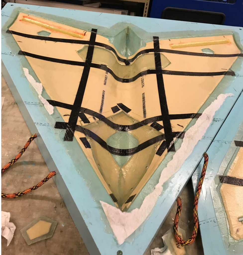
Figure 84: Top skin after layup but before removal. Hatches can be seen under skin
