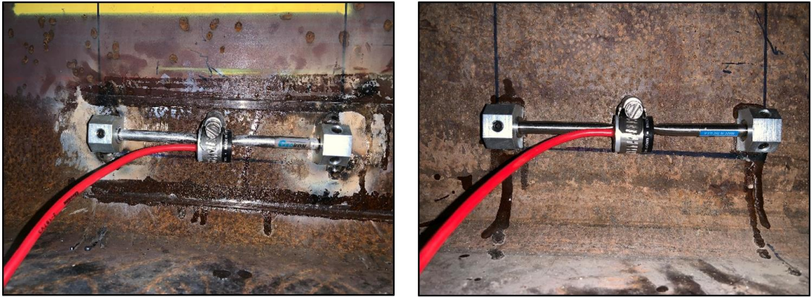
Figure 24. Geokon model 4000 VWSGs welded and glued to the steel beam of the prototype bridge
