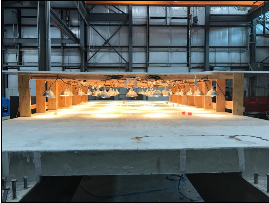
Figure 77. Photograph showing the setup of Heat lamps atop the prototype bridge deck
