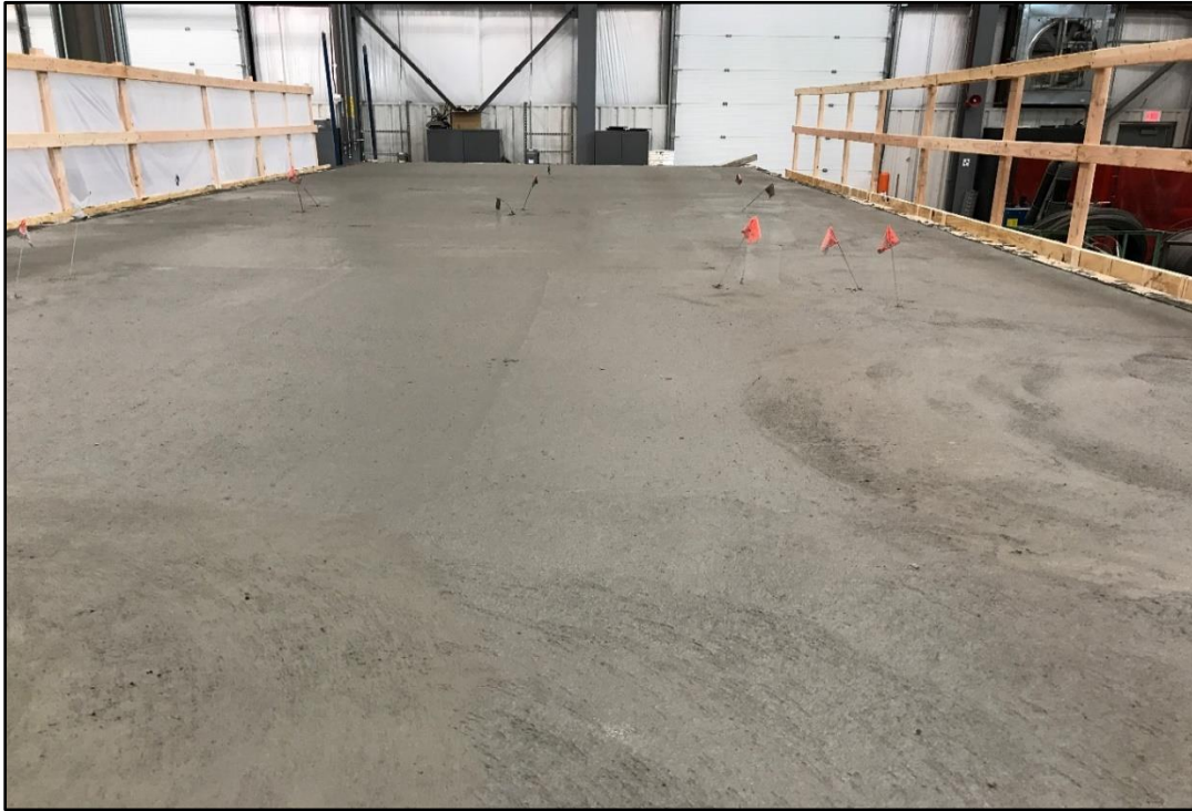
Figure 52. Bridge deck after casting and finishing concrete. A broom finish was applied.
