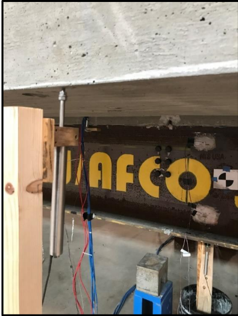
Figure 49. Installation of LVDT sensors at the midspan location of South Girder (LVDT 3) and South edge of slab overhang (LVDT 4)
