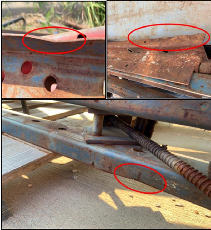
Figure 40. C-49 Overhang brackets with warped and permanently deformed sections
