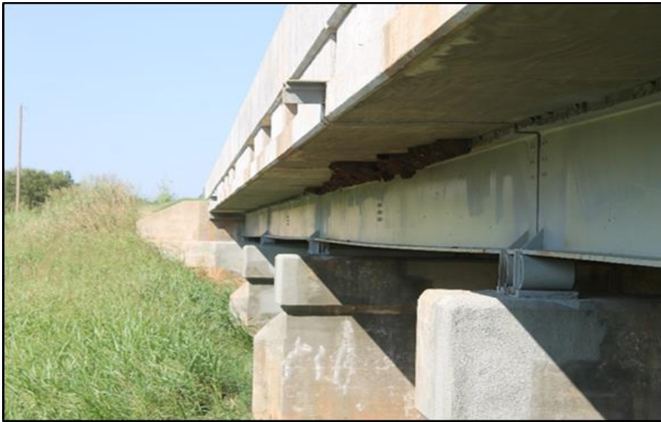
Figure 45. Eagle Chief Creek Bridge “A” on SH 14, Woods Co., OK. View looking North.
