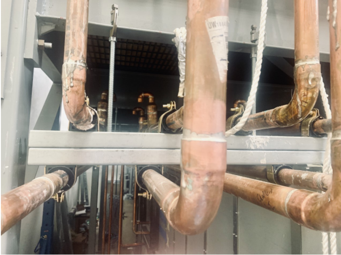
Figure 5.3: This is a view of the piping supports located on the side of the airside facility.
