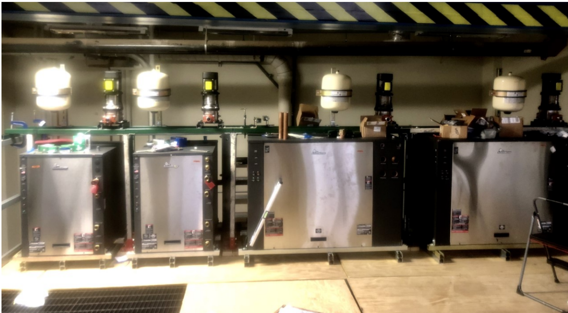
Figure 2.5: The placement and location of the heat pumps.
