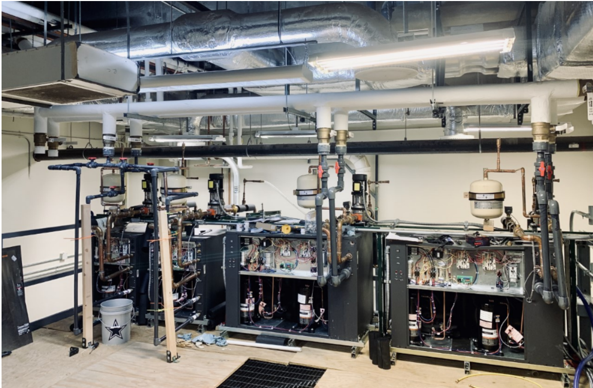
Figure 5.5: The heat pumps are connected to the lab chilled water via PVC as seen here, please note the wood supports are temporary.
