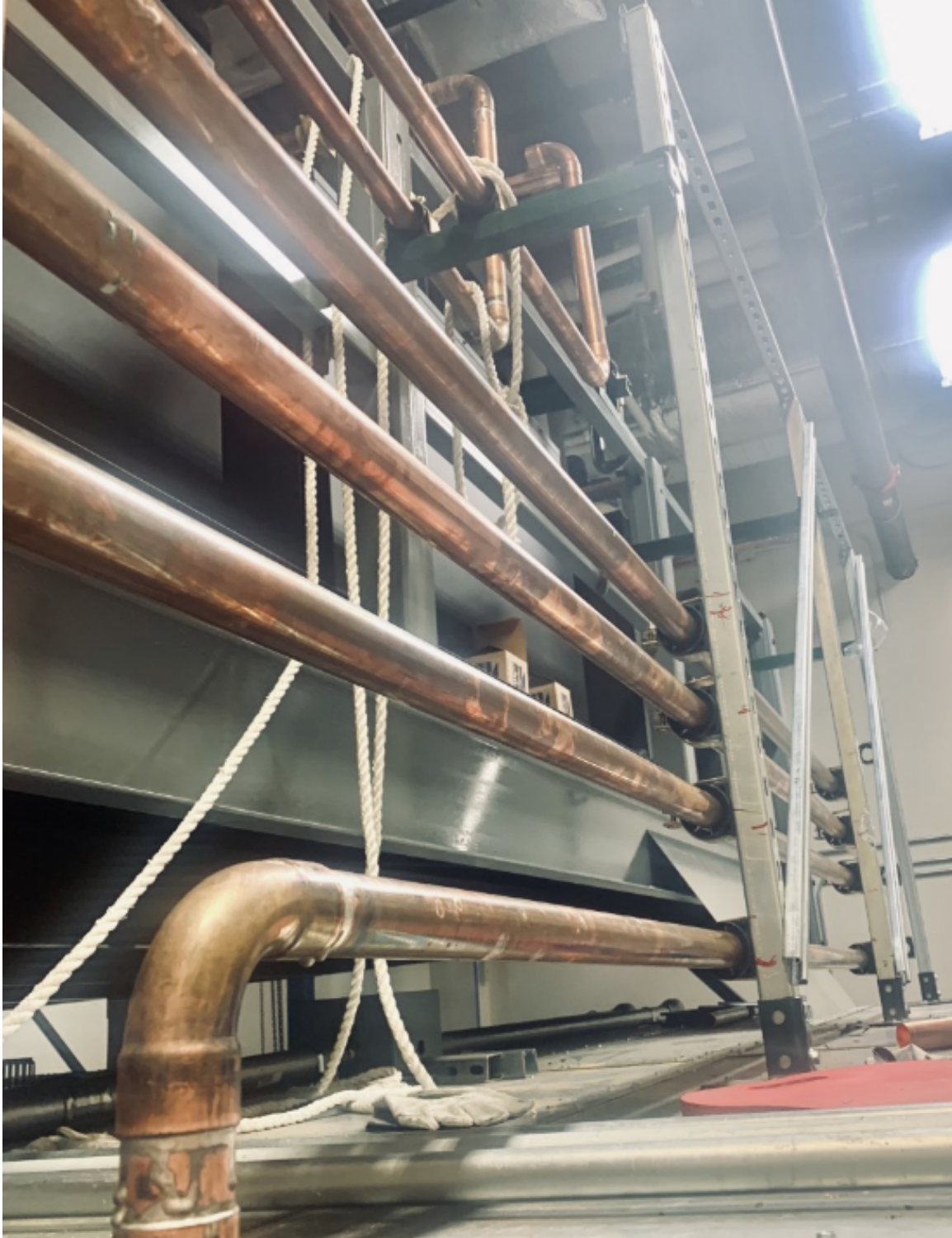
Figure 5.2: This is a view of the piping supports located on top of the airside facility.
