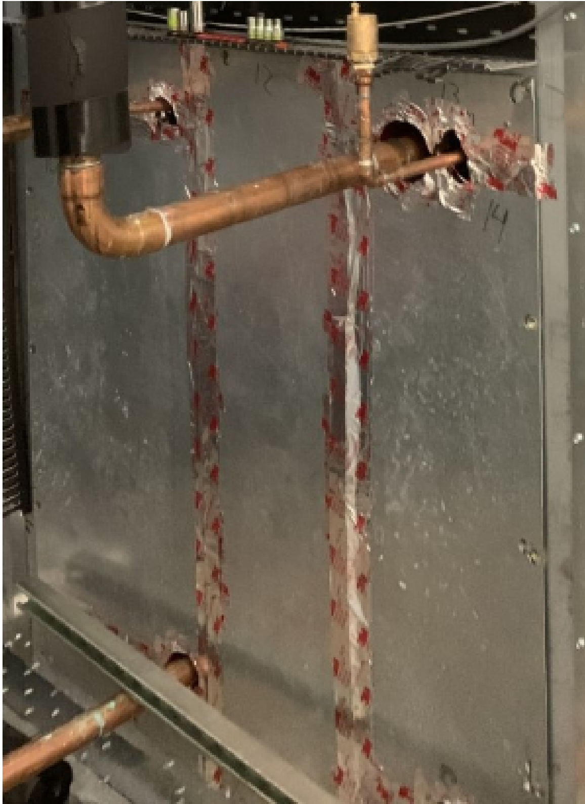
Figure 5.4: Holes were cut into the access panels to allow them to still be easily removable.
