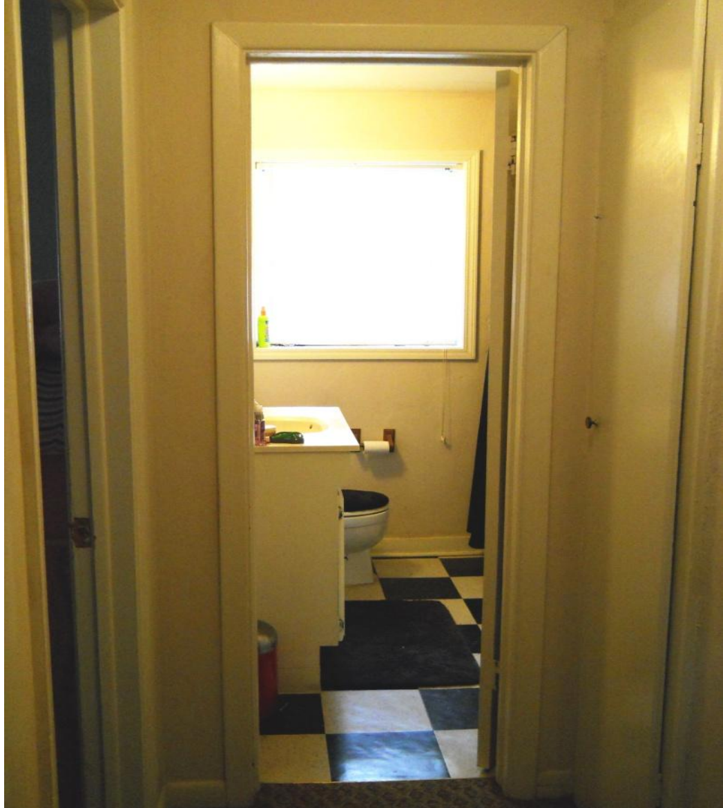
Figure 13: Photograph of bathroom showing assessment instrument violations due to a lack width to enter the space, the lack of floor space to maneuver safely, and the presence of a slippery floor begin the list of violations
