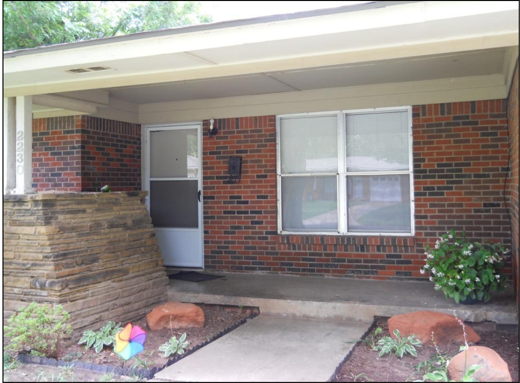
Figure 5: Photograph of front porch illustrating assessment instrument violations of a front step, an elevated mailbox, insufficient lighting, lack of access to the front entry, lack of furniture for placing items when accessing the front entry, an unusable planter and a deficiency in providing visitability conditions
