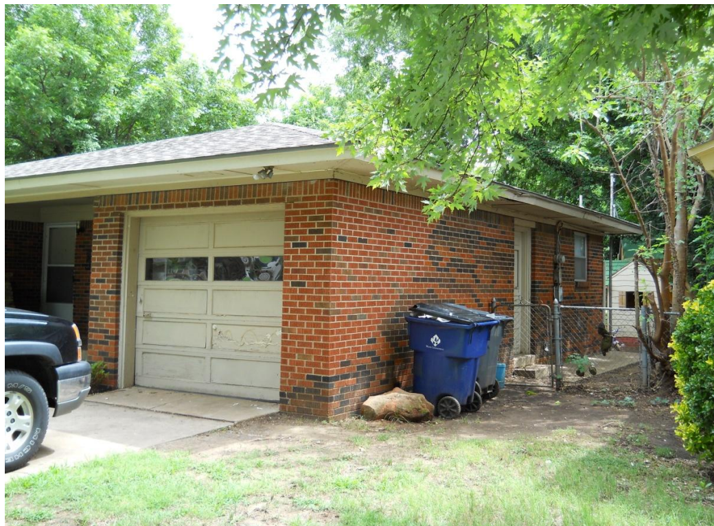
Figure 2: Photograph of west side of property illustrating assessment instrument violations due to a narrow sidewalk and the lack of a sidewalk necessary for backyard access
