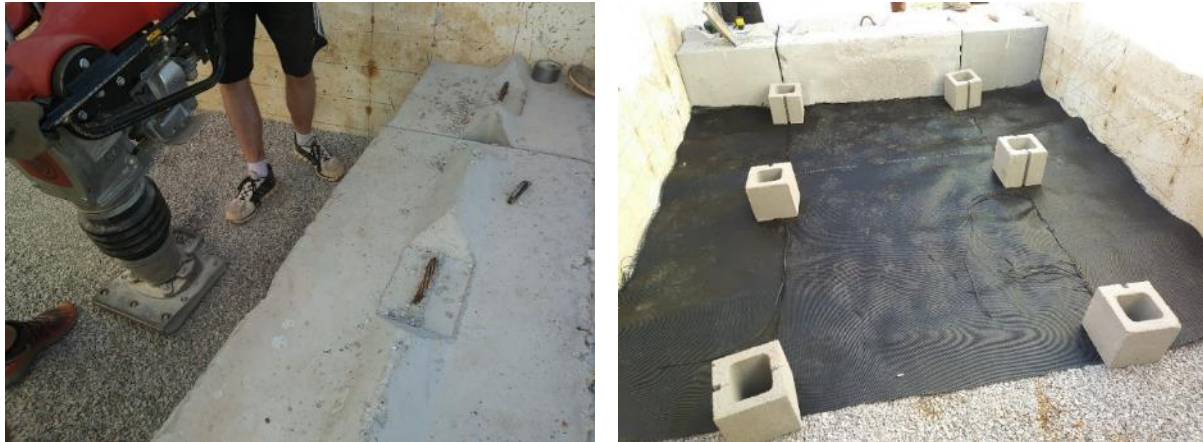
Figure 52. (Left) Compaction of the GRS bridge abutment fill behind the first-row of large concrete blocks; (Right) Installation of the first geotextile layer
