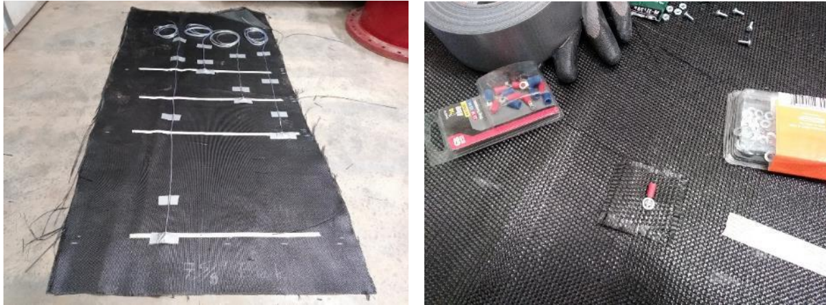
Figure 15. (Left) WP connections at 75-inch level reinforcement layer; (Right) WP connections on the geotextile reinforcement
