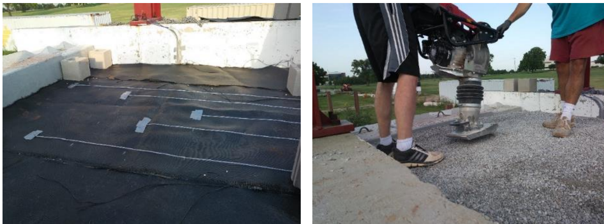
Figure 54. (Left) Installation of the top geotextile reinforcement layer at Elevation 91-inch above the foundation slab; (Right) Compaction of final aggregate lift using a Jumping-Jack compactor
