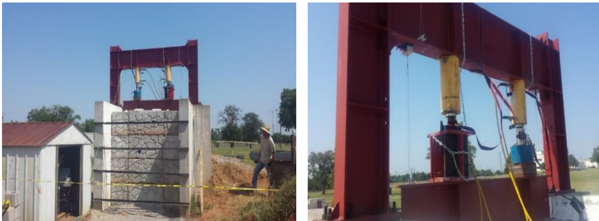
Figure 55. (Left) Front view of safety precautions for surcharge load testing of GRS Abutment Model #2; (Right) Back view
