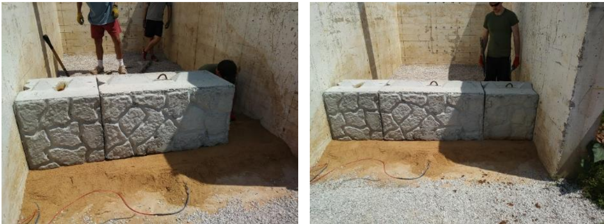
Figure 51. (Left) Installing the second large concrete block of the first-row; (Right) Third large concrete block
