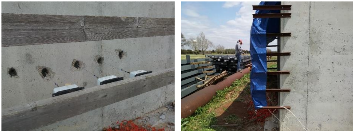
Figure 37. (Left) WPs at the back of test box; (Right) WP protection measures
