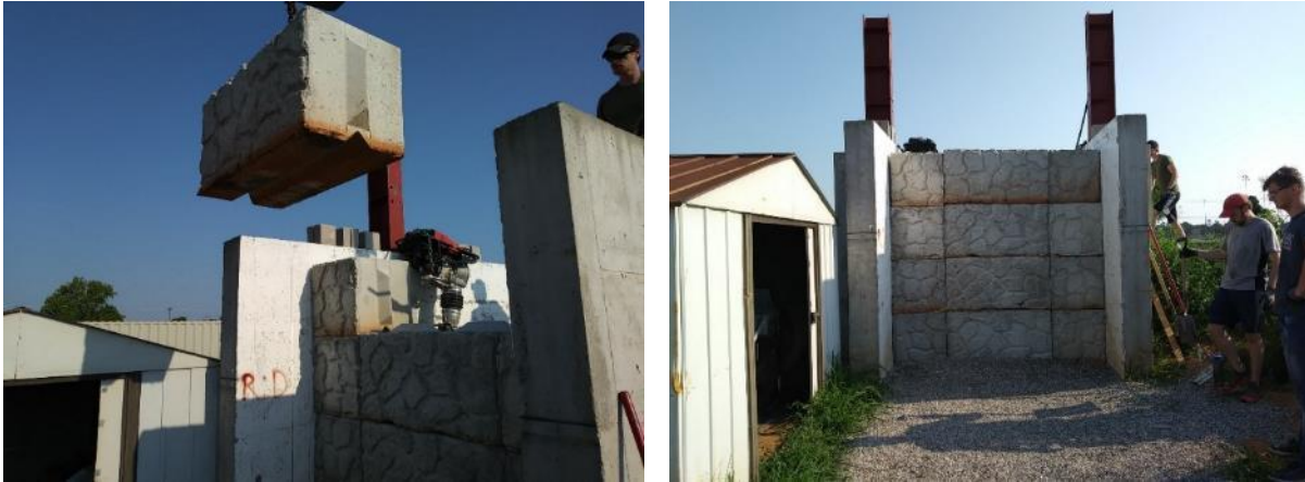
Figure 53. (Left) Installation of the top (forth) row of large concrete block facing; (Right) The subsequent elevation view of the GRS bridge abutment
