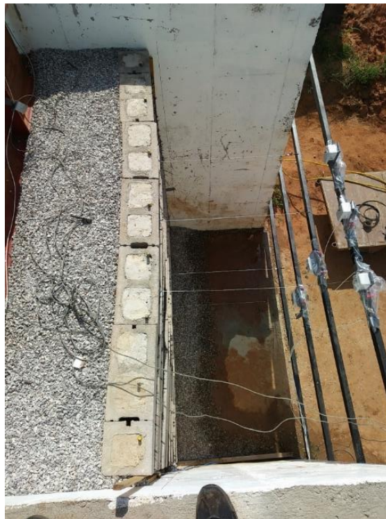
Figure 83. Facing deformation of GRS Abutment Model #1 at the end of surcharge load testing
