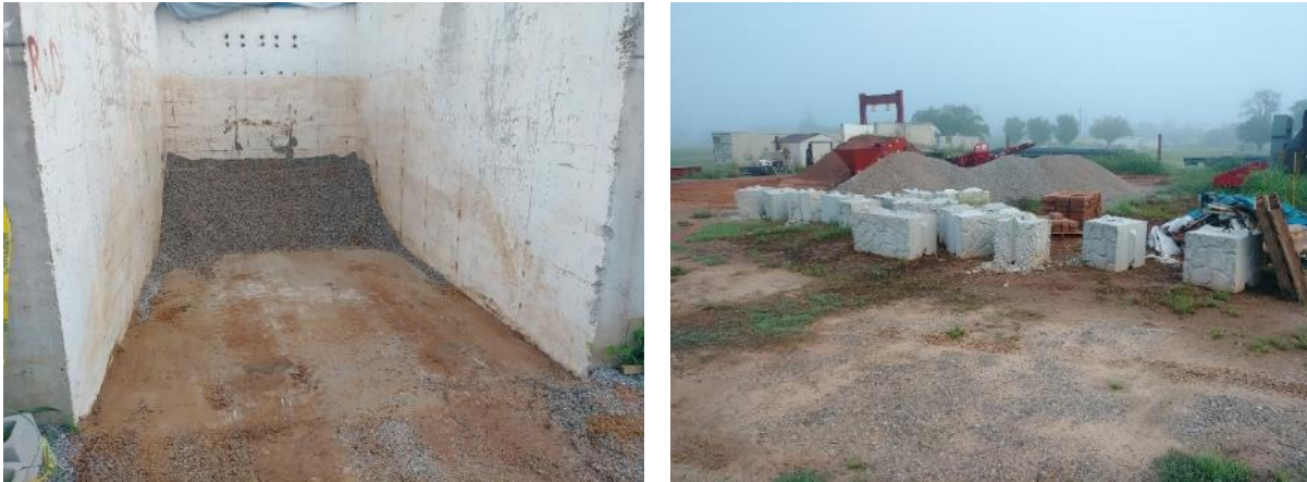
Figure 67. (Left) Test box after excavation and removal of GRS Abutment Model #2; (Right) Fill gravel and large concrete block storage area for the construction of GRS Abutment Model #3
