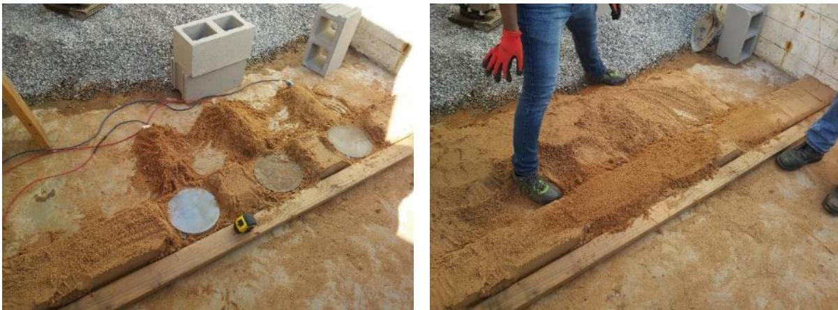
Figure 32. (Left) Installation of the first three EPCs under the CMU blocks before covering with sand; (Right) After covering with sand
