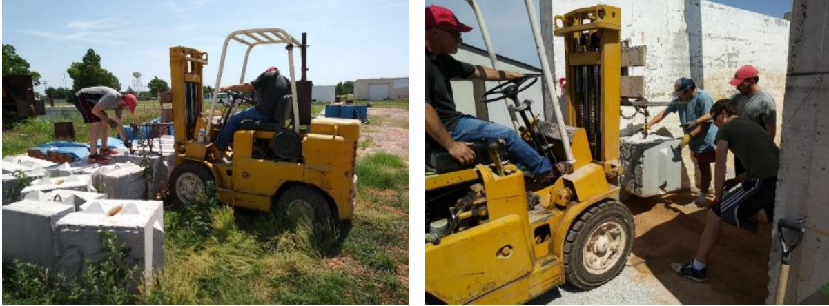
Figure 50. (Left) Transporting the large concrete blocks in the test box; (Right) Placing them
