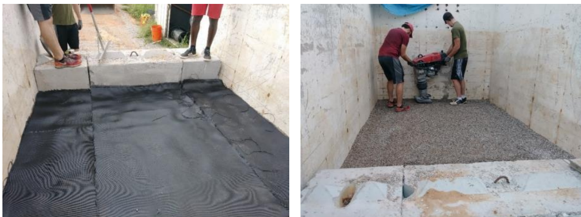
Figure 58. (Left) Installation of the first reinforcement layer in GRS Abutment Model #3; (Right) Compaction of the GRS fill at every 12-inch lift
