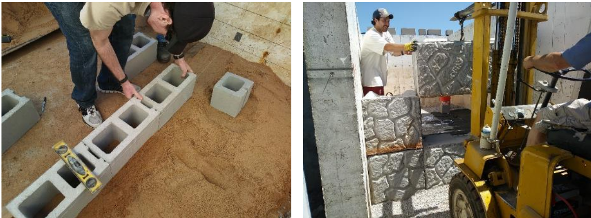
Figure 18. (Left) Manual placement of CMU facing blocks; (Right) Placement of large concrete blocks using a forklift
