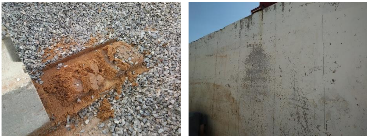
Figure 64. (Left) Settlement of sand layer underneath CMU blocks; (Right) Scratch marks on the painting of the east sidewall indicating the pressure bulb
