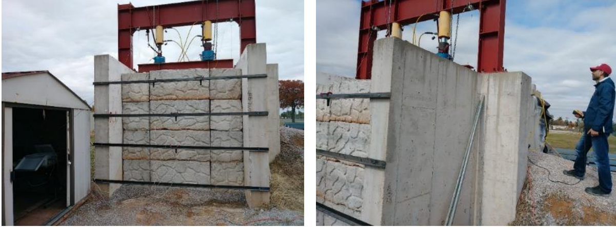
Figure 59. (Left) Front view of fully constructed GRS Abutment Model #3 before the start of surcharge load testing; (Right) Controlling the electric hydraulic pump during surcharge load testing
