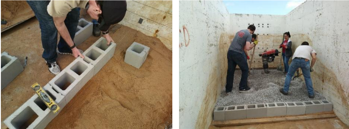
Figure 33. (Left) Placement of the first-row of CMU blocks; (Right) Placement of backfill lift
