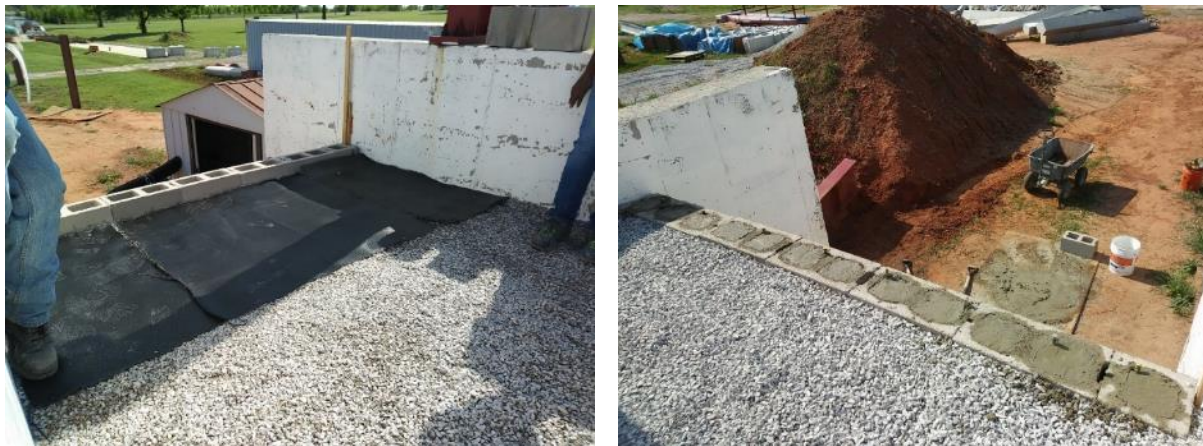
Figure 40. (Left) Placement of the reinforcement layers for shallow footing under the loading beam; (Right) Connecting the top three CMU blocks using concrete and rebar as per the FHWA guidelines
