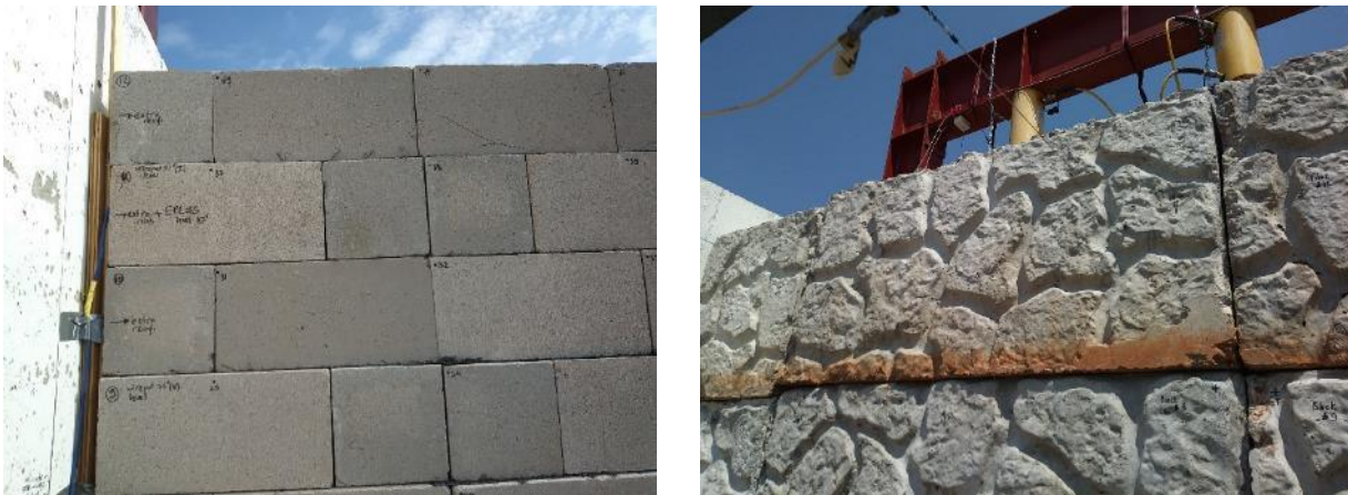
Figure 7. (Left) Reference points on CMU blocks for manual reading of facing deformations; (Right) Large concrete blocks
