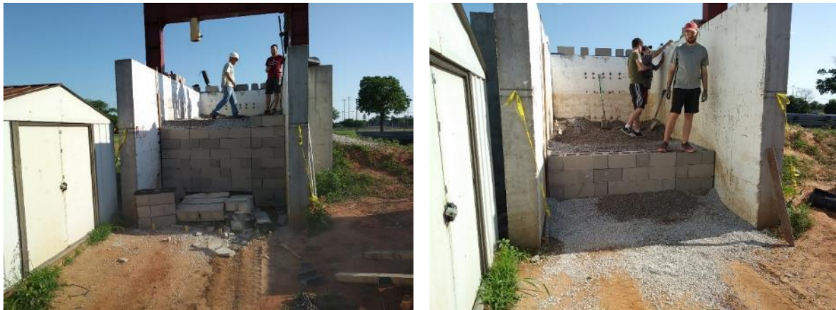
Figure 63. (Left) Demolition of the top three rows of CMU blocks; (Right) Final stages of GRS fill excavation from the test box
