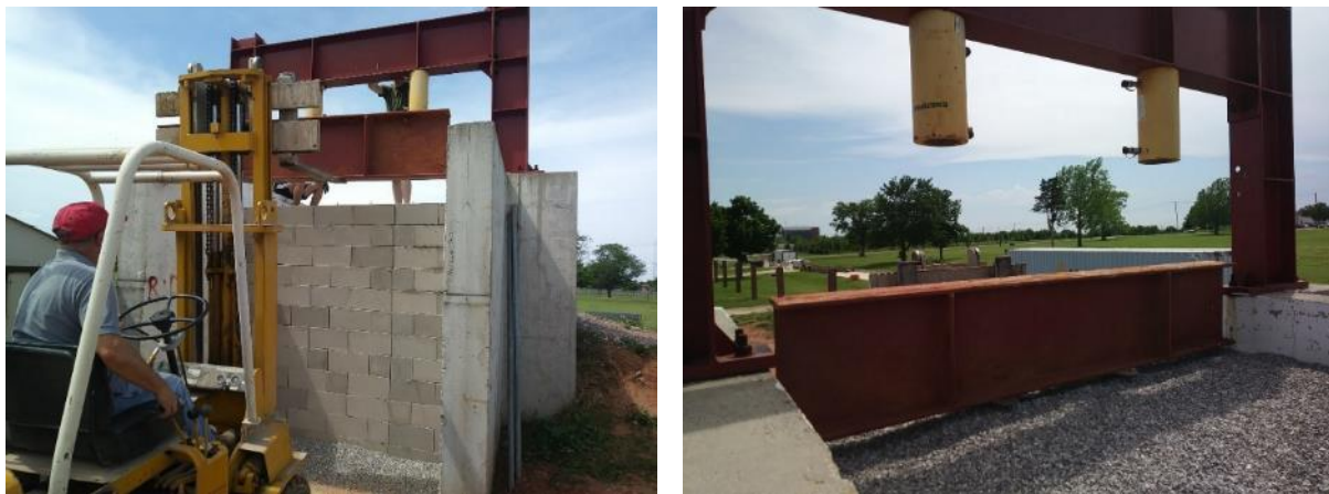
Figure 43. (Left) Front view of the installation of the loading beam under the hydraulic pistons; (Right) Back view
