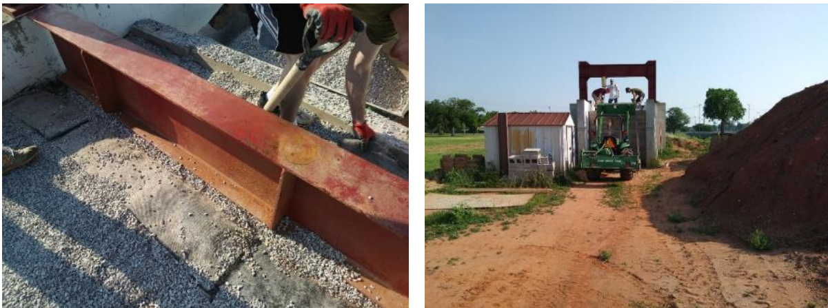
Figure 60. (Left) Initial stages of the deconstruction of GRS Abutment Model #1; (Right) Front view of the test station during deconstruction
