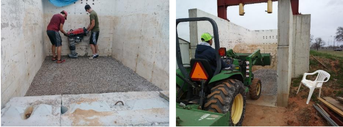
Figure 19. (Left) Compaction of GRS fill; (Right) Placement of the fill inside the test station
