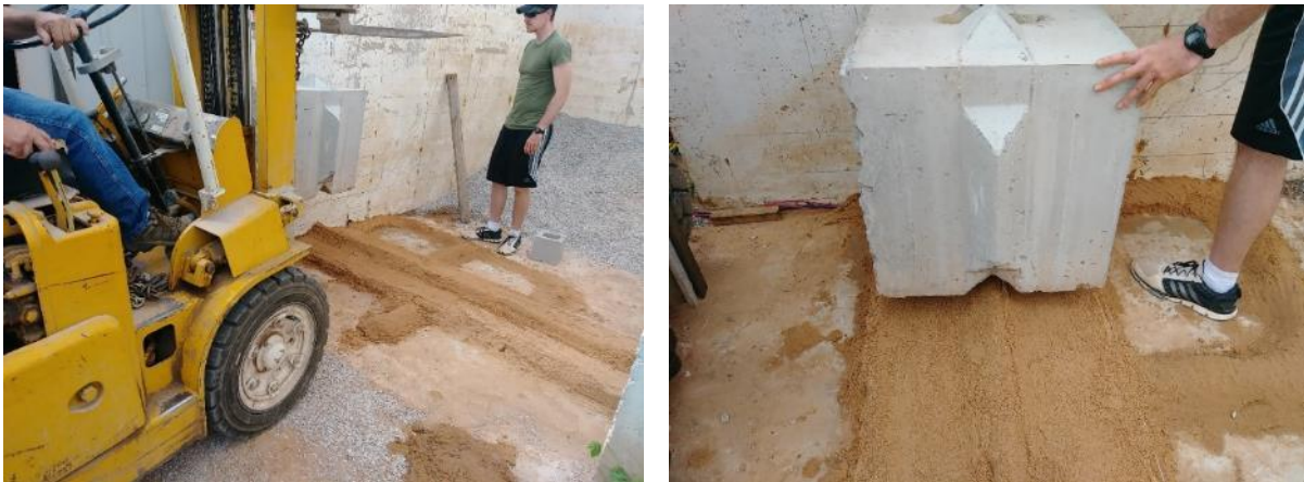
Figure 57. (Left) Front view of the installation of the first-row of facing blocks in GRS Abutment Model #3; (Right) Side view
