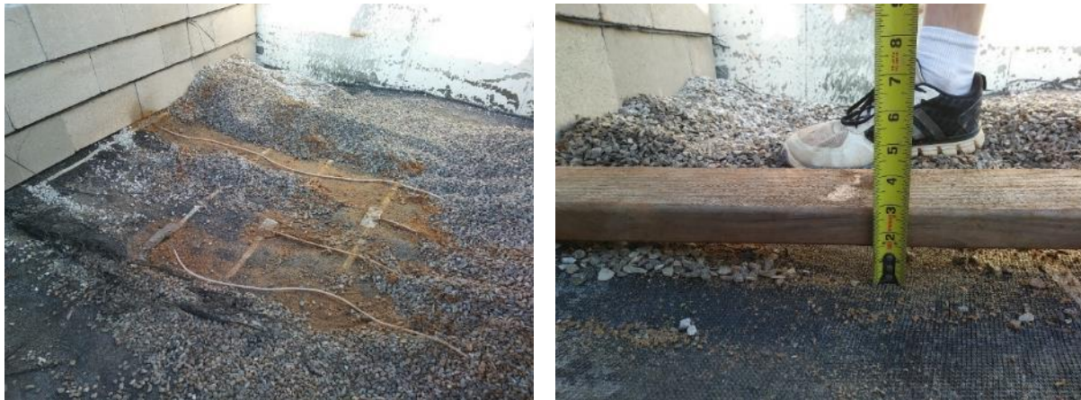
Figure 62. (Left) An exhumed instrumented geotextile reinforcement layer after the load test; (Right) Measuring settlements at each reinforcement layer
