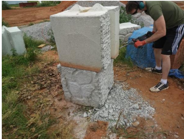
Figure 49. Removal of shear key and a thin layer of material from the side of a large concrete half-block before its installation in the GRS abutment model
