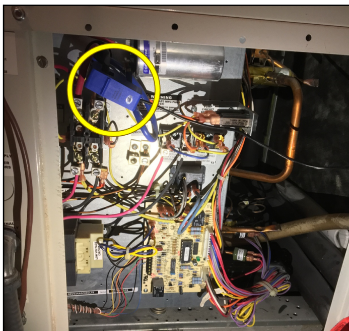
Figure 7.2: Picture of the current transducer clamped around the incoming electrical power cables inside the GSHP.
