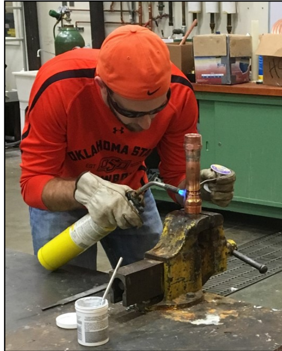
Figure 2.17: Soldering together threaded adapters to the end of a short pipe section.
