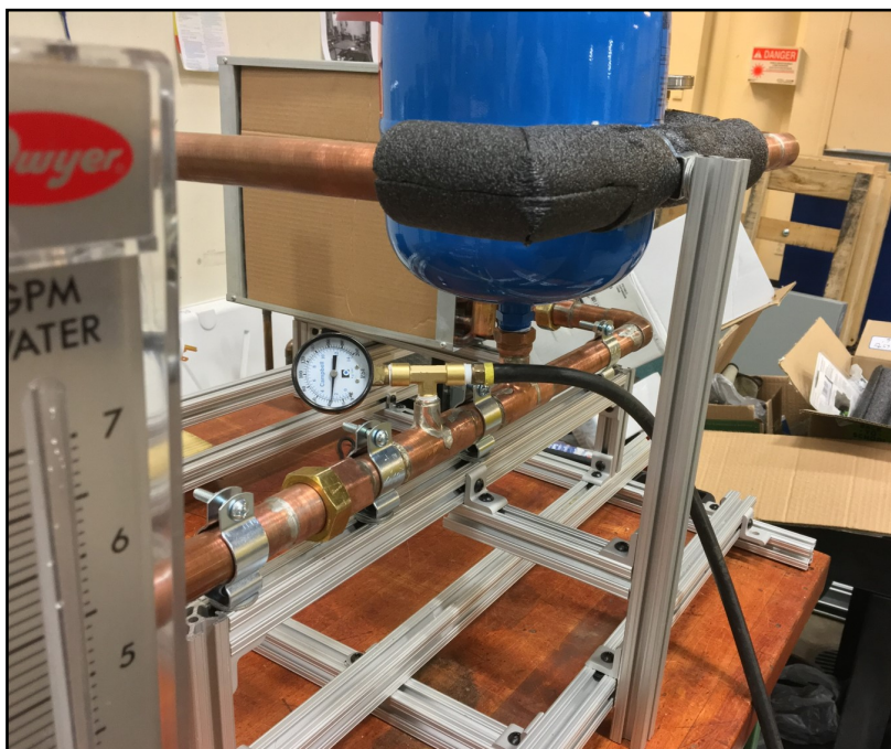
Figure 2.23: Close up of pressure gauge and air-compressor hose during initial pressurization of pressure test.
