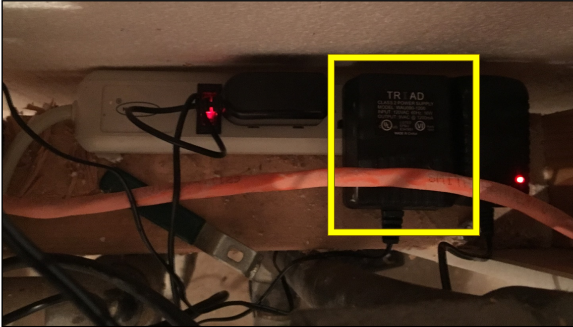
Figure 7.5: Picture of the voltage transformer plugged into the 120 V power strip, in order to measure the wall voltage.
