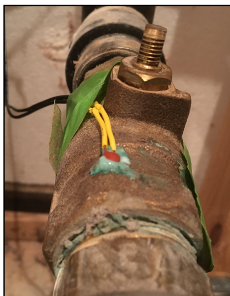
Figure 7.3: Picture of one of the thermistors measuring the on-pipe water temperature (with insulation removed).
