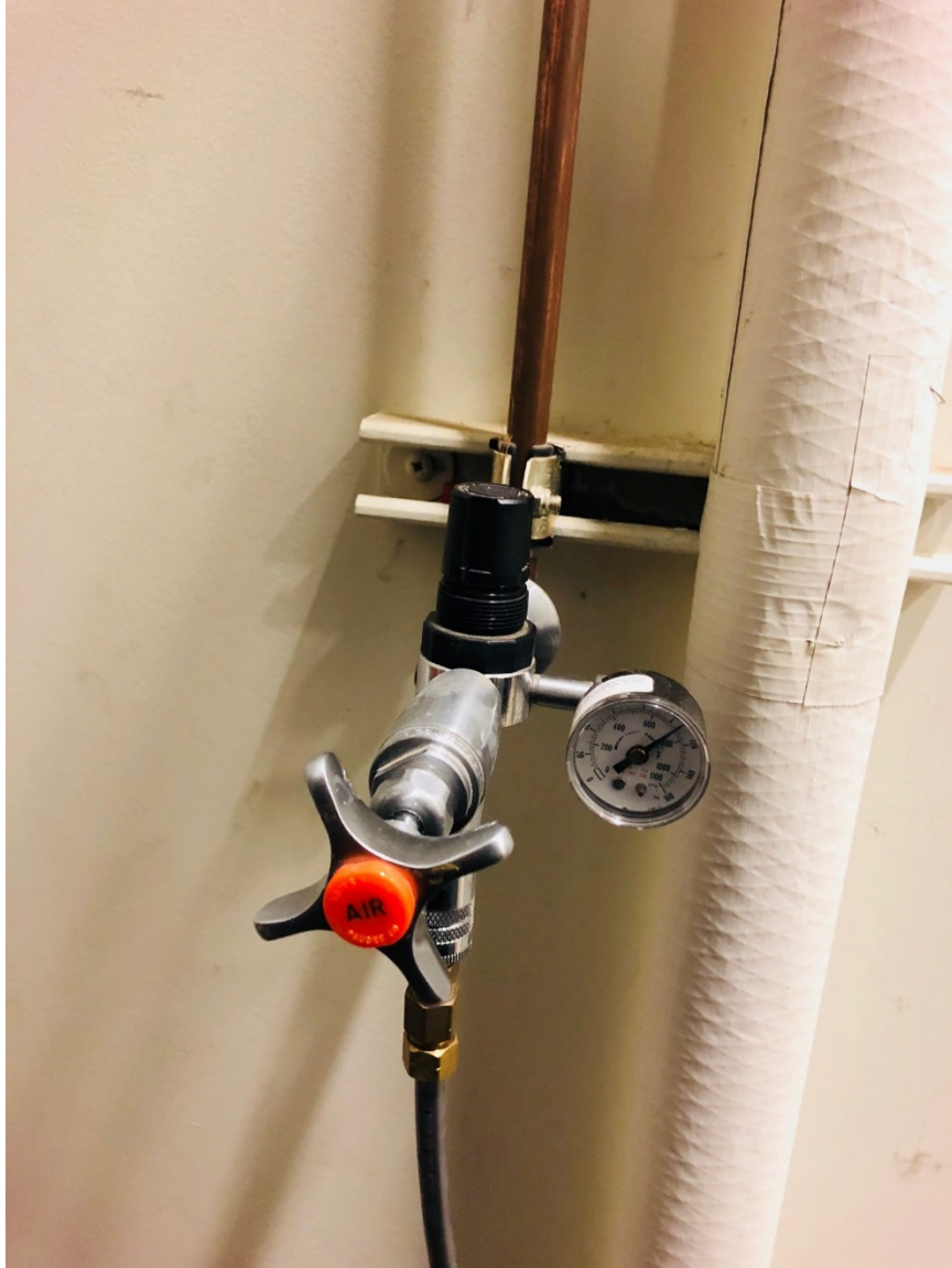
Figure 3.2a.8 – Pressure Control Valves (PCV-101) at Instrument Air Utility Supply Line.
