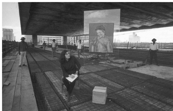
Fig. 3. Lina Bo Bardi with one of the glass and concrete supports on the second floor of MASP during construction.
