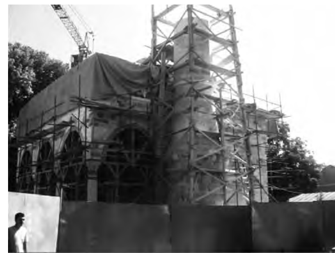
Fig. 1. The rising walls of the Ferhadija Mosque with the minaret under construction. (Photograph by author, August 2011)
